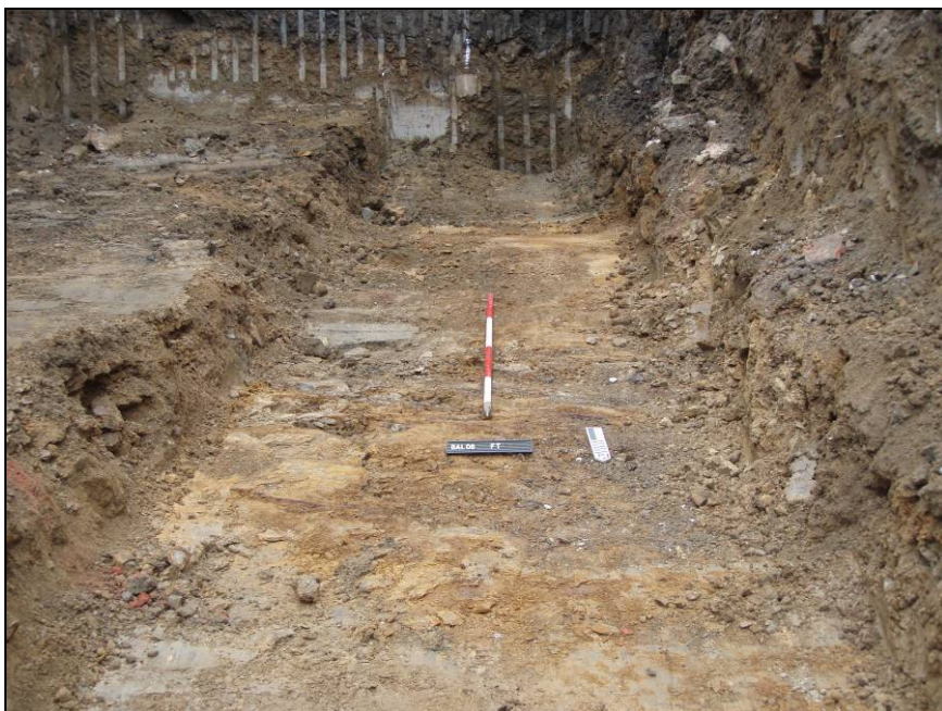
Fig. 6 Part of the foundation trench showing bedrock at the southwest side of the study area.
