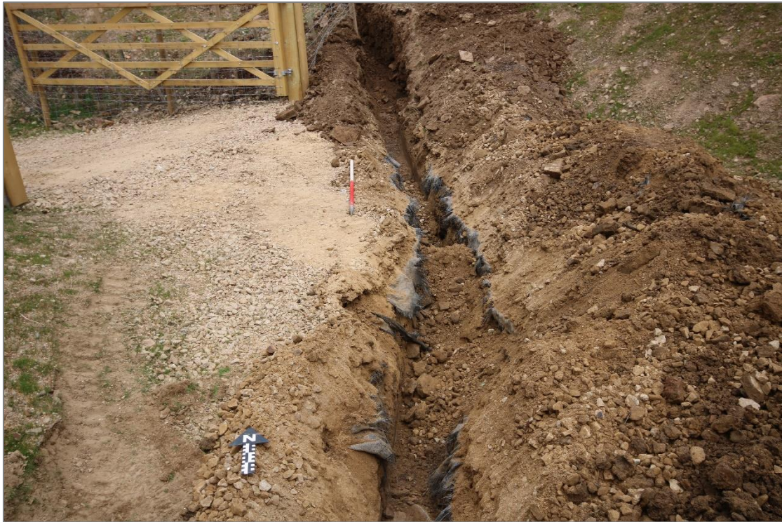
Figure 5: View north of excavated service trench showing hardcore deposit. Scale 1x1m in 0.5m graduations.
