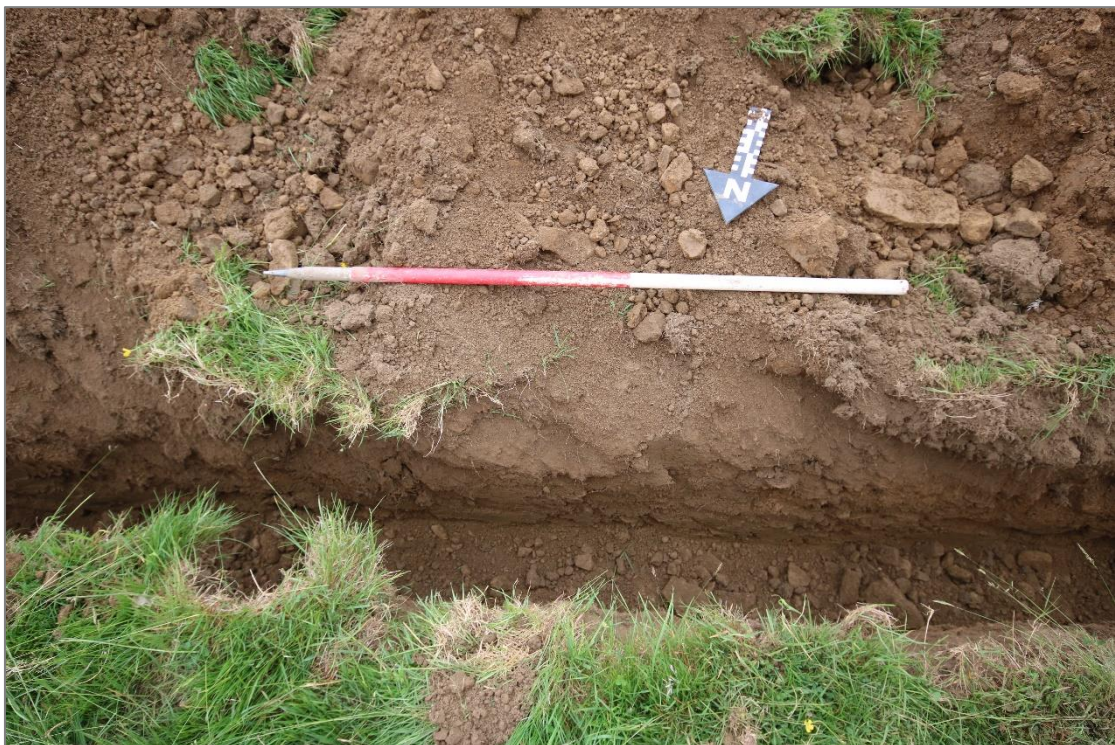
Figure 6: View south-east of representative section of excavated service trench. Scale 1x1m in 0.5m graduations.
