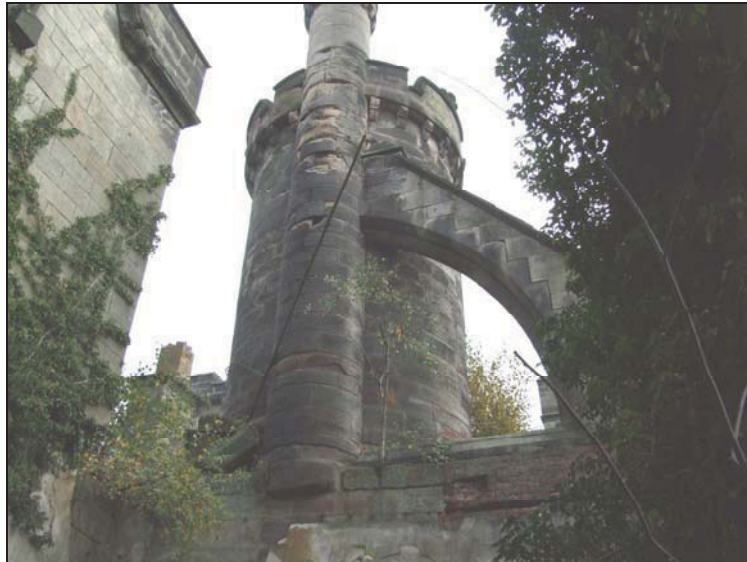
Fig. 13 Upper storeys of west elevation showing protruding chimney and flying buttress
