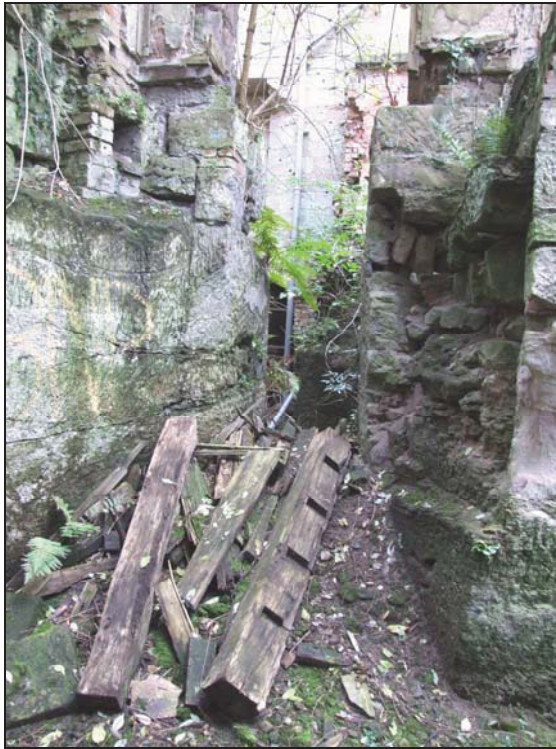
Fig. 8 Collapsed floor causing restricted access to north elevation
