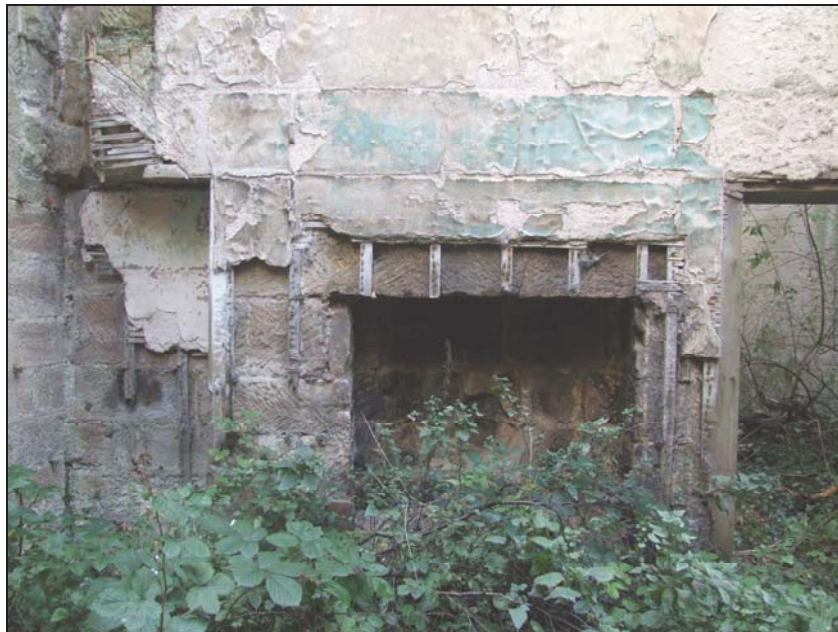
Fig. 11 Lower storey of west elevation showing fireplace, surviving plaster and turquoise paint
