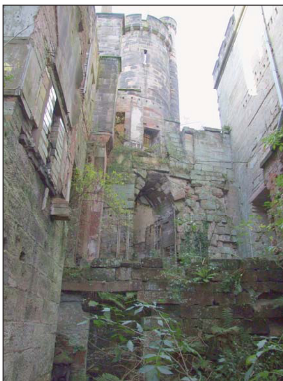
Fig. 2 Northern elevation of tower showing it's location within larger Alverton Lodge structure. Photograph taken from storey below that at which recording started and lower section obscured by wall in foreground at base of illustration.
