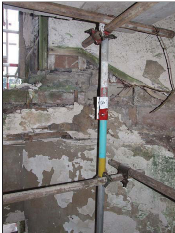
Fig. 15 Detail of the 'ghost' of the original interior spiral staircase showing the exposed brickwork behind the lath and plaster rendering.
