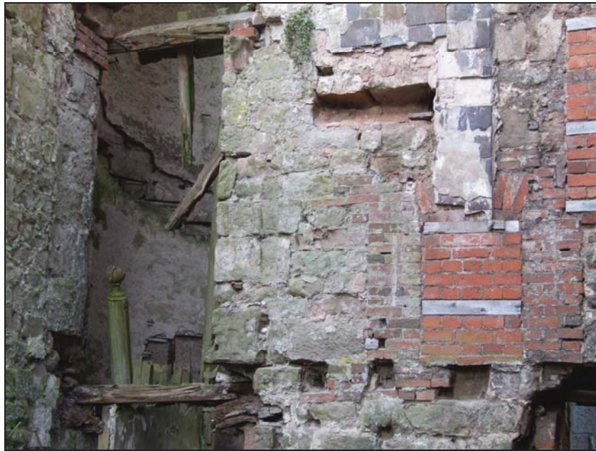
Fig. 5 Central storey of east elevation showing doorway to Round Tower and phases of brickwork infilling and remodelling
