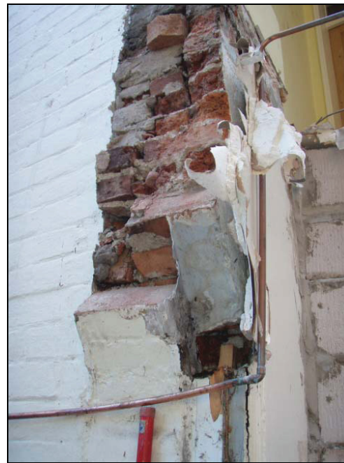
Fig. 4 Arch revealed after the demolition of the modern kitchen, utility and bedroom (facing south)
