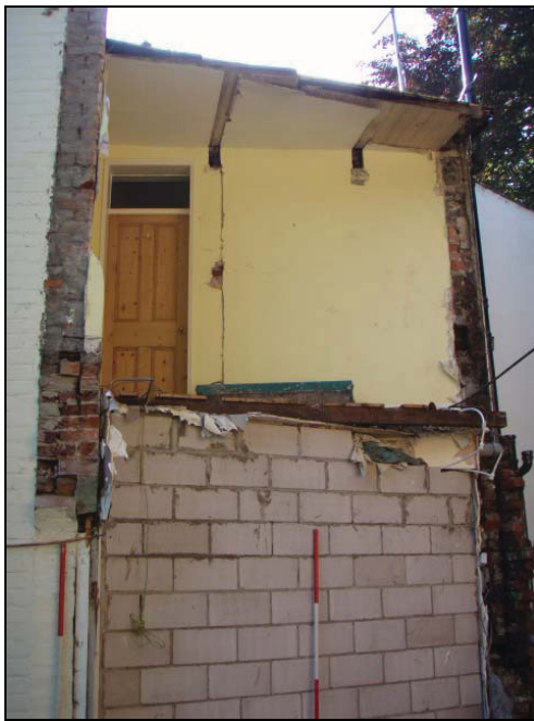
Fig. 3 Evidence of the demolished kitchen, utility room and bedroom (facing east)
