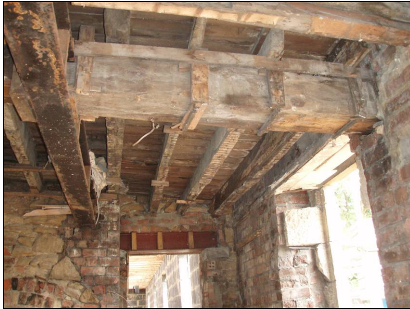
Fig. 3 Dangerous roof joists looking up from ground floor.
