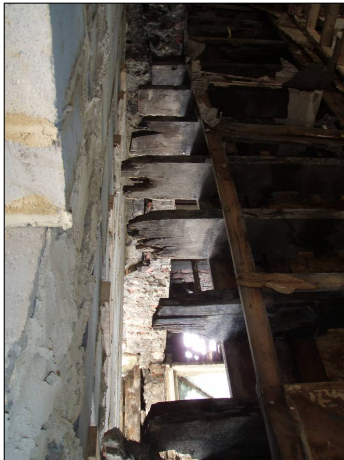
Fig. 2 Rotten joists, looking down from first floor
