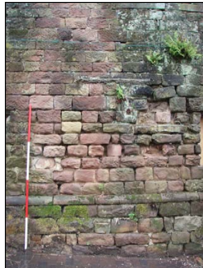
Fig. 29 Heavy erosion of the south-east wall of the extension to the farmhouse
