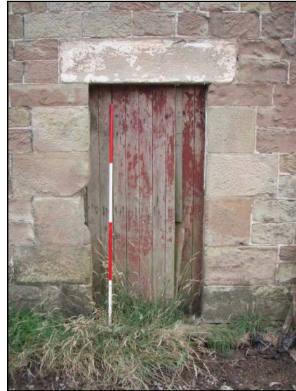
Fig. 10 Lintelled and jambmed door on ground floor of north-east elevation of the barn
