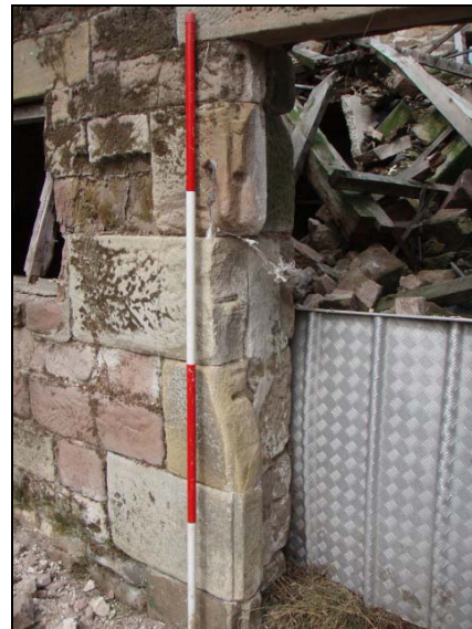
Fig. 15 Carved sandstone jamb of ground floor door in the south-west elevation of the barn
