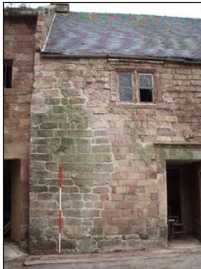
Fig. 28 Area of the north-west wall of the farmhouse extension which has undergone repair and upper window
