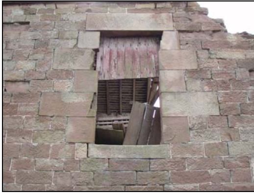
Fig. 9 Lintelled and jambmed door on upper floor of north-east elevation of the barn
