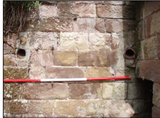
Fig. 17 Ventilation pipes within the south-west elevation of the barn
