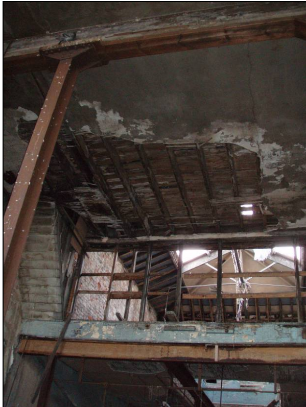
Fig. 25 Condition of first floor, floor support and ceilings 172/3
