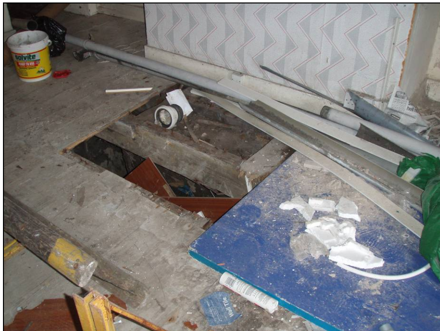
Fig. 30 Condition of ground floor boards 174/5
