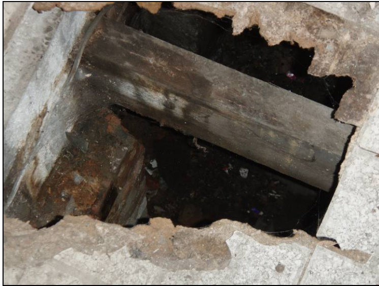
Fig. 19 Poor condition of flooring of 170/1
