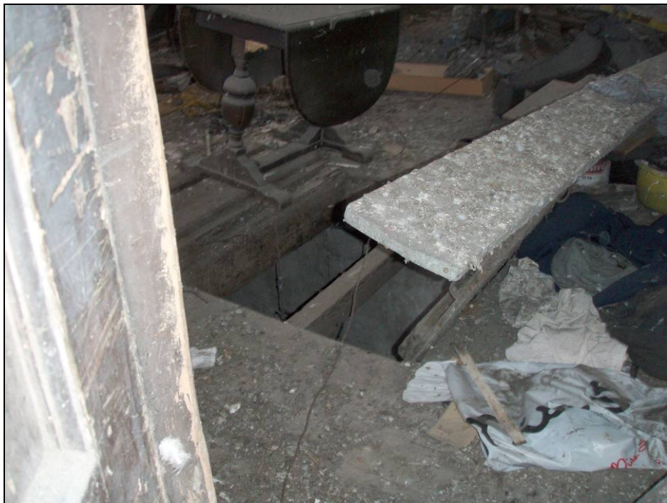
Fig. 26 Ground floor flooring and vermin contamination
