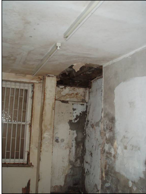
Fig. 31 Rotted ceiling joists 174/5
