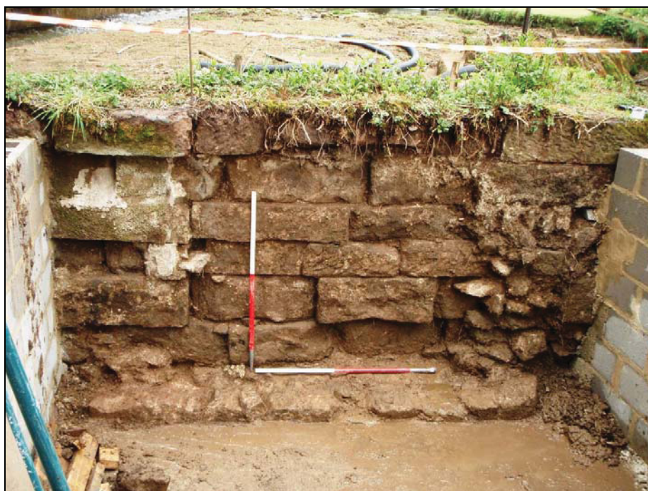
Fig. 15. North facing section of reservoir wall within the intake house. Scale 2 x 1m
