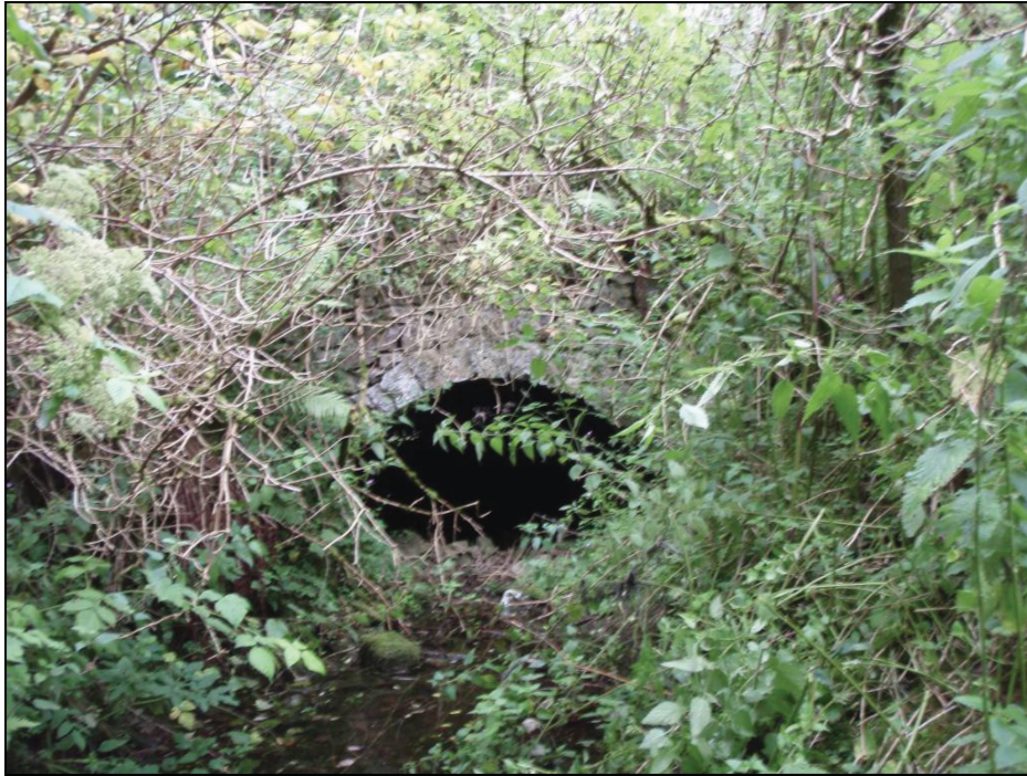
Fig.4 The stone built exit of the covered mill race prior to defoliation, facing south towards the mill.
