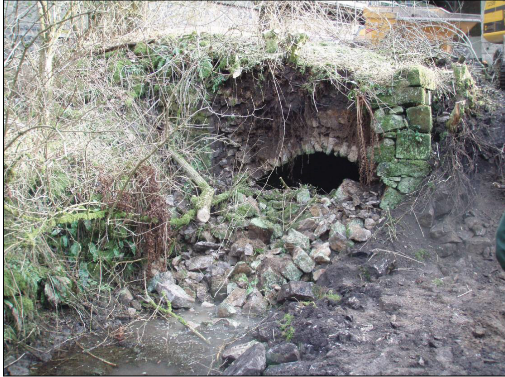
Fig. 7 Collapse of the mill race front showing evidence of extensive root penetration.
