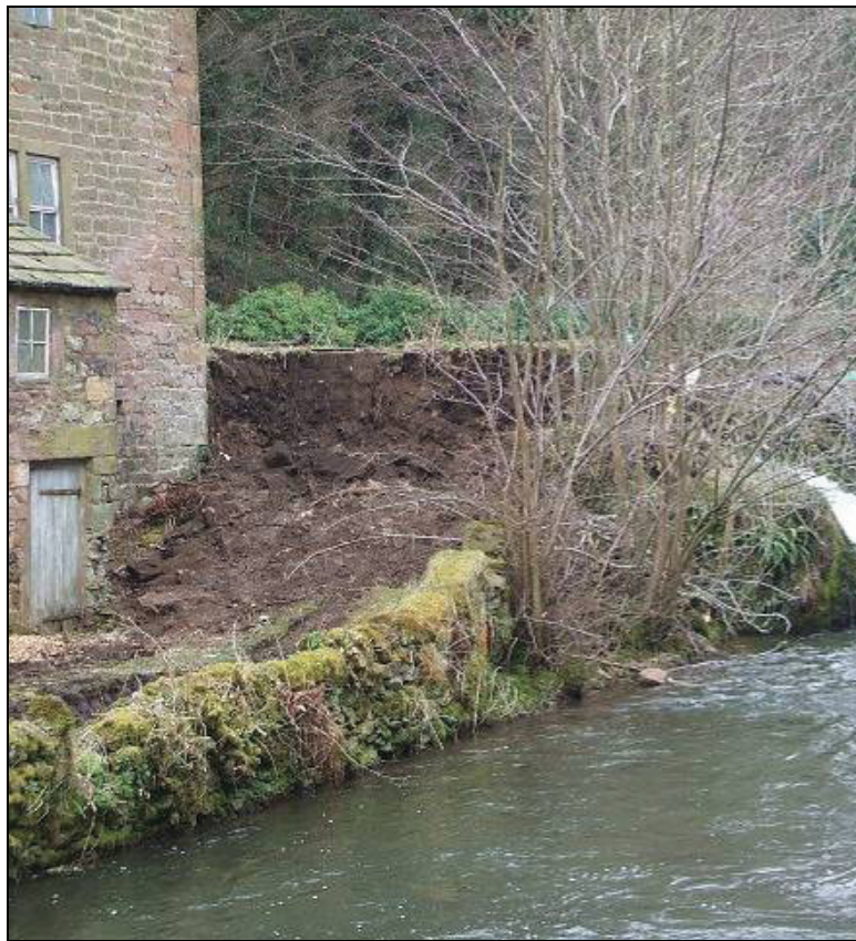
Fig. 12 Intake Tank area under excavation, facing south-west. Photograph supplied by Derwent Hydro Ltd.
