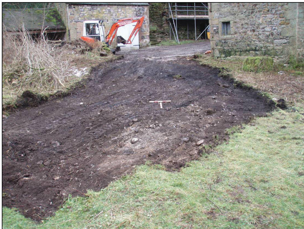
Fig. 3 Stripped area north of the mill to allow consolidation of access, facing east.
