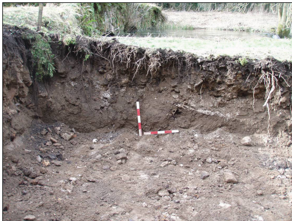
Fig. 6 The east facing section of the turbine pit before excavation of the sump.
