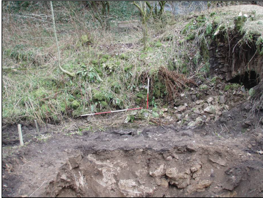
Fig. 8. A dilapidated section of the eastern mill race wall near the covered outlet, post collapse.
