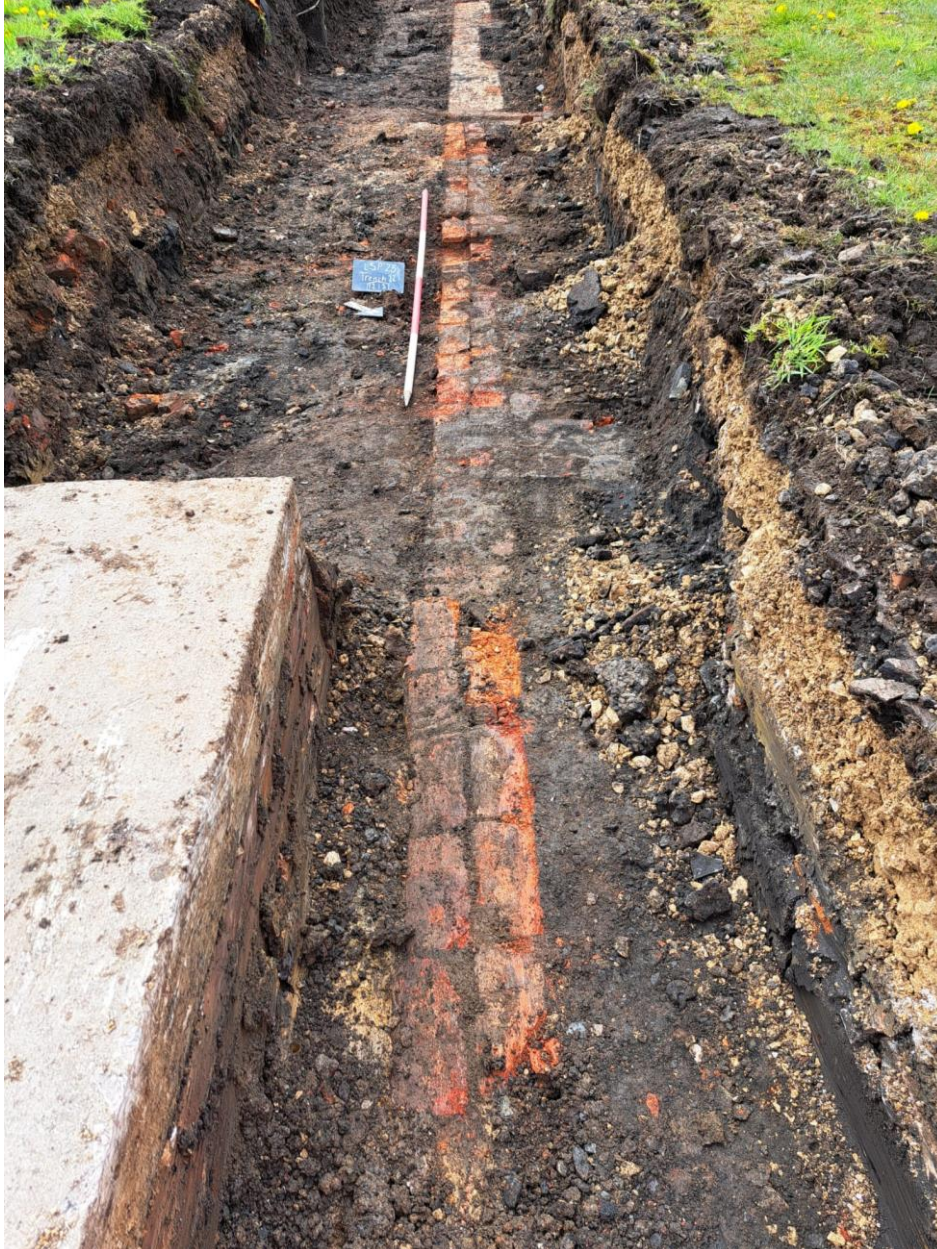
Figure 21: Photograph showing the eastern wall of the former refreshment rooms, looking south-west, with later wall {1213} in foreground, and earlier wall {1218} in background. Scale 1x2m in 0.5m graduations.
