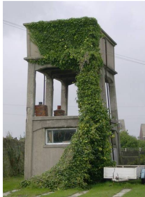
Figure 7.18 The water tower at Robert's Battery, a Grade II* Listed Building (author)
