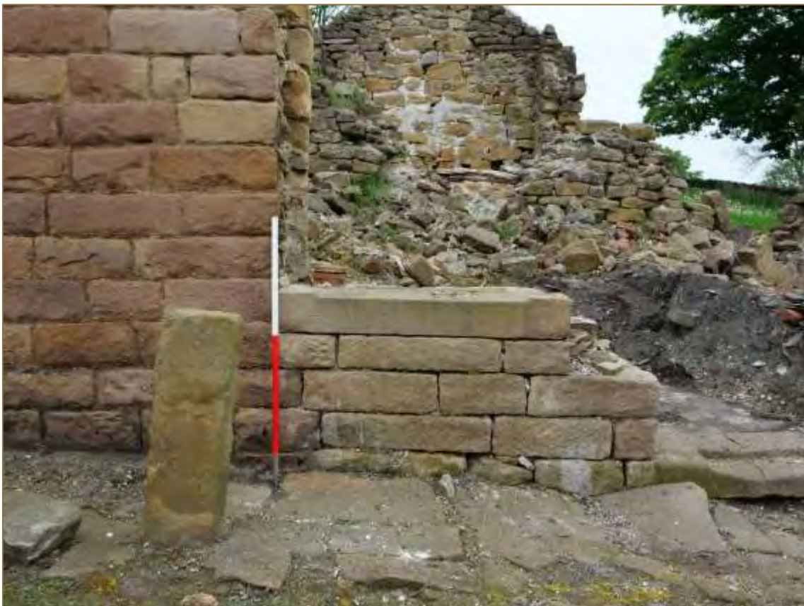
Photograph 10: The in-situ cill to the centre range aperture. Scale 1m. (File: HBR_112)
