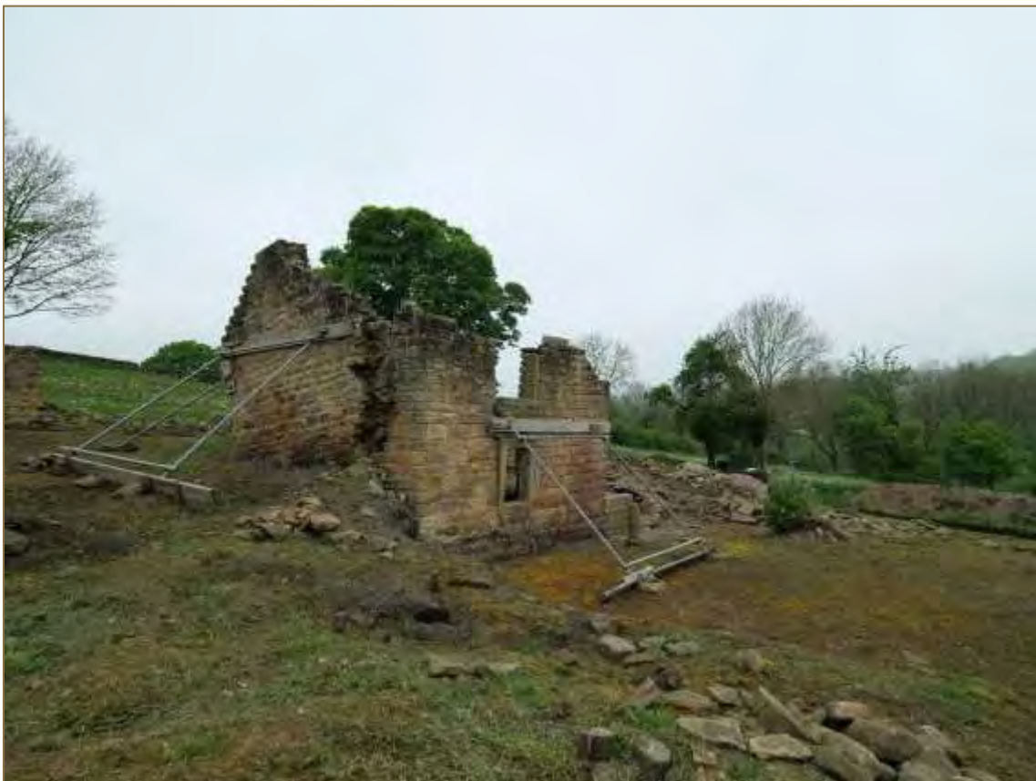
Photograph 5: Overall view of the remains of Hay Lane Cottage (looking north west). (File: HBR_9)
