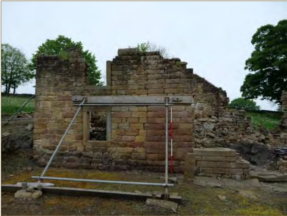
Photograph 7: The east elevation of the remains of Hay Lane Cottage (looking west) Scale 2m. (File: HBR_10)
