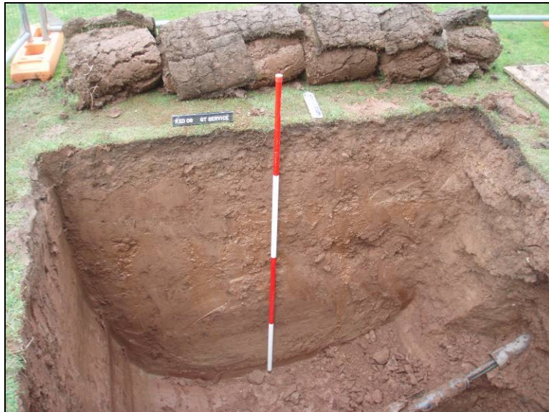
Fig. 16: View of the pit for the new grease trap, Scale: 2m (looking north).
