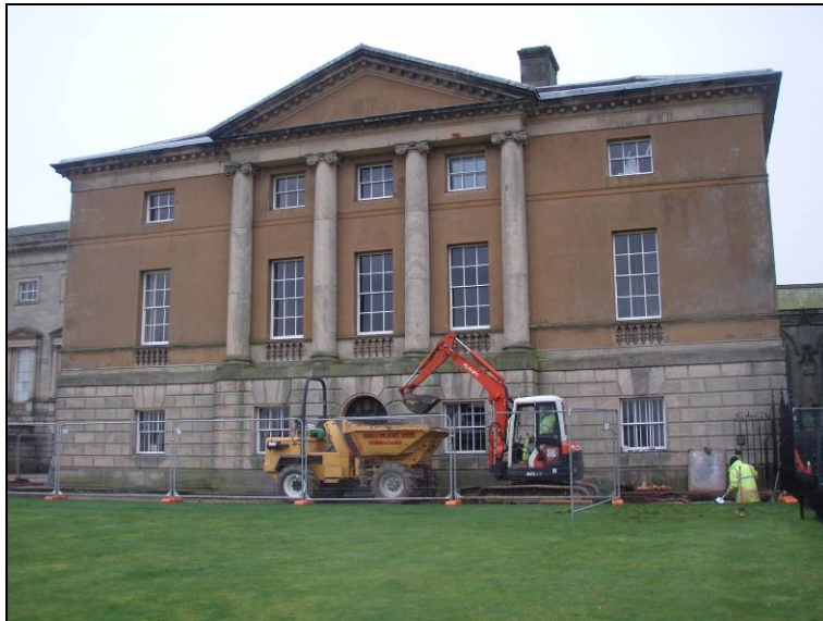
Fig. 15: View of the West Wing showing work to remove the grease trap underway.
