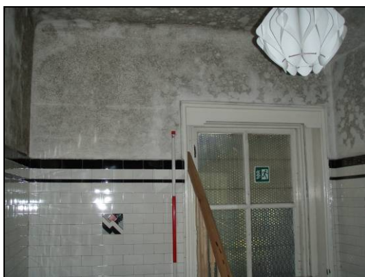
Fig. 47 Water damage to Room 13.
