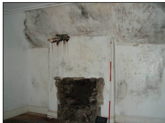
Fig. 44 Damaged chimney breast in Room 10
