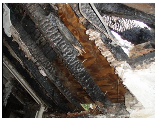
Fig. 38 Fire damage to roof of Stable Block
