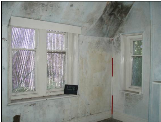
Fig. 41 Sash windows and water damage to Room 8.
