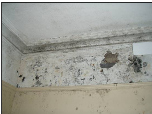
Fig. 35 Ceiling coving and rot in Room 4
