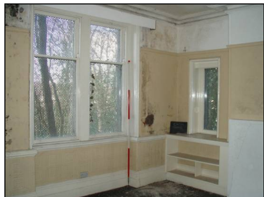
Fig. 34 Sash window and wall rot in Room 4.
