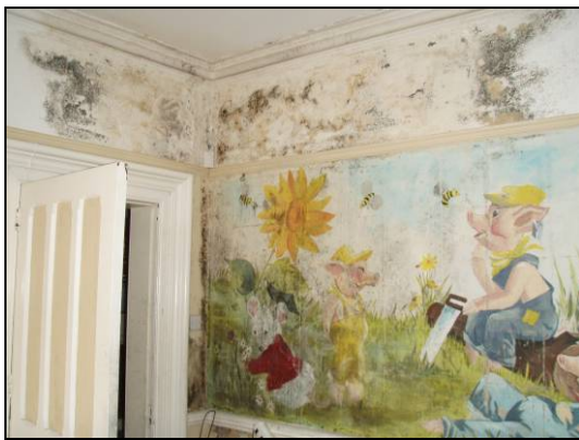
Fig. 31 Damp in Room 2.
