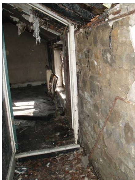
Fig. 37 Poor condition of Stable Block
