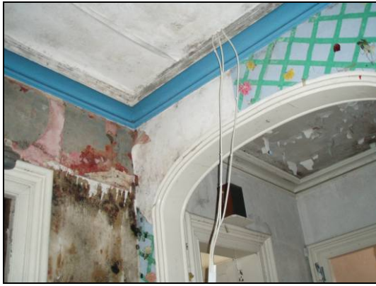
Fig. 29 Room 1, damage to ceiling.
