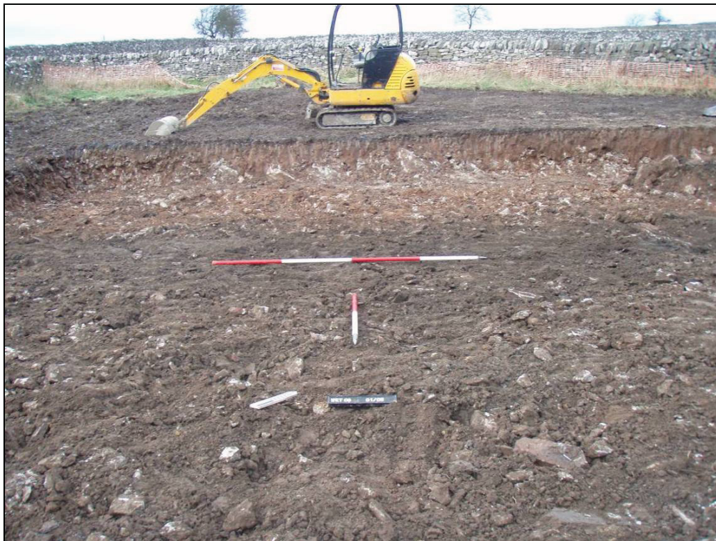
Fig 3 – Photo looking north showing the basic site sequence of shallow topsoil (001), underlying made-ground (002), natural clay (003), limestone bedrock (004) and the modern subsoil containing inclusions of limestone pieces (005) covering the south of the site in the foreground. Scale: 1 x 1m & 1 x 2m.
