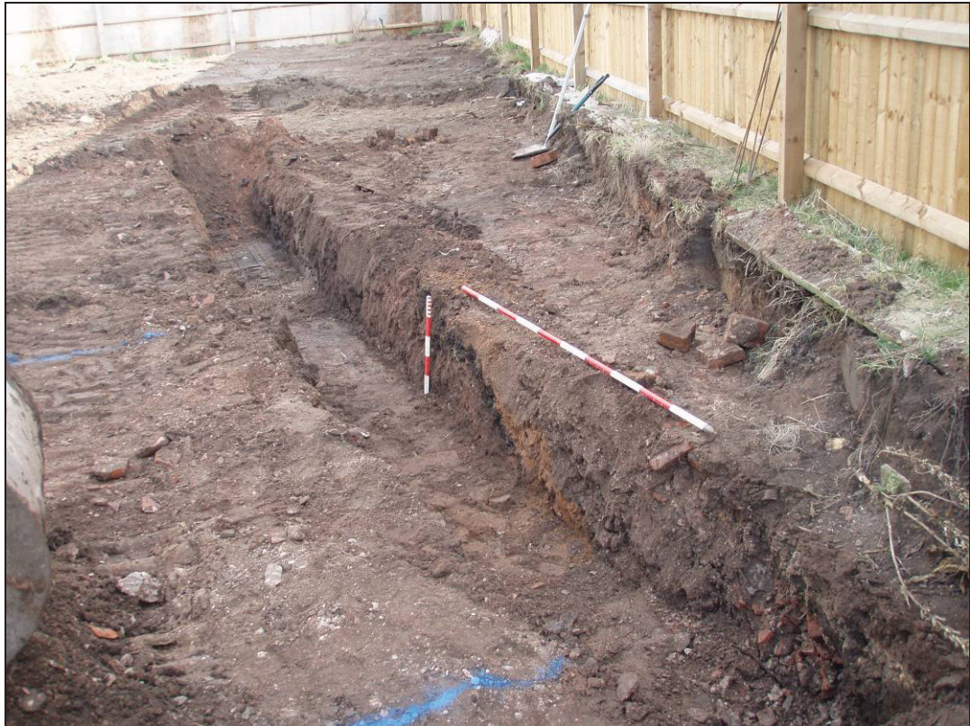
Figure 4. Oblique section of the most easterly foundation trench after initial ground reduction. Facing north.
