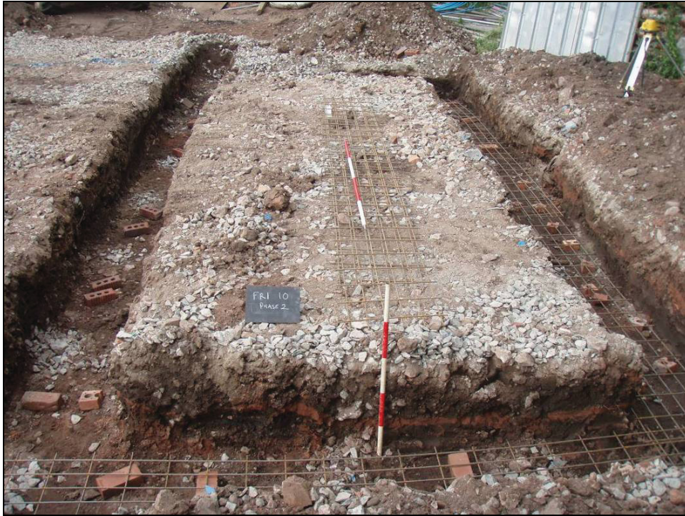
Fig. 3: Excavated area at the western extent of the site. Facing south. Scale 1m & 2m.
