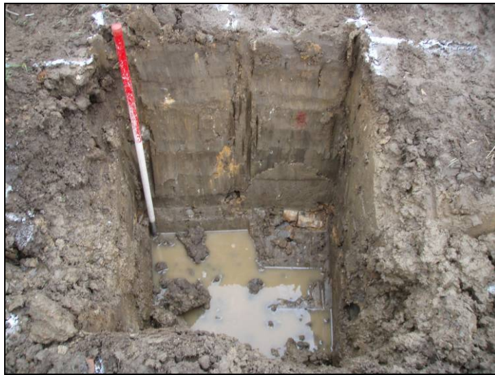
Fig. 3 A test pit to the west of the site with topsoil removed.
