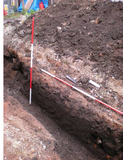
Excavation of foundation trench for new extension showing considerable post medieval disturbance.
