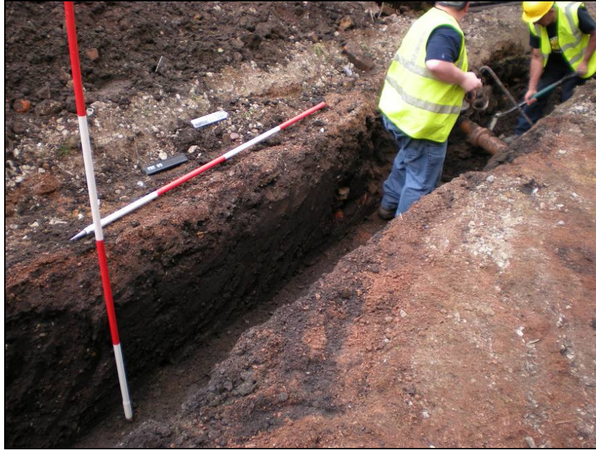
Fig 5. Excavation around pipes by hand, also showing level of post medieval disturbance
