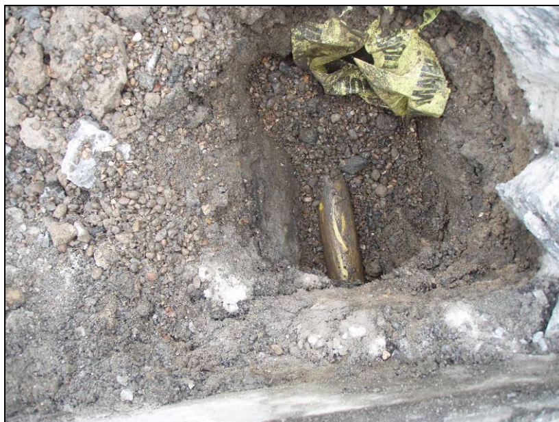
Fig. 4 Gas pipe sitting on made ground.
