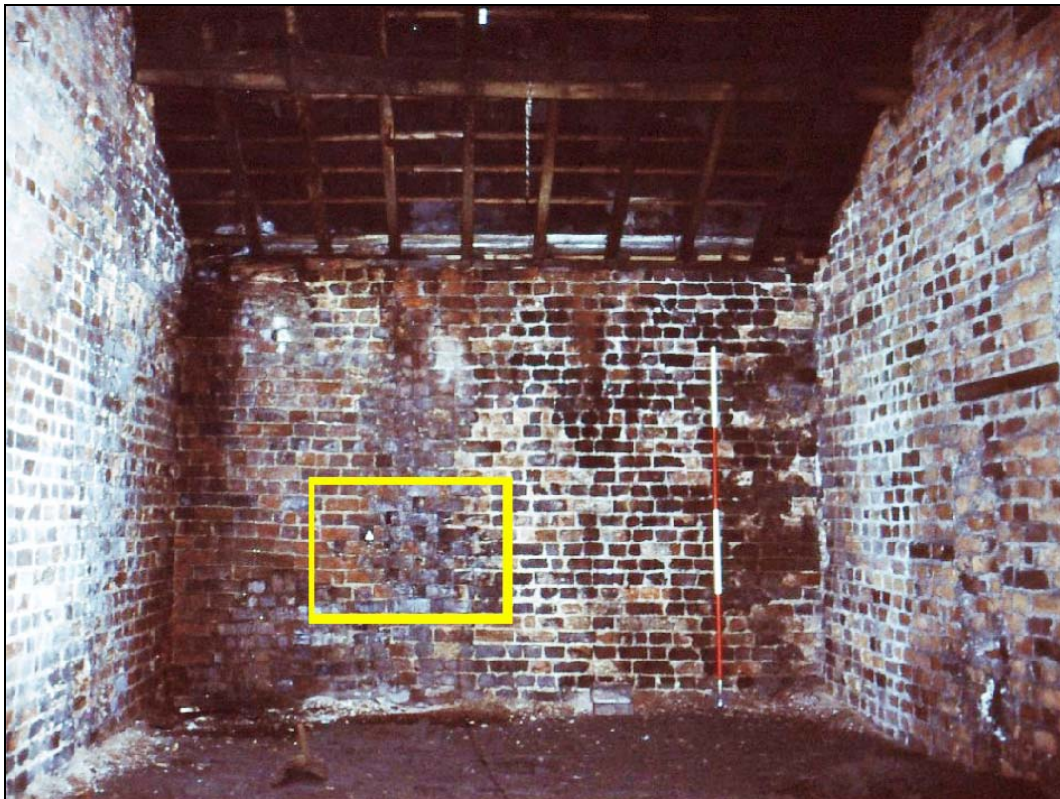
Figure 45: West wall of the original Barn with surviving honeycomb ventilators shown within the yellow box
