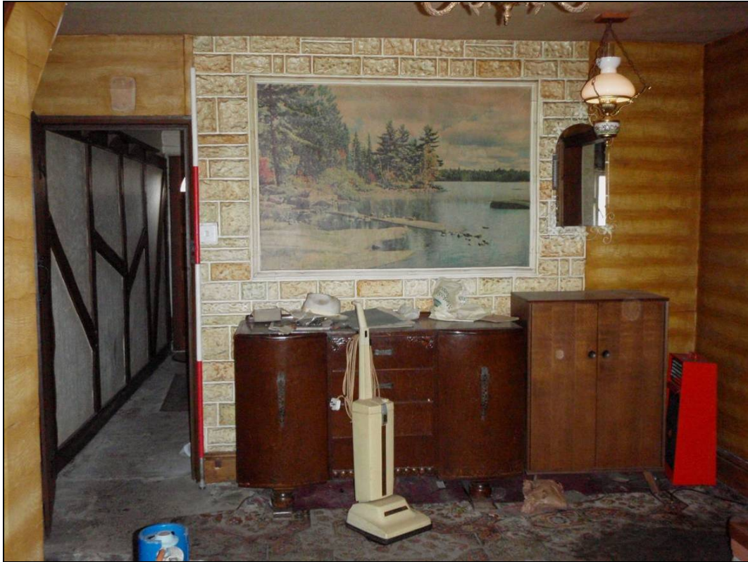
Figure 13: View of the partition wall between the Sitting Room and the Parlour
