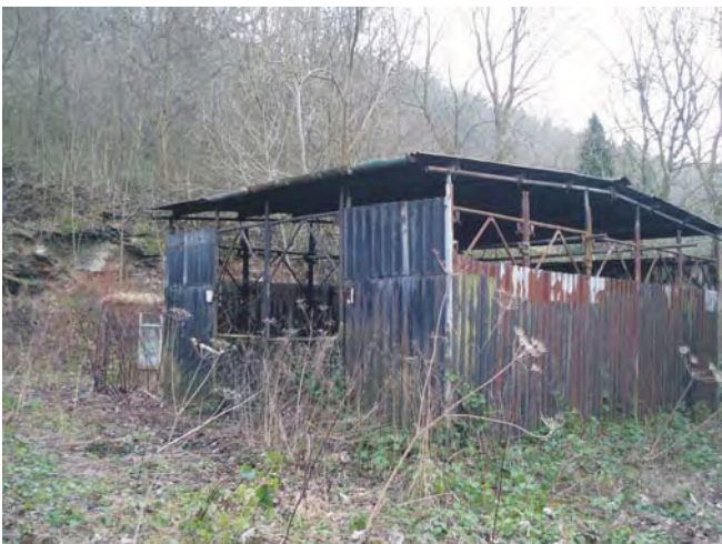
Figure 15: Looking south towards the main structure situated within the base of the former quarry
