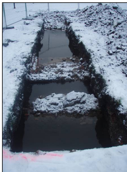
Fig. 7 Trench 2 flooded with central sewage pipe
