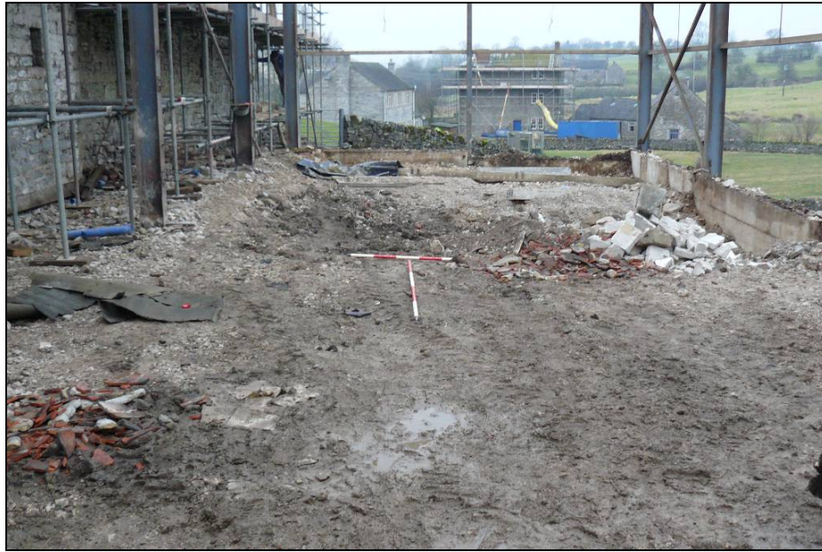
Fig. 8: Trench 3 swimming pool area prior to excavation. Facing west: Scale 1m & 2m
