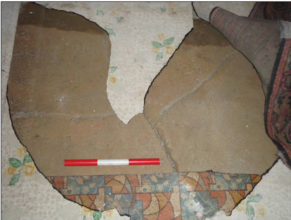
Figure 61: Fissures on the screed floor (scale 300mm)
