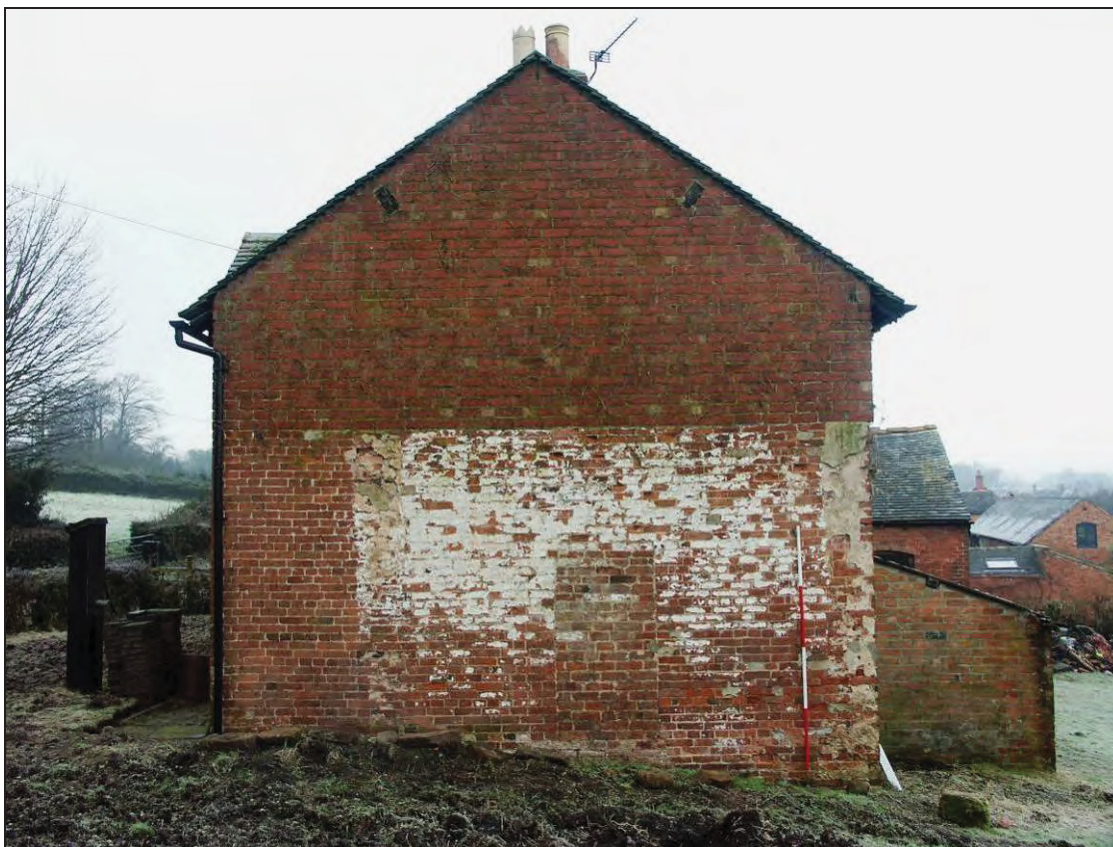
Figure 20: South elevation showing a blocked doorway and scars of a demolished structure (scale 2m)
