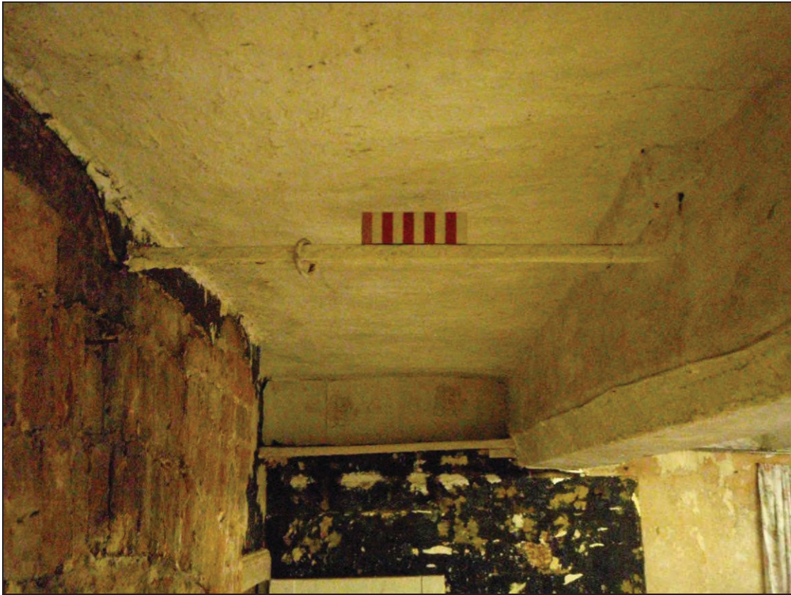
Figure 38: Iron rod with ring over the arched head of a former kitchen range (scale 100mm)
