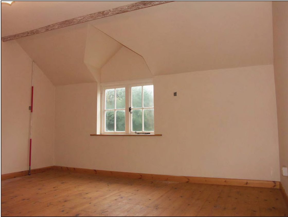
Figure 53: General view of room F-1 with new plaster board walls and floor boards (scale 2m)
