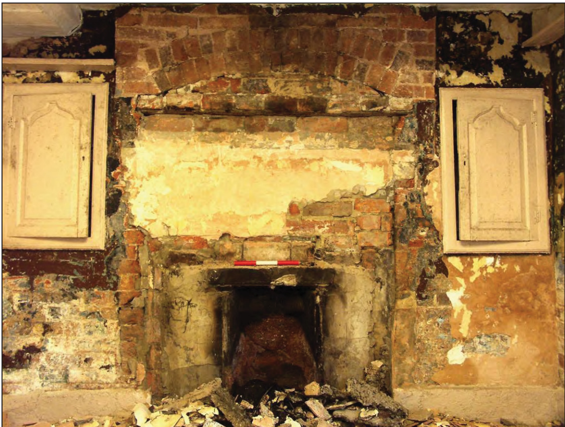
Figure 37: Detail of the fire place inserted in a larger blocked-up opening of a kitchen range (scale 300mm)
