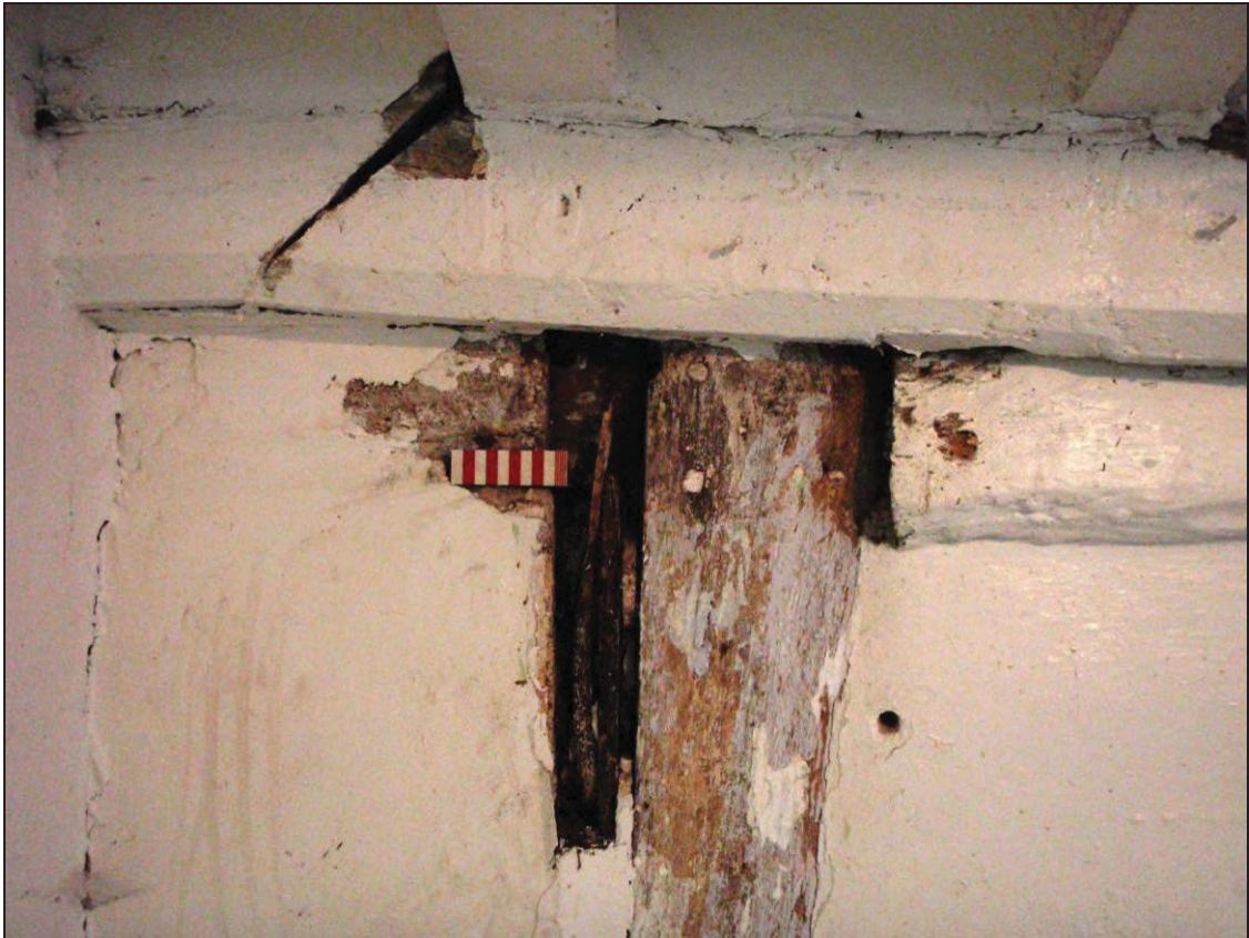
Figure 30: Detail of stud detached from rail with later cement infill, looking south (scale 100mm)
