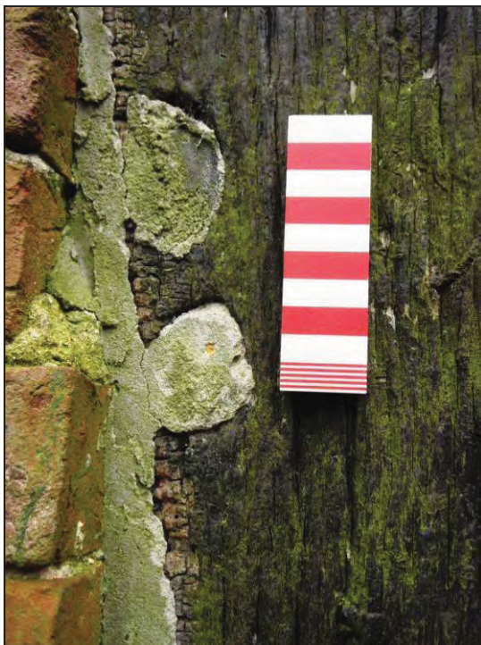
Figure 5: Detail of removed pegs (scale 100mm)
