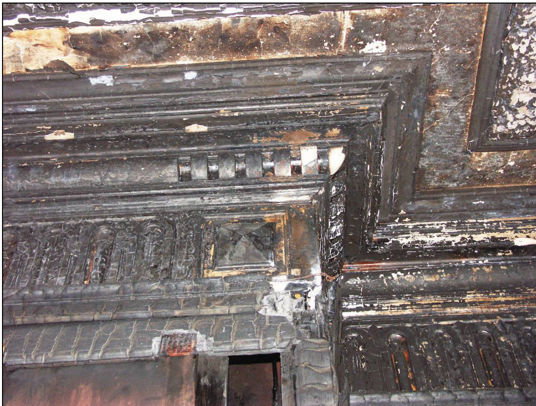
Fig. 32 Detail of plaster frieze and cornice with severe burn damage
