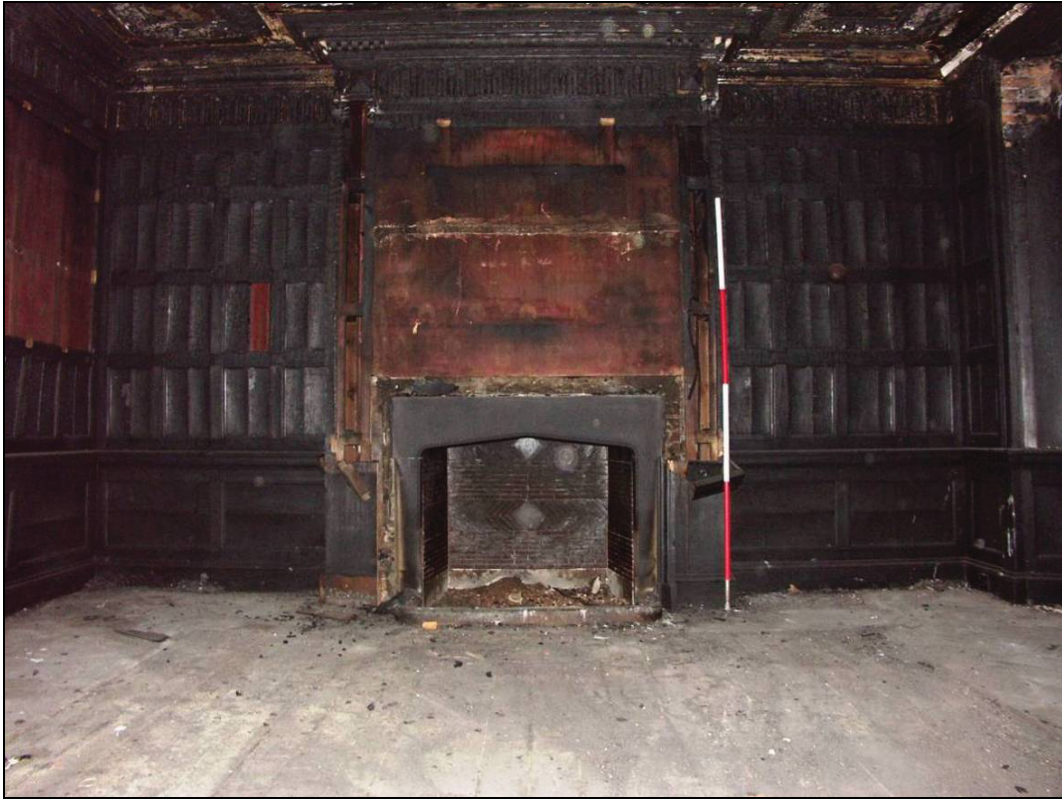
Fig. 30 Fireplace and burnt wall panelling in the south-western main room
