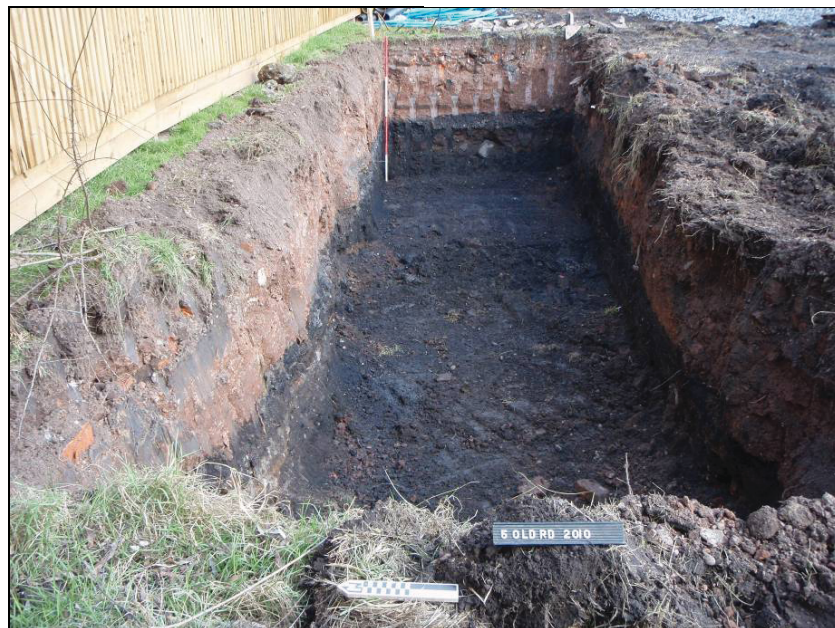
Fig. 9: Post excavation of soakaway 4, made ground of clay/rubble and fly ash. Facing East, Scale 2m
