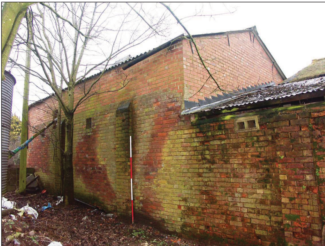
Plate 2: South elevation of Building A incorporating an earlier brick wall with pilasters
