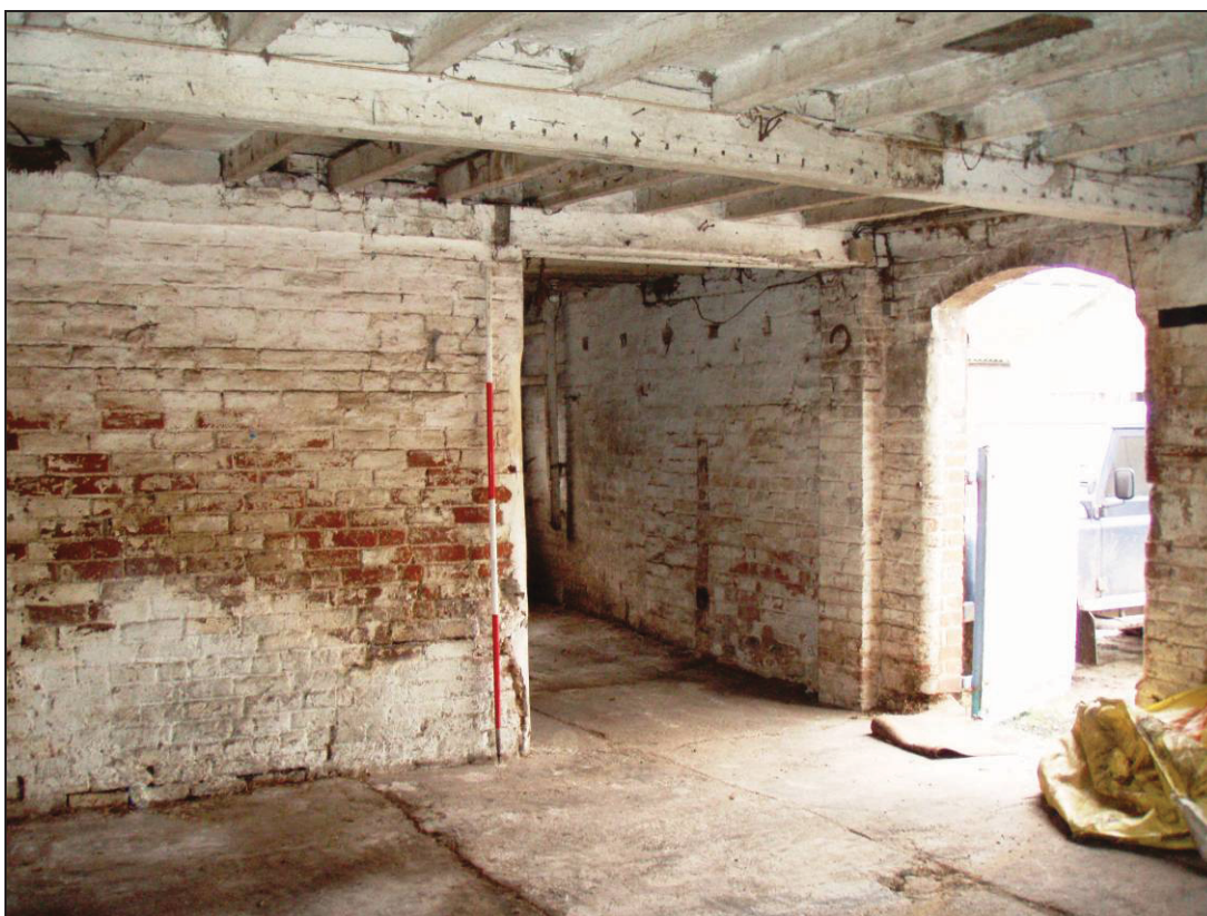
Plate 47: Internal view of the main central room on the ground floor of Building K
