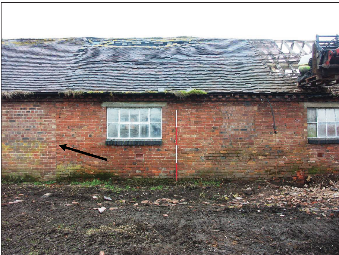
Plate 21: Construction break on the east elevation of building E, indicated with an arrow
