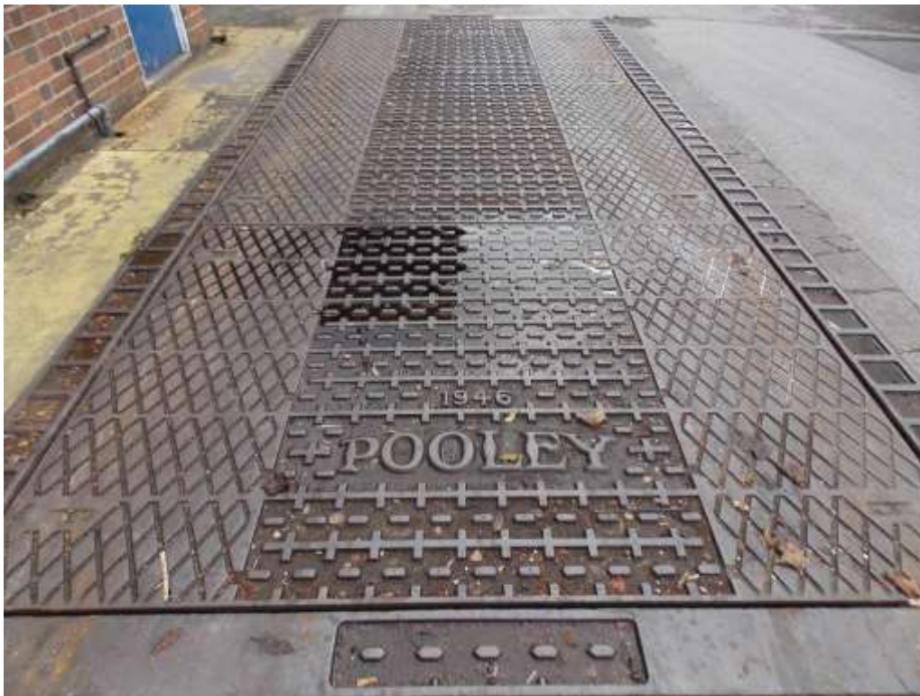
Figure 83: Detail of weighing bridge adjacent to the gate house of Building K.
