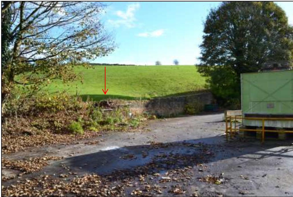
Figure 29: View north-east of part of the eastern boundary of the PDA. The wall itself is brick, which was once faced, and topped with several courses of stone. A cast-iron bearing housing is built into this wall, though it is currently overgrown with vegetation (red arrow).
