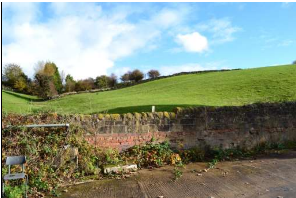
Figure 30: View west of the brick and stone boundary wall, and the undulating landscape beyond.
