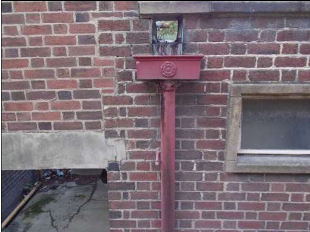
Figure 90: Detail of the construction joint between Buildings L and M and cast-iron hopper.
