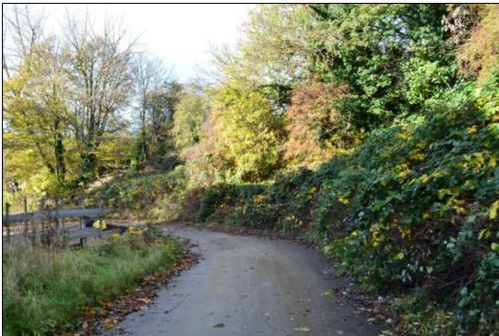
Figure 28: View of the northern boundary of the PDA. A retaining wall, following the access road, lines the majority of this boundary, which is overgrown with thick vegetation.
