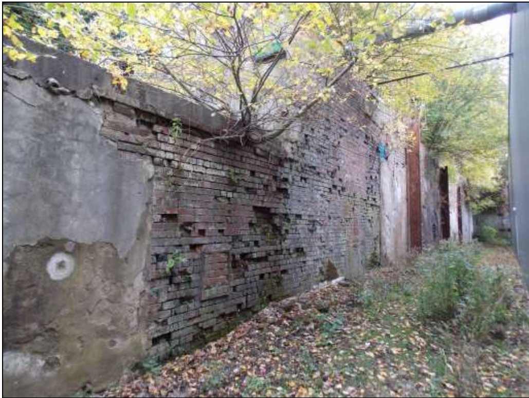
Figure 31: View south-east along the eastern border of Building D. This deep area potentially represents the footprint of the original Park Foundry building.
