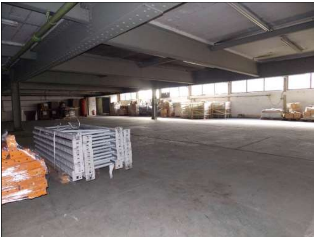
Figure 86: Southern area of Building K leading to the south cross-wing with curved wall.
