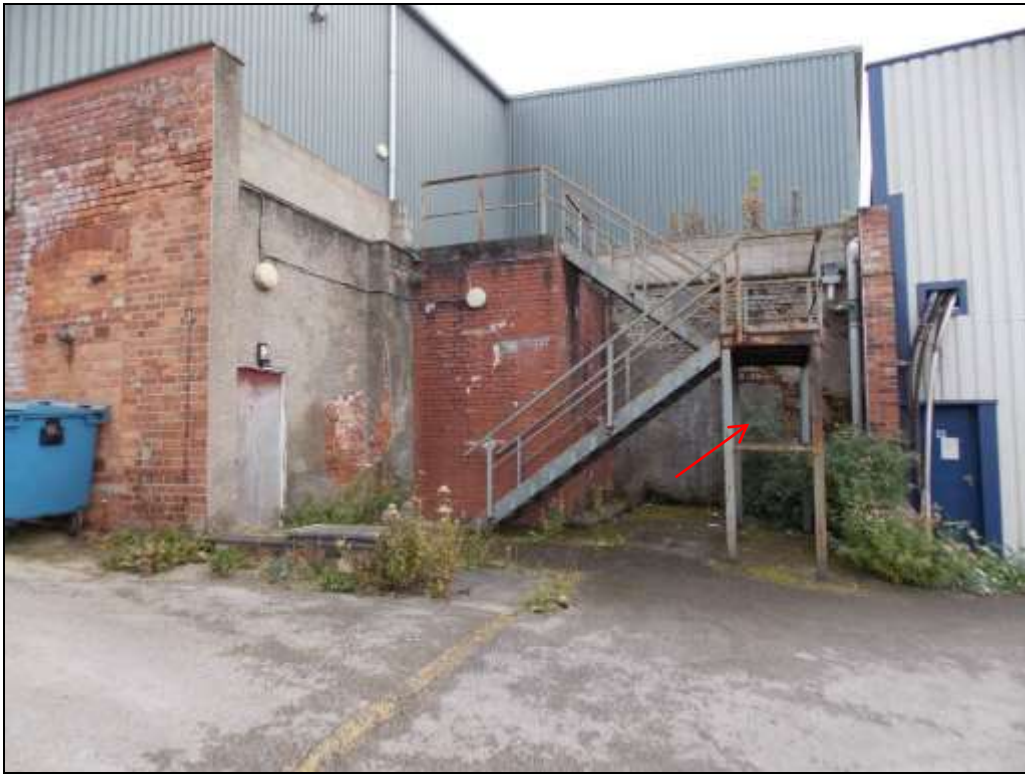
Figure 55: Chamfer plinth along the north elevation and blocked-up opening within an internal wall (arrow).
