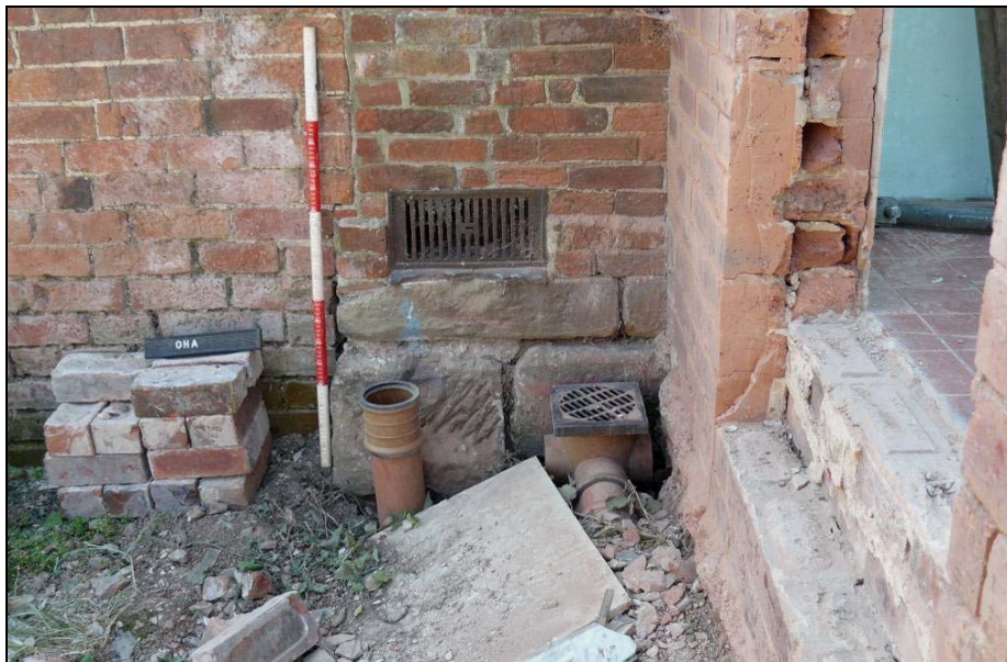
Fig. 3: Sandstone plinth at the south-east corner of Old Hall Farm. Facing west. Scale 1m
