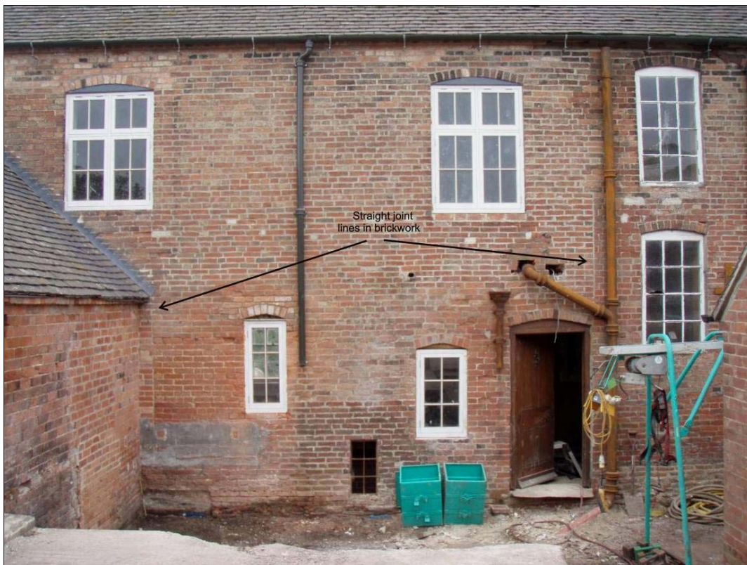
Fig. 14: Straight joint lines in the brickwork of the north elevation.
