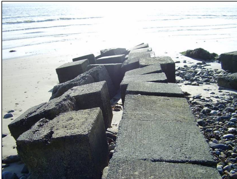
Fig 5.9.10 Anti-tank blocks used as part of the outflow of the Bondicarr Burn.
