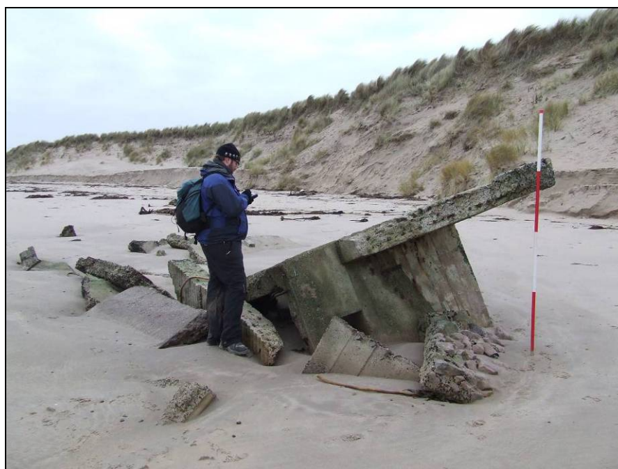
Fig. 7.25 Rapid recording of an eroding pillbox at Warkworth in Northumberland.
