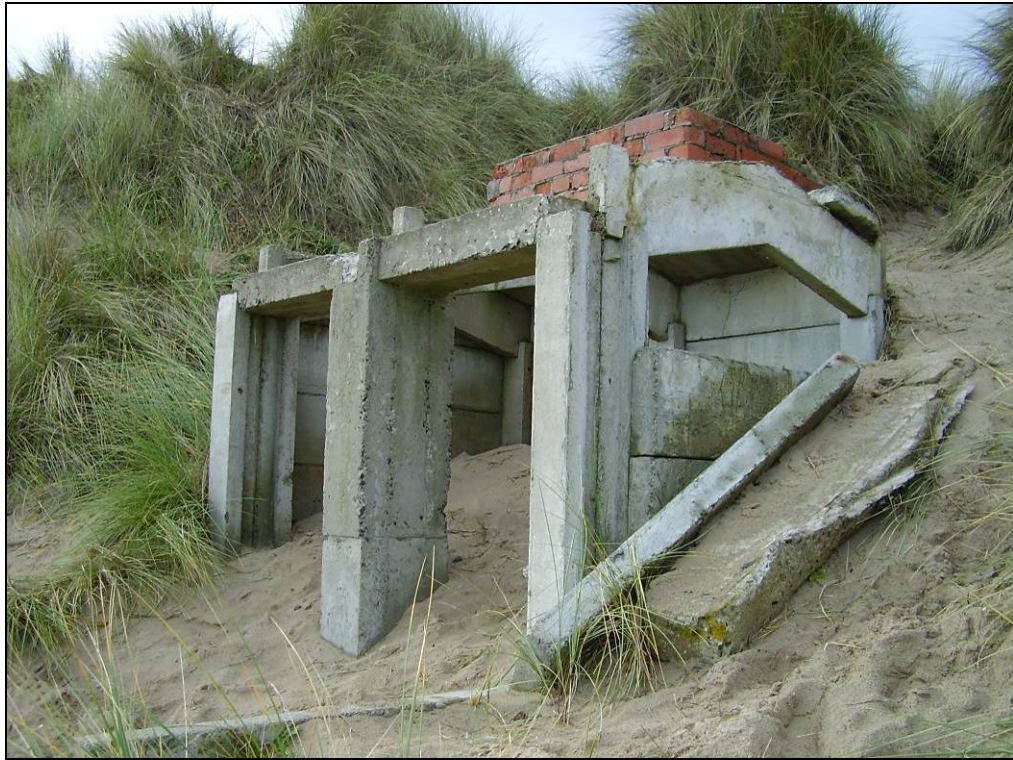
Fig 5.8.16 eroding military structure.
