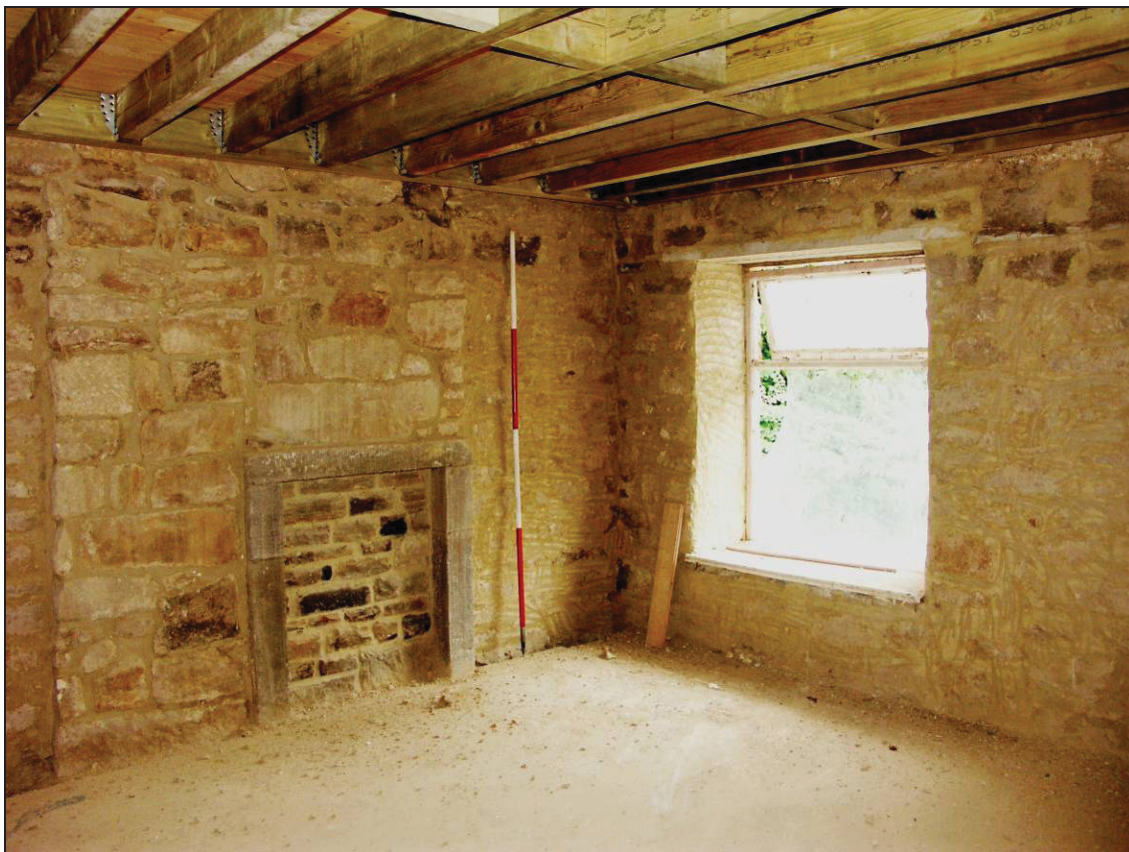
Figure 21: Blocked fire place in room F-3, looking west (scale 2m)
