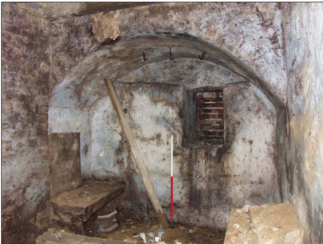
Figure 10: General view of the cellar with former coal chute blocked up, looking south (scale 1m)
