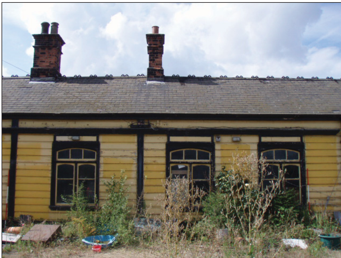
Figure 11: View of the third, fourth and fifth bay (from the south) of the east elevation
