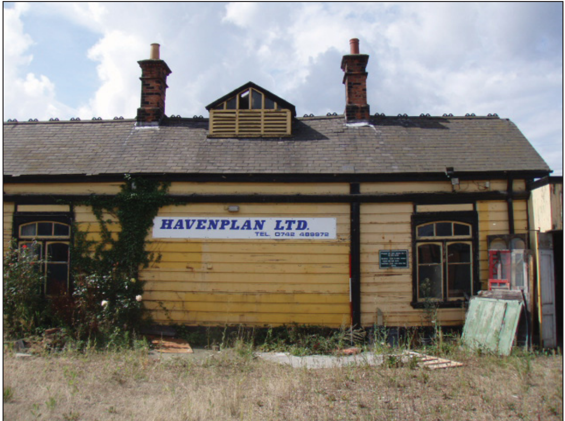
Figure 13: Northern end of the east elevation showing chimney stacks and louvre lantern
