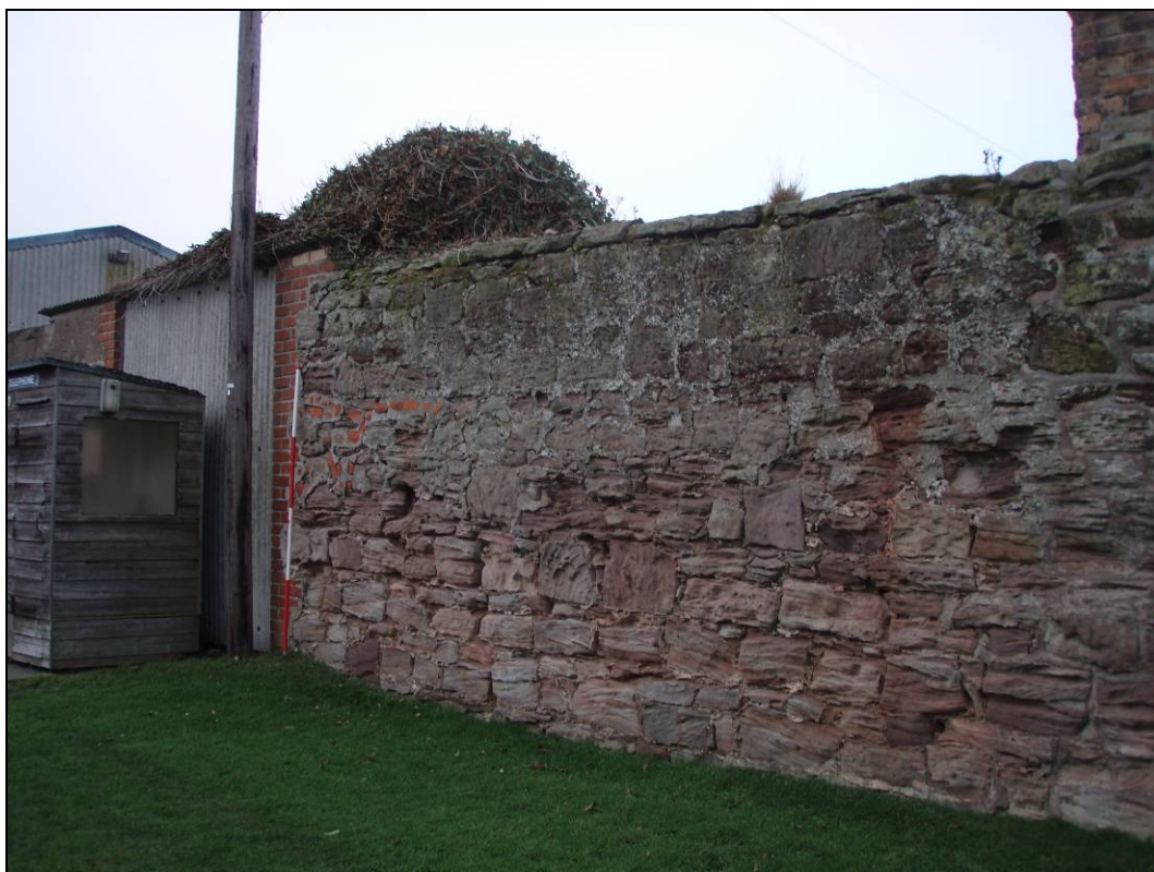
Figure 15. Wall 2 southeast facing elevation, showing heavy erosion.
