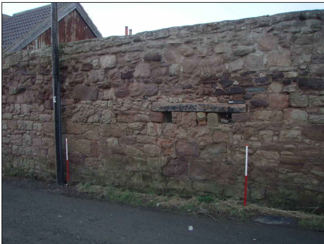
Figure 9. Wall 1 northwest facing elevation, with blocked off opening and utility holes
