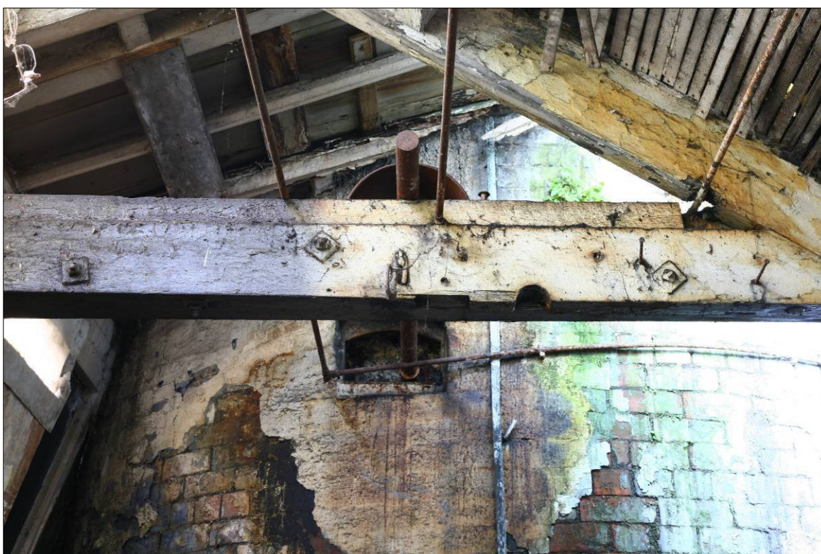
Figure 59. Location of the surviving pulley on the east wall and its bearing box set into the chimney stack.
