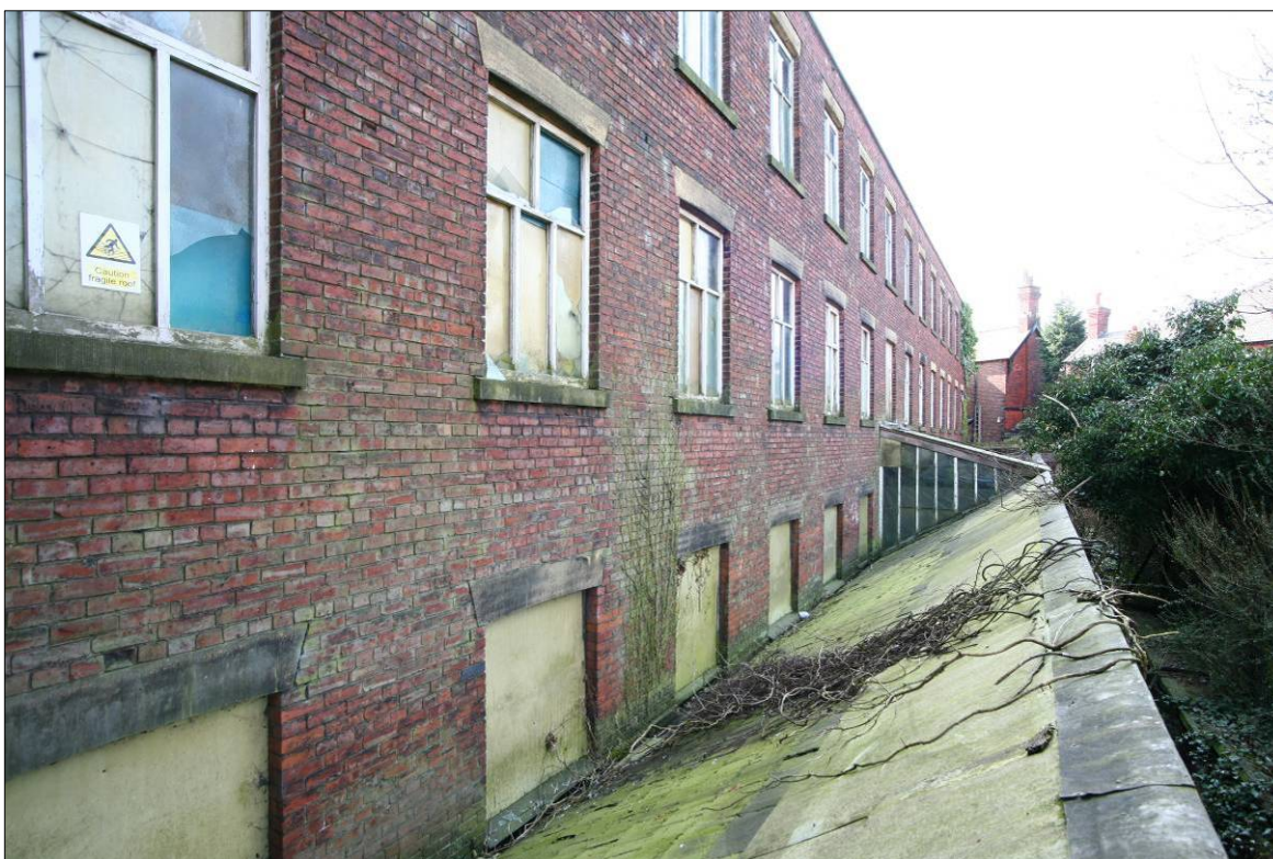
Figure 27. View along the north elevation, showing the top of the north-light roof of the single-storey extension.
