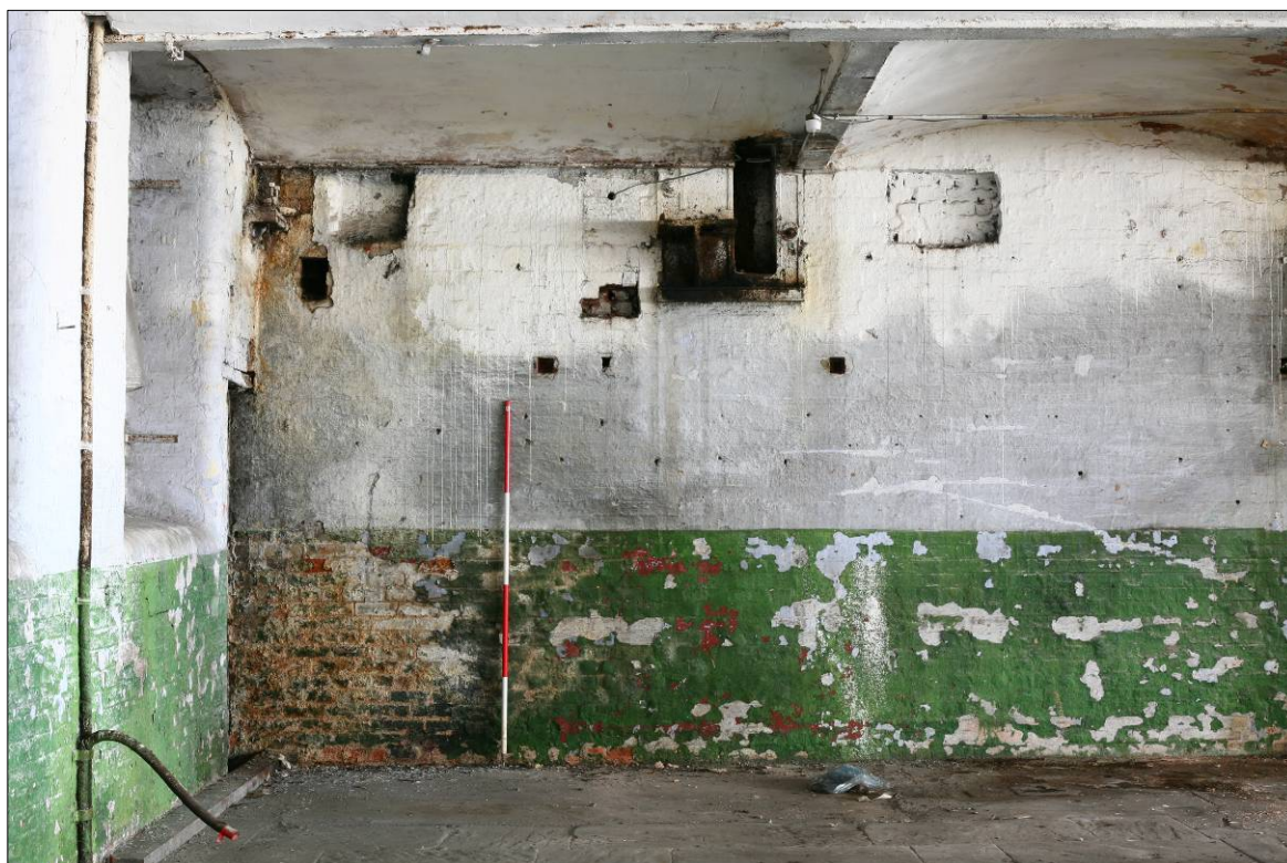
Figure 75. North end of the east wall showing the location of bearing boxes.
