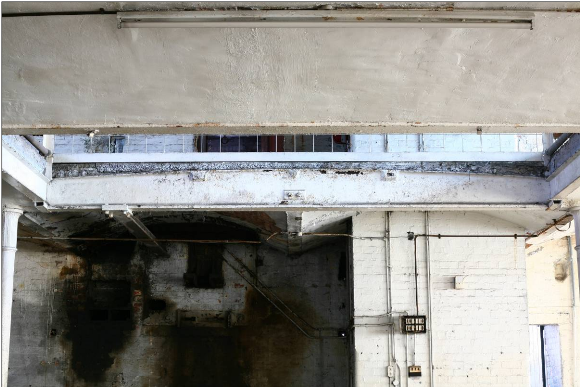
Figure 72. Detail of bowed cast-iron girder.
