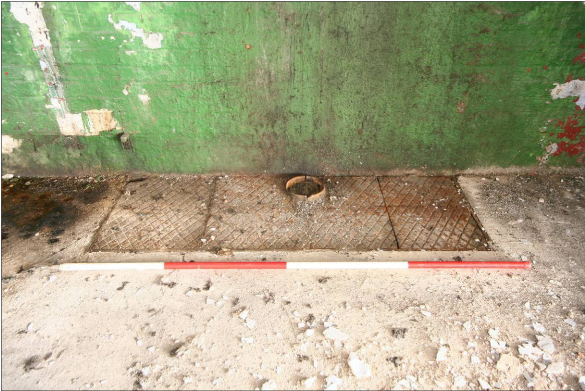
Figure 76. Sheet metal plate covering an opening through to Room G-1 below in the centre of the east wall.
