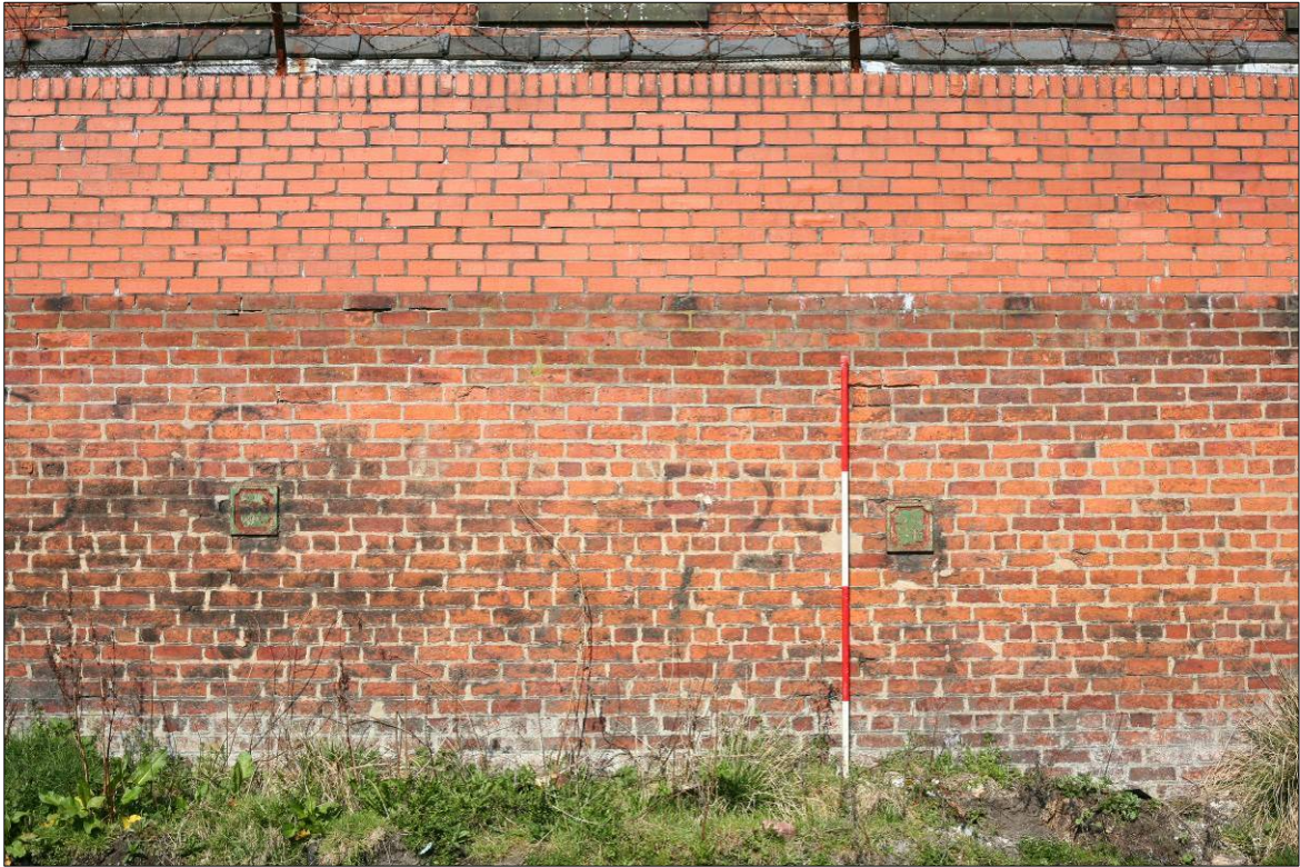
Figure 22. Detailed view of the end of cast-iron brackets running through the South wall.
