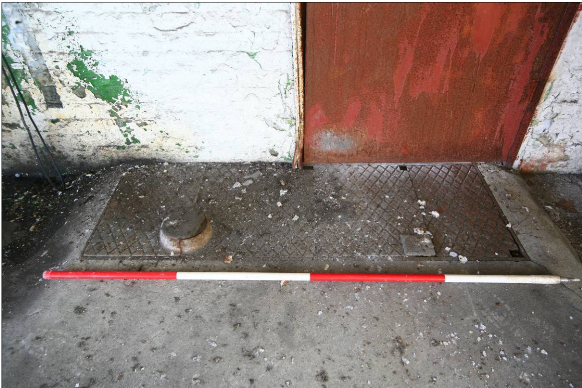
Figure 93. Sheet metal plate over opening in the floor through to Room F-1.
