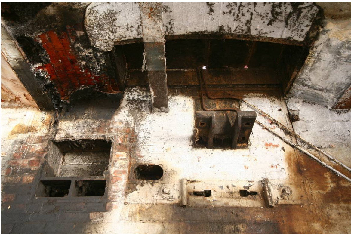
Figure 77. Sheet metal plate in the ceiling, covering a similar opening through to Room S-1 above.
