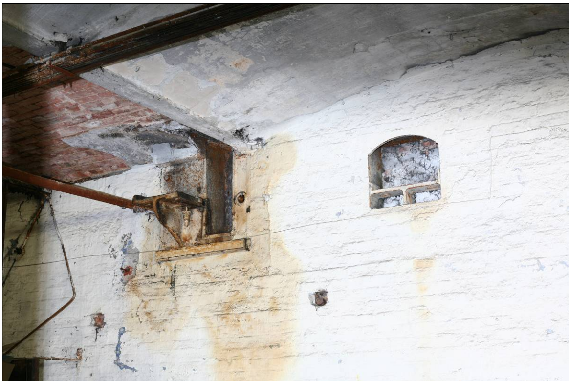
Figure 50. Detail of bearing boxes in the north end of the east wall.
