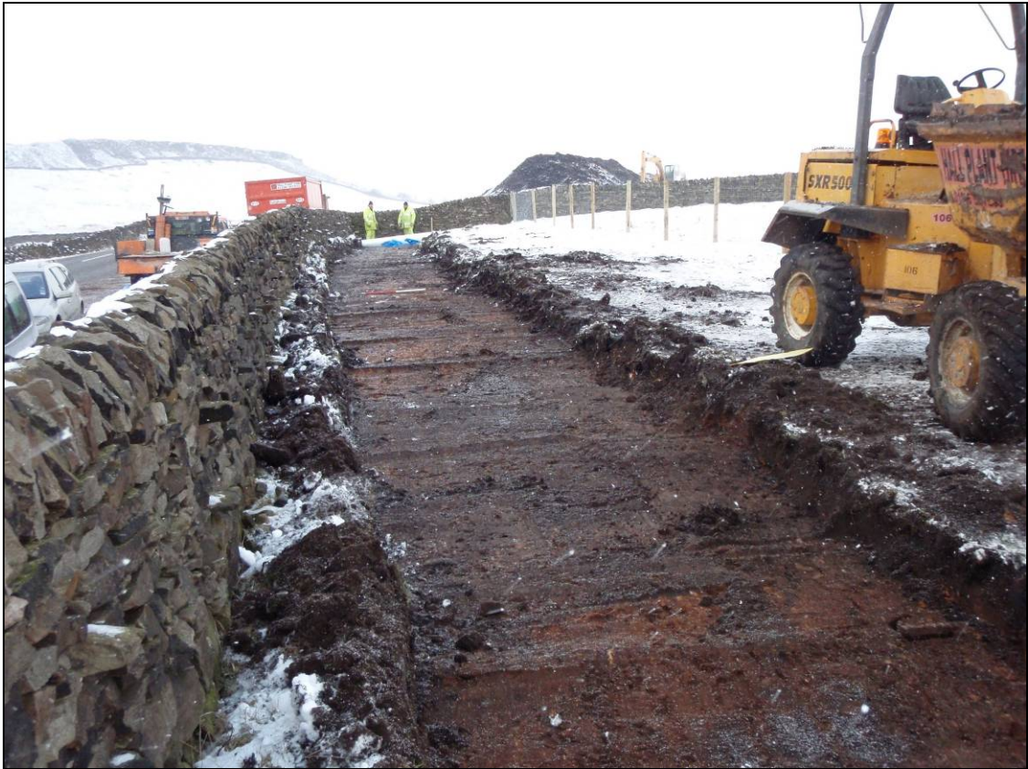
Figure 7: Excavation of the northernmost section of the bridleway, looking north (scale 1m)
