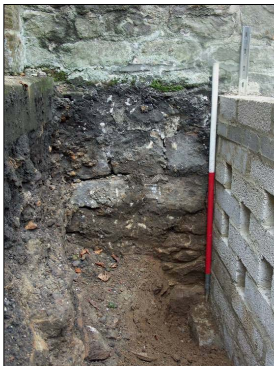
Fig. 12 Lower courses of north wall of the church, looking south (scale 1m).
