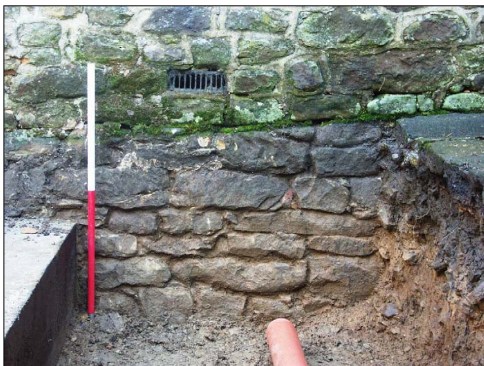
Fig. 13 Lower courses of medieval church exposed after ground reduction, looking south (scale 1m).
