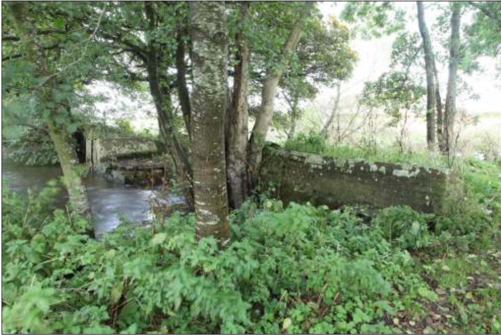
Plate 7: The weir structure prior to demolition showing a detail of the west bank, west wall
