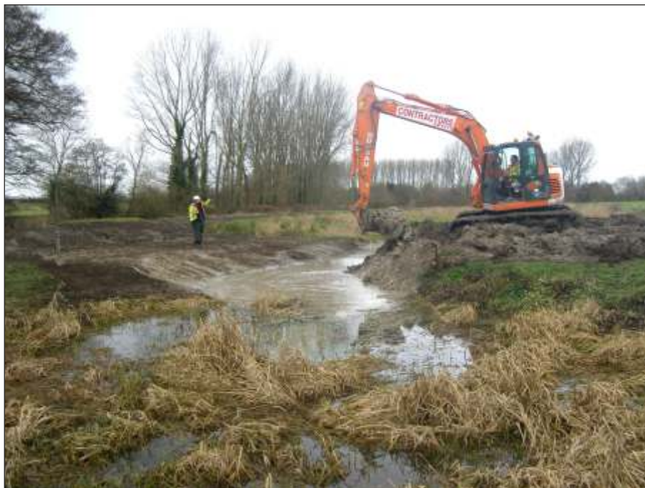
Plate 22: Removal of levee material works prior to culvert removal. View from the south-east
