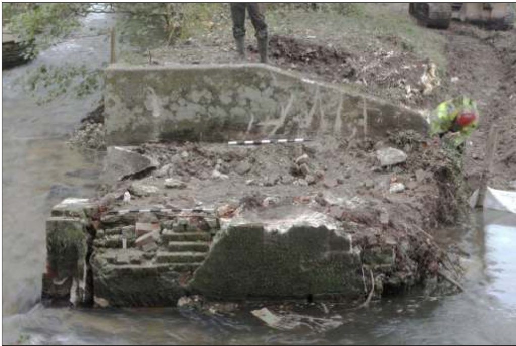
Plate 10: The weir structure on the east bank after the concrete platform was removed. The photo shows the brick sub-structure and earth and rubble infill
