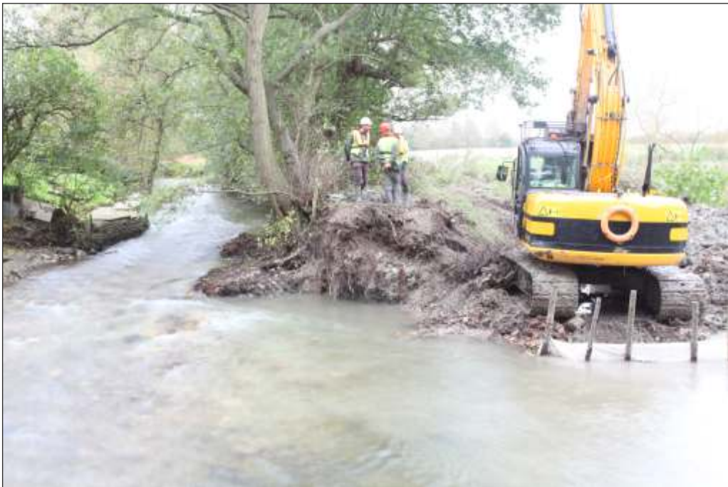
Plate 16: The east bank after the complete demolition of the weir structure but prior to the final re-grading of the bank
