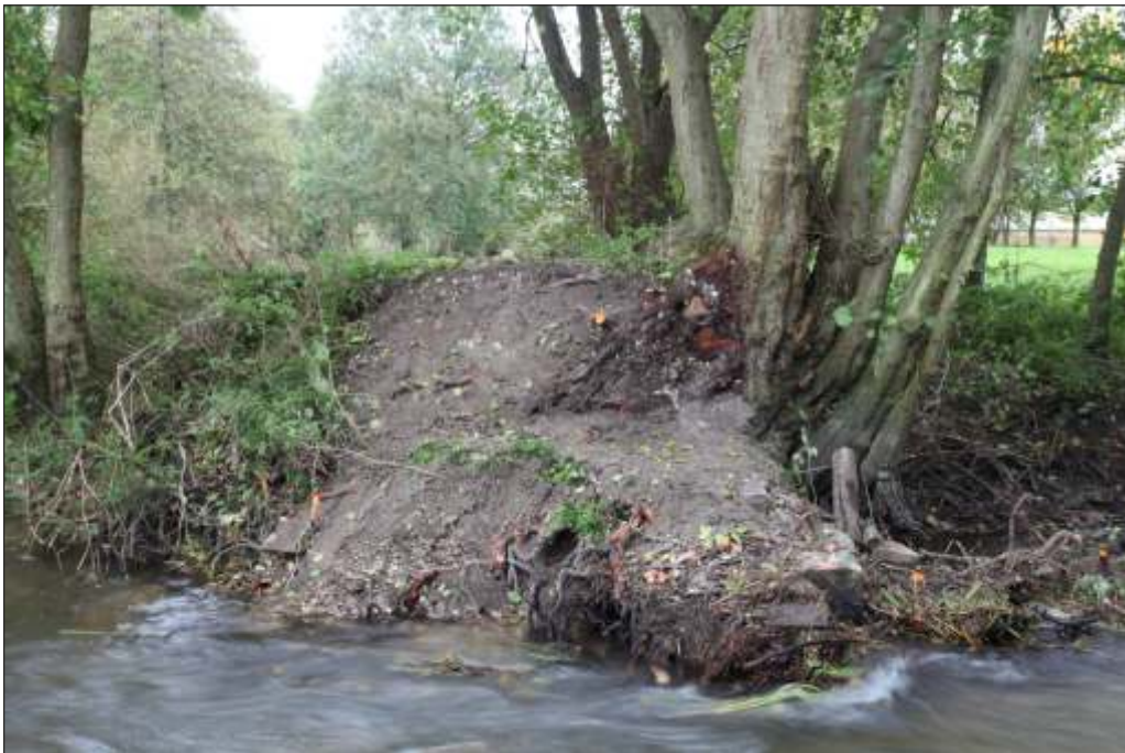
Plate 6: The west bank of the weir structure after demolition and the re-grading of the bank. The course of stone blocks is visible to the lower right of the photo
