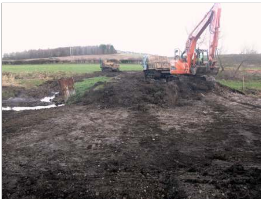
Plate 20: Levee construction material revealed after topsoil strip, (viewed from the southwest) with rubble made ground material on the edge to the left and chalk made ground material on the edge to the right
