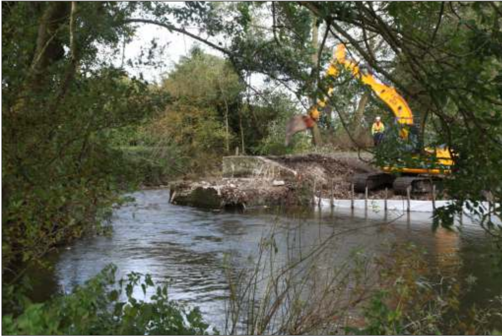
Plate 9: The weir structure on the east bank after the concrete platform was removed
