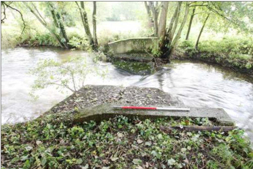
Plate 4: The weir structure viewed from the east to the west bank prior to demolition
