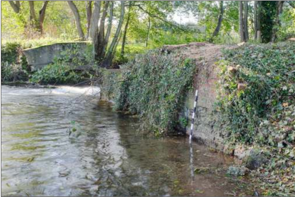
Plate 3: The east bank, east wall (foreground) and west bank (background) of the weir structure prior to demolition
