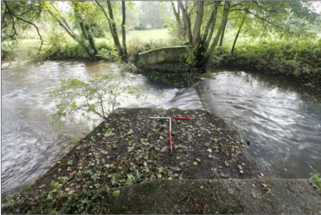
Plate 5: The weir structure viewed from the east to the west bank prior to demolition. The photo shows the east bank concrete platform
