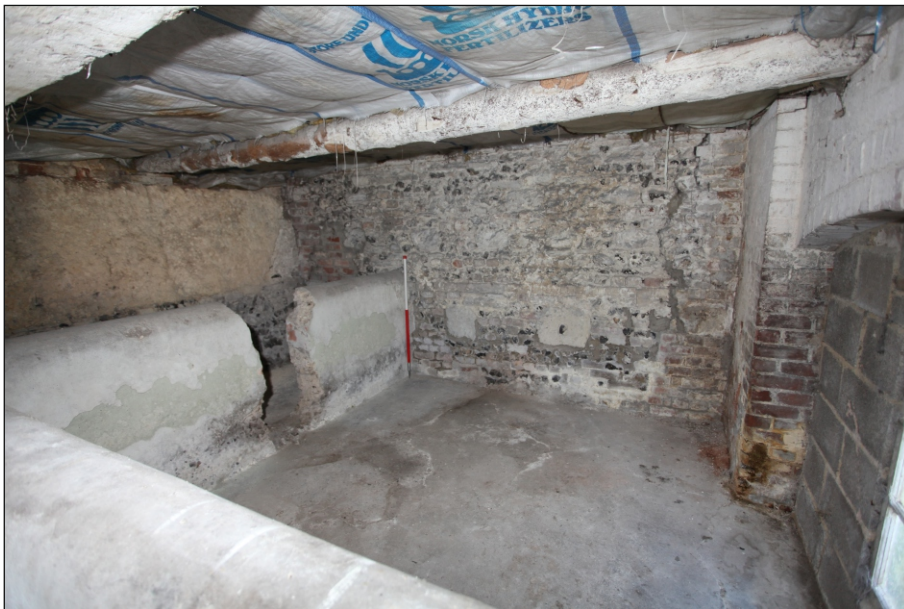
Plate 18: Drax Cottage ground floor west end. Showing typical pigsty and flint west wall with construction joint to right of image
