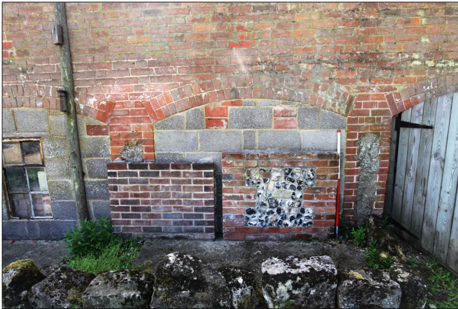
Plate 13: Detail showing cut back pig pen walls to sides of blocked openings
