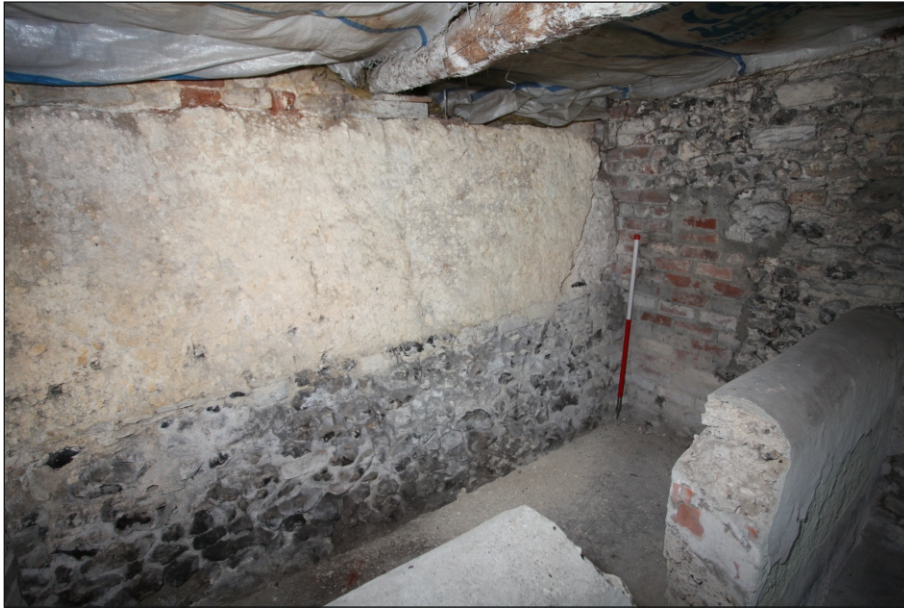
Plate 19: Drax Cottage south wall west end showing internal cob walling on top of flint wall
