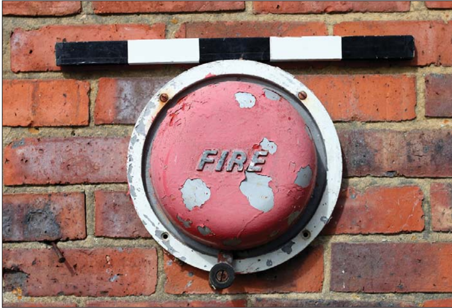
Plate 89: WI 0 218 fire alarm on the south-east side of the building.
