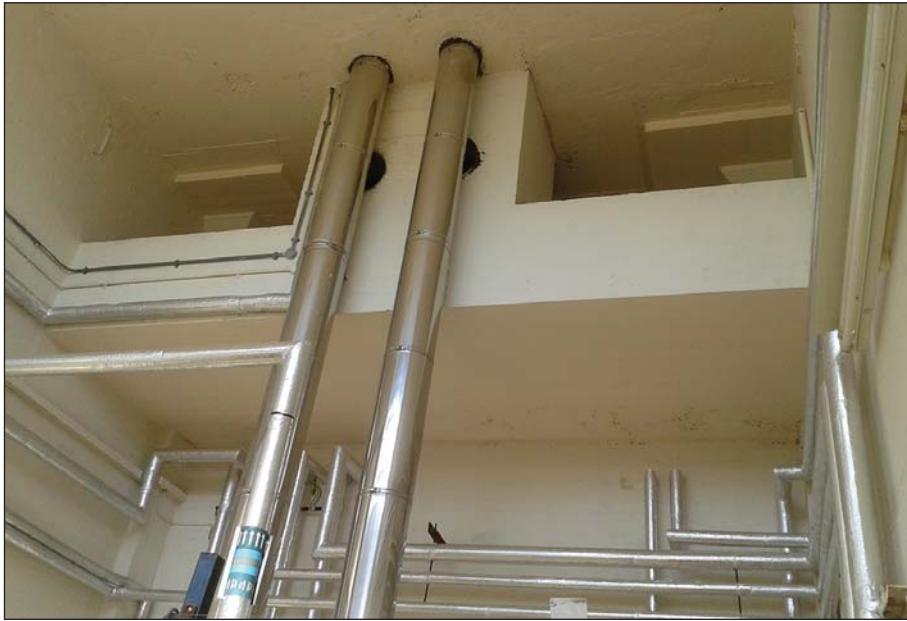
Plate 15: WD 0 040 ground floor. Boiler house high level platform and chimney breast at the north-west end.
