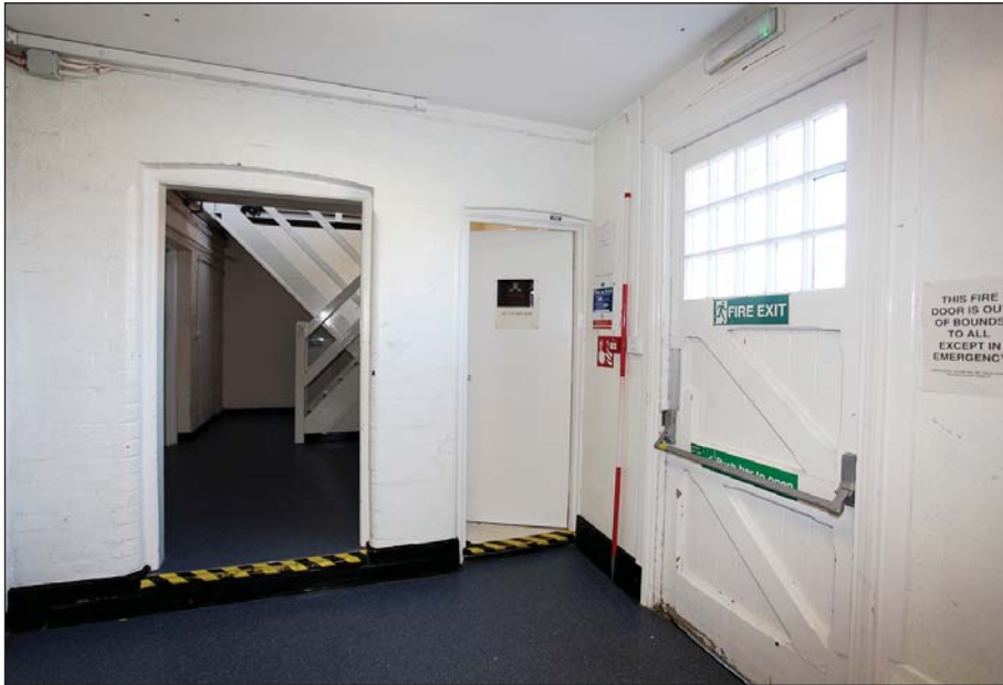
Plate 115: KW 0 415 north-west end of the corridor at the north-east end of the building. It shows the external door (right), toilet door (centre) and staircase to the first floor (background).
