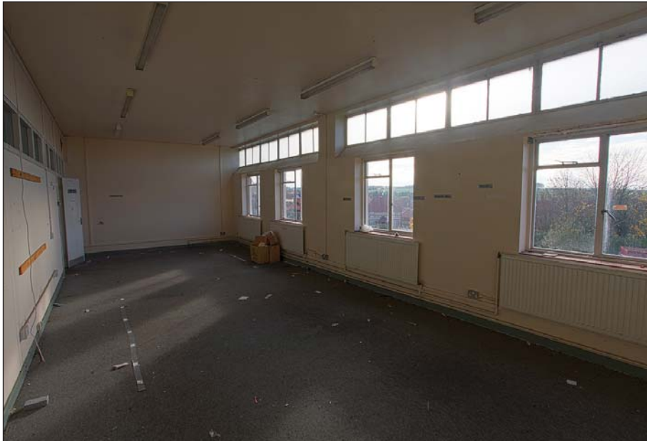
Plate 18: WD 0 040 first floor. A large office. Note the glazing to the internal wall (left) to light the corridor beyond.
