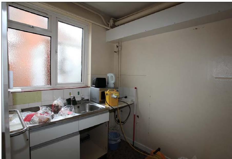
Plate 84: WI 0 216 utility room kitchen (previously a bathroom) viewed from the west. Note the incised line at dado level and blocked door opening (right).
