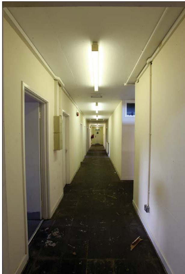
Plate 20: WD 0 040 first floor. Typical corridor viewed from the north. The doors to the original utensil, yeast, salt stores and master baker's office are on the far left.
