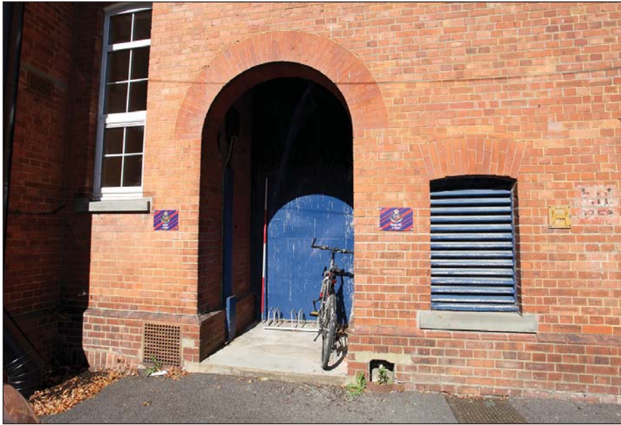
Plate 33: WI 0 082 blocked door on the south-east side of the building. Note the blocked window with its arched head visible to the left of the door and shuttered window and painted fire hydrant sign to the right.
