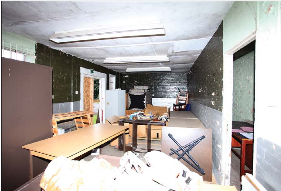
Plate 91: WI 0 218 large store room on the south-east side of the building, viewed from the north. Note the metallic silver paint finish at low level.
