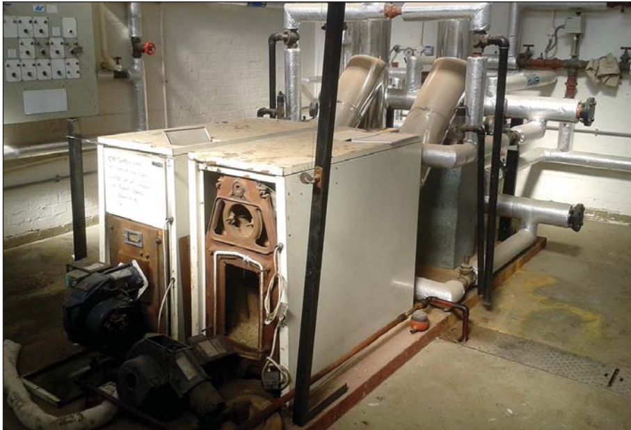
Plate 14: WD 0 040 ground floor. Boiler house equipment.
