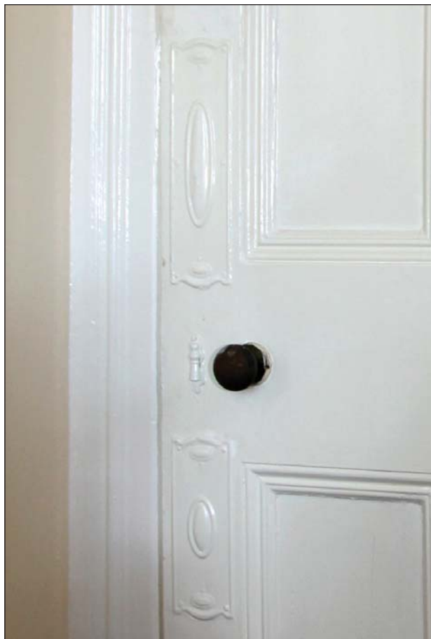
Plate 128: PC 0 707 detail of possibly original door finger plates and other door furniture that appears on several doors in the west range.
