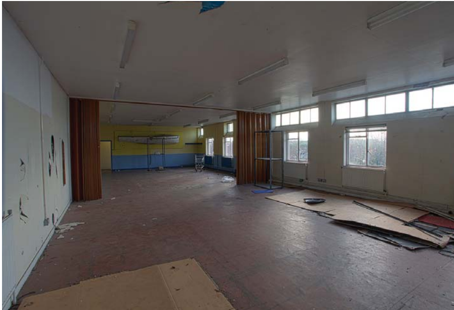
Plate 21: WD 0 040 first floor. Function room at the east corner of the building.
