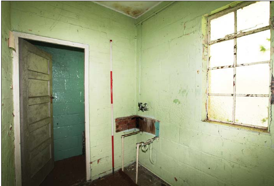
Plate 92: WI 0 218 W.C. showing former location of the sink and the door to the toilet, which is likely original.
