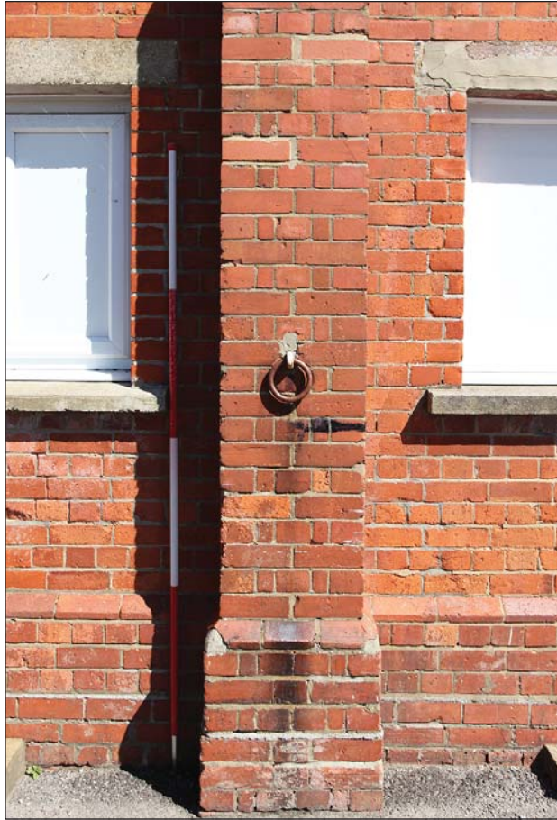
Plate 109: KW 0 415 riding school iron ring fixed to the south-west elevation.
