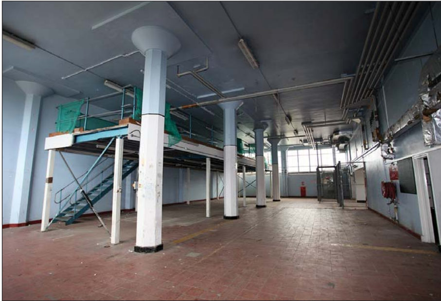
Plate 9: WD 0 040 ground floor. Original oven room after the room had been cleared.
