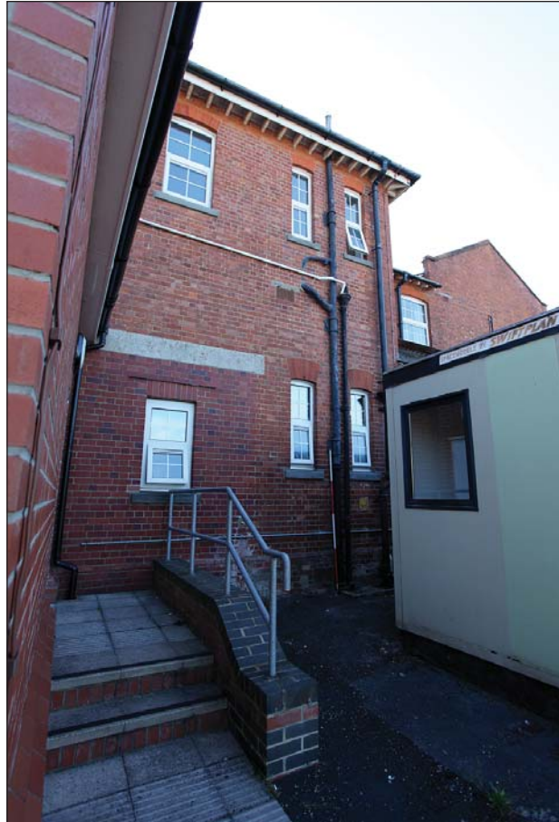
Plate 31: WI 0 082 projecting block on the north-west side of the building, part of the original core. It also shows a window inserted in the one of the former door openings.
