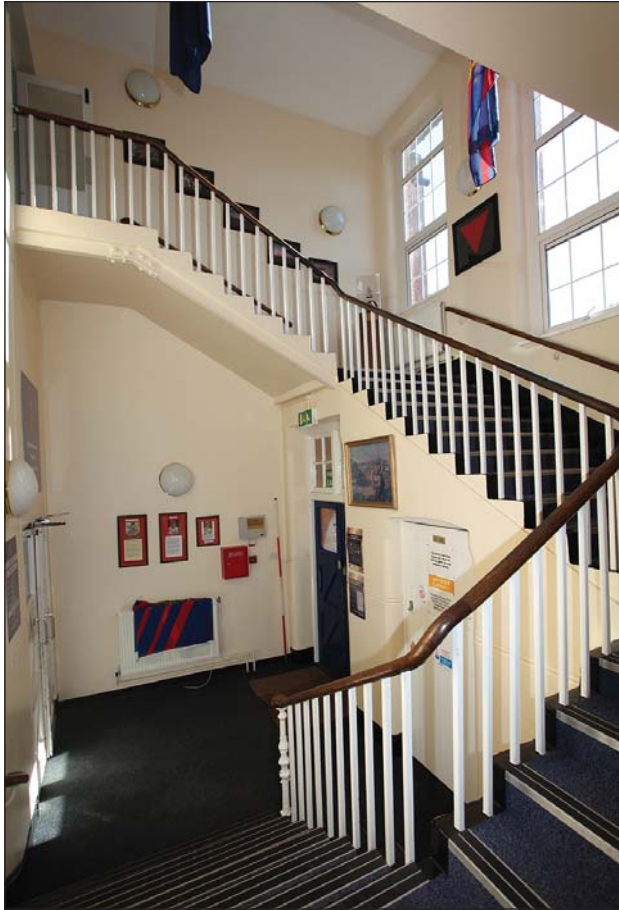
Plate 37: WI 0 082 lobby and stairwell (0.1). The I-beam that supports the upper flight of stairs is visible (top left).
