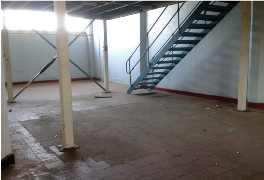
Plate 12: WD 0 040 ground floor. Open room untiled floor surface that marks the location of the final prober.
