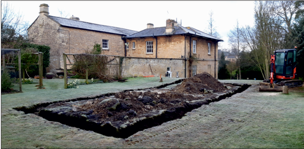
Plate 3: Excavation of the swimming pool exterior wall footing trench. Photo from the north-east
