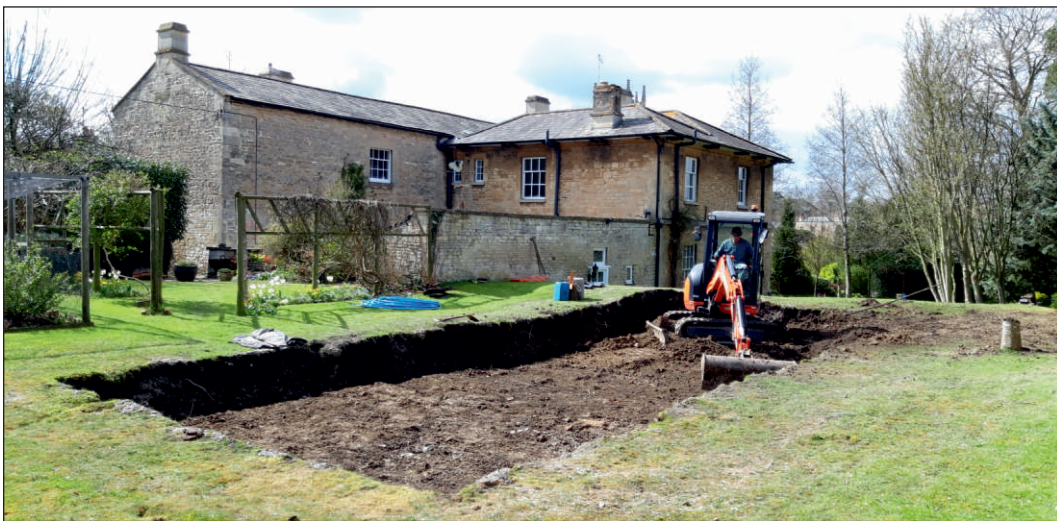
Plate 4: Working shot showing excavation of the swimming pool interior down to the archaeological horizon. Photo taken from the north-east
