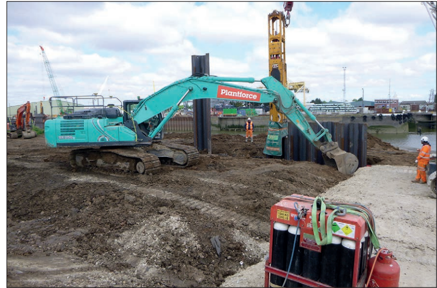
Plate 19: Removing sediment up to 2m from inside the piling while piling is still ongoing
