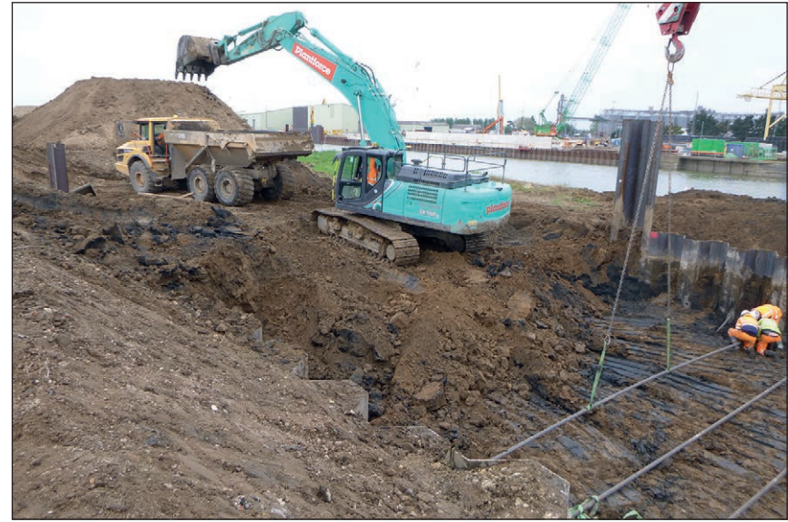
Plate 23: Installation of the tie rods in the trench while excavation is still ongoing
