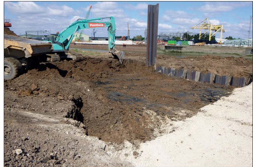
Plate 21: Removing sediment up to 2m from inside the piling while piling is still ongoing
