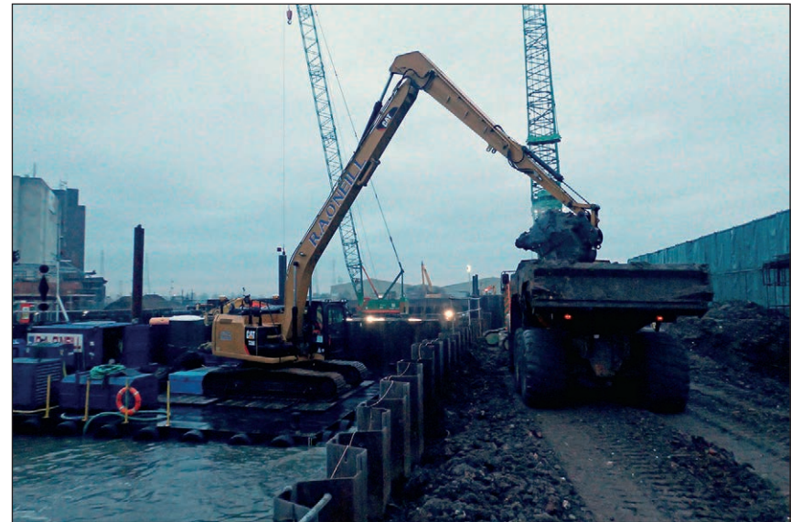
Plate 8: Dredging river to the west of the cofferdam from pontoon and transferring material into hopper
