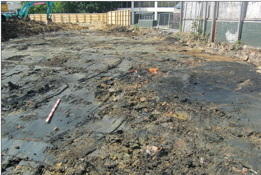
Plate 2: General view of northern extent of strip, view from the north-east. Scale 1 m
