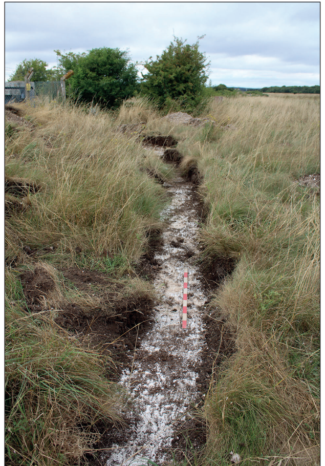
Figure 6: Cable trench from the north-west
