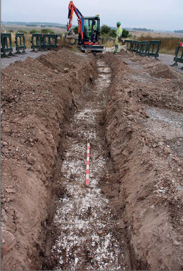
Figure 7: Cable trench from the south-east
