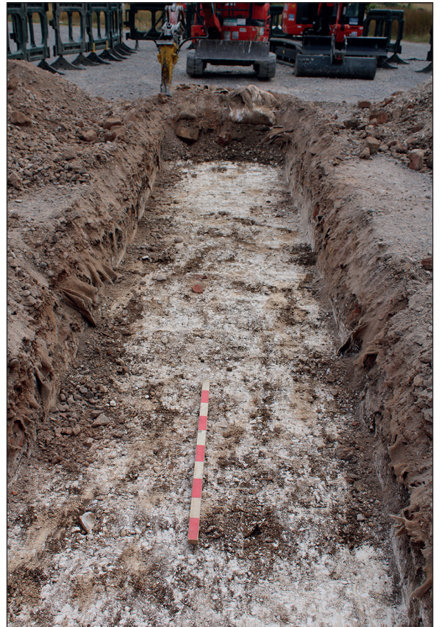
Figure 8: Cable trench from the east
