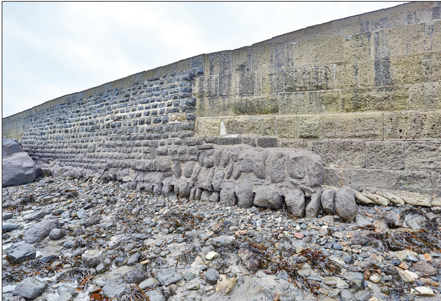
Plate 2: Southern Arm, north face walling, 16th century vertical Cowstones at centre base, 1860's squared Biscuit Work to left, and 1890's Ashlar Portland Stone to right.
