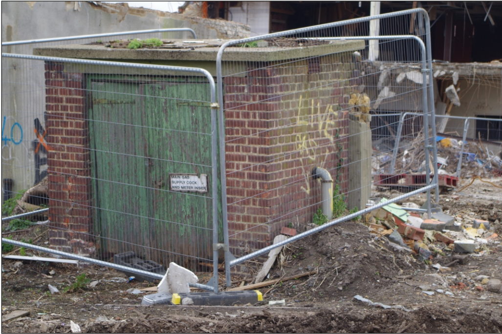
Plate 5: Live gas main warning – location of WB area 2 inside partially demolished building in background
