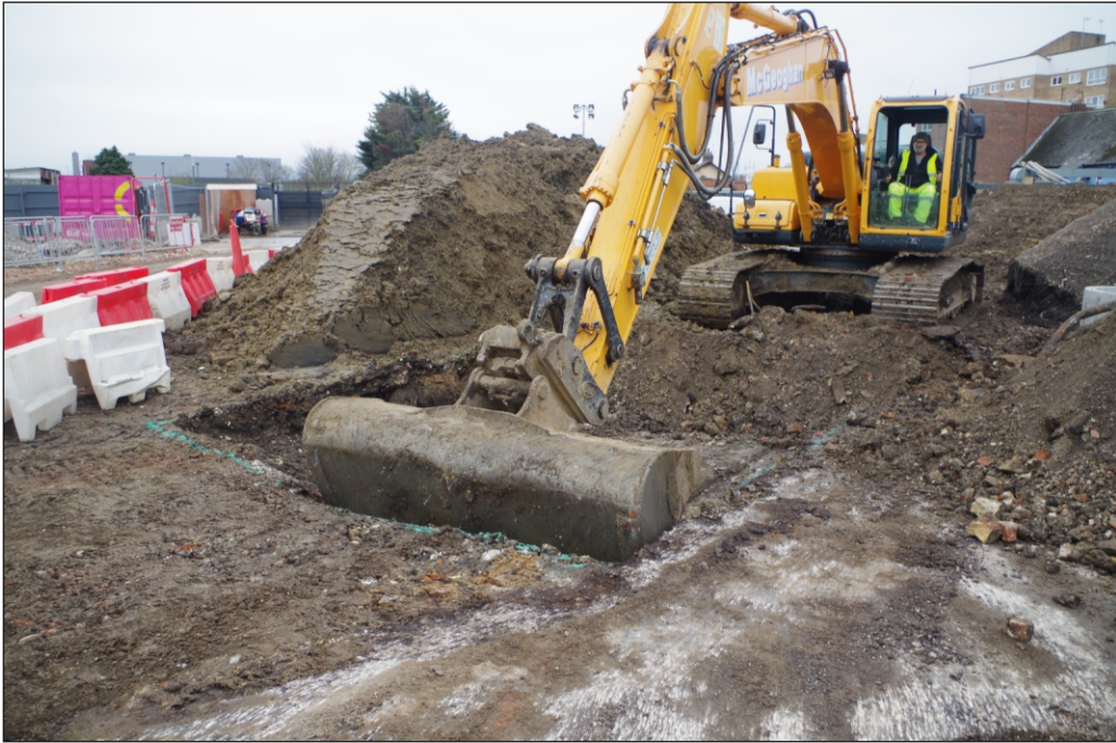
Plate 1: Working shot of WB area 1 – note access constrained by spoil heaps and access road
