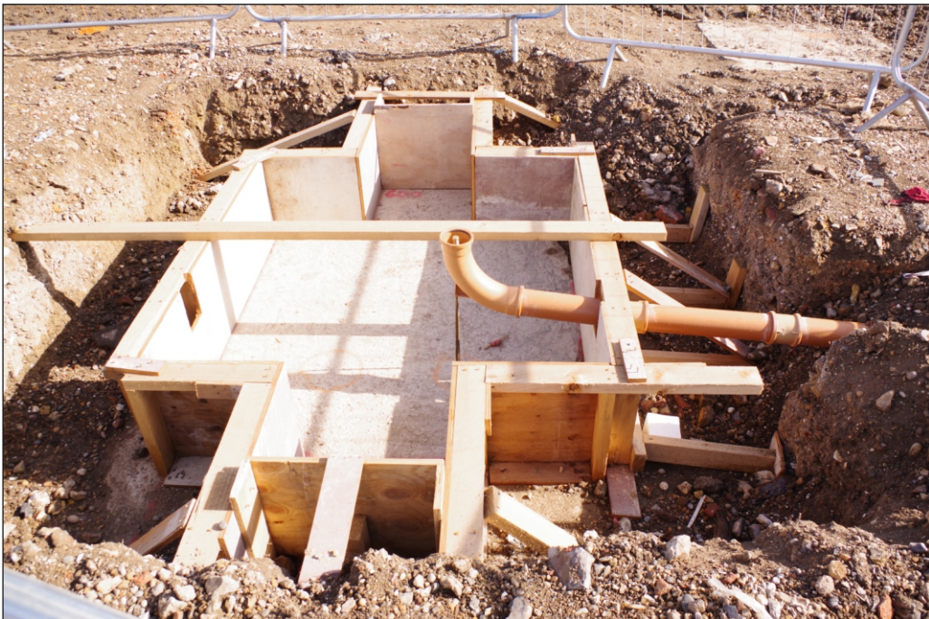
Plate 12: View of conduit system in WB area 5, facing north
