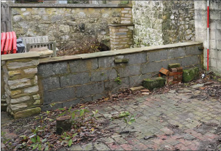
Photograph 15: The south-east side of the garden wall showing exposed concrete blockwork
