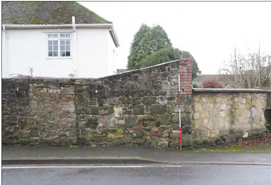
Photograph 6: The sloping section at the western end of the West Street boundary wall
