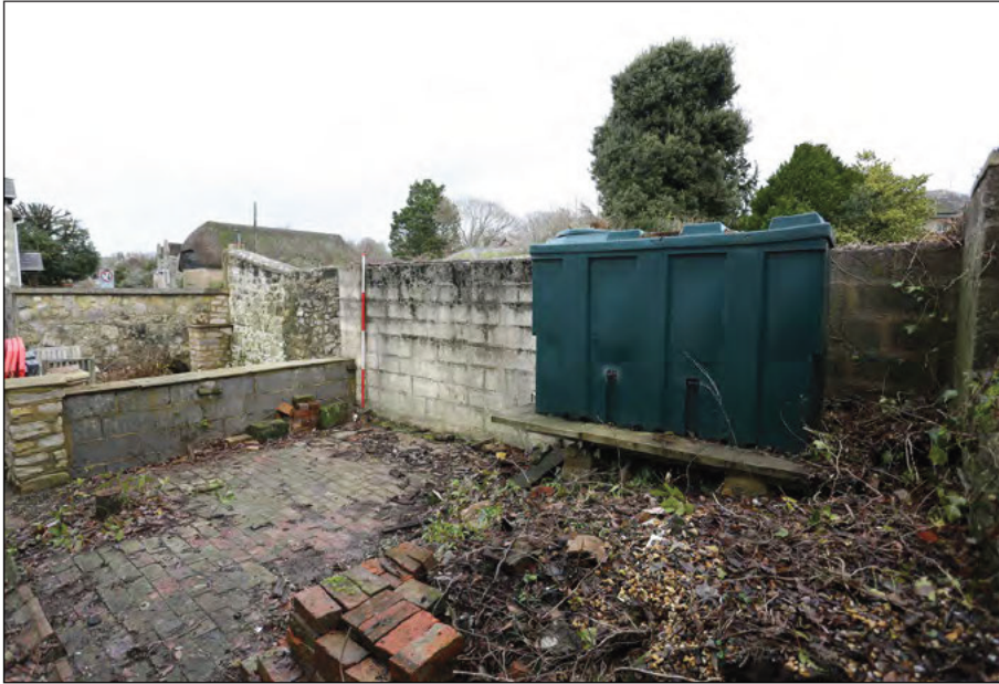
Photograph 11: The south-west side of the West Street boundary wall, viewed from the south
