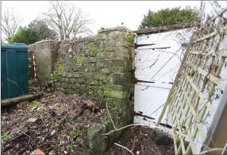
Photograph 19: The Duck Lane boundary wall and short return wall showing the extent of the building that once stood here
