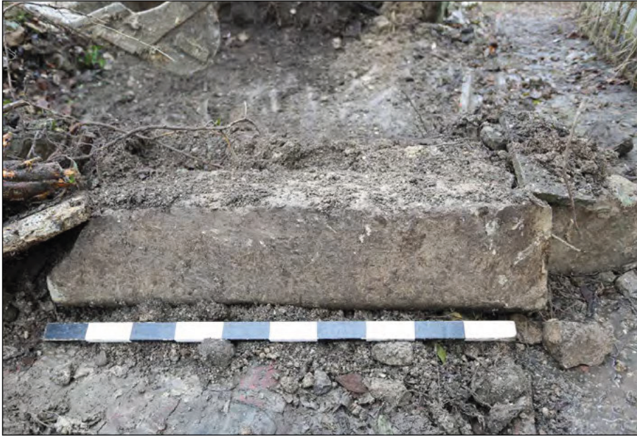
Photograph 25: The moulded L-profile limestone block interpreted as a lintel which was found during demolition
