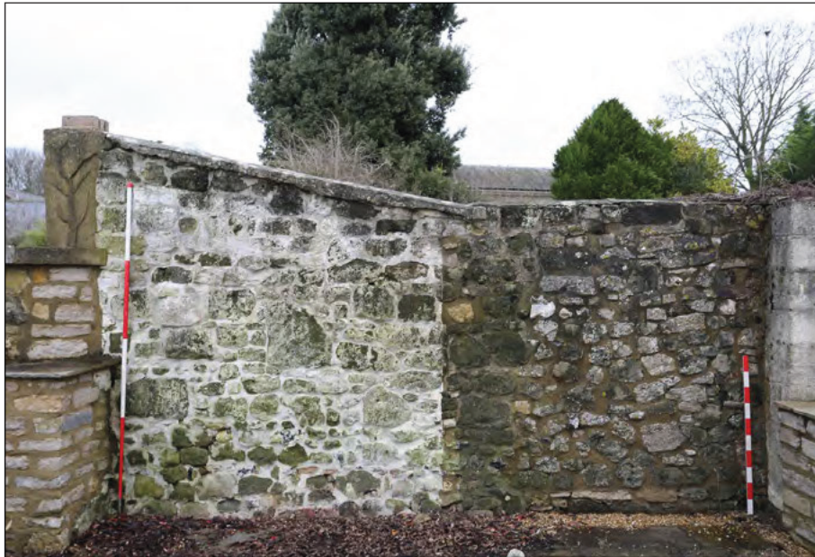
Photograph 13: Remnant paint on the sloping section of wall suggests this was part of a lean-to or mono-pitched structure
