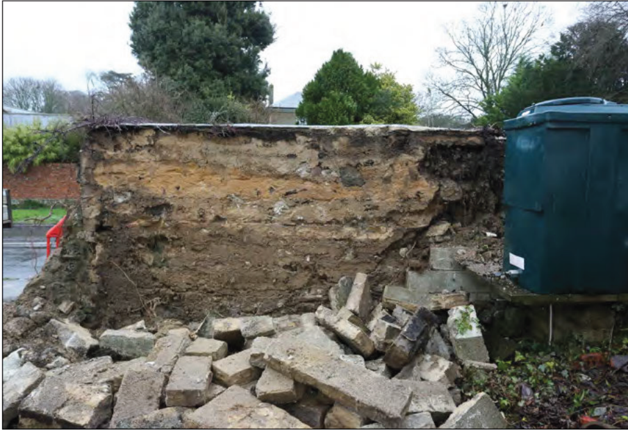
Photograph 23: The south-west elevation of the West Street boundary wall after the removal of the concrete block skin
