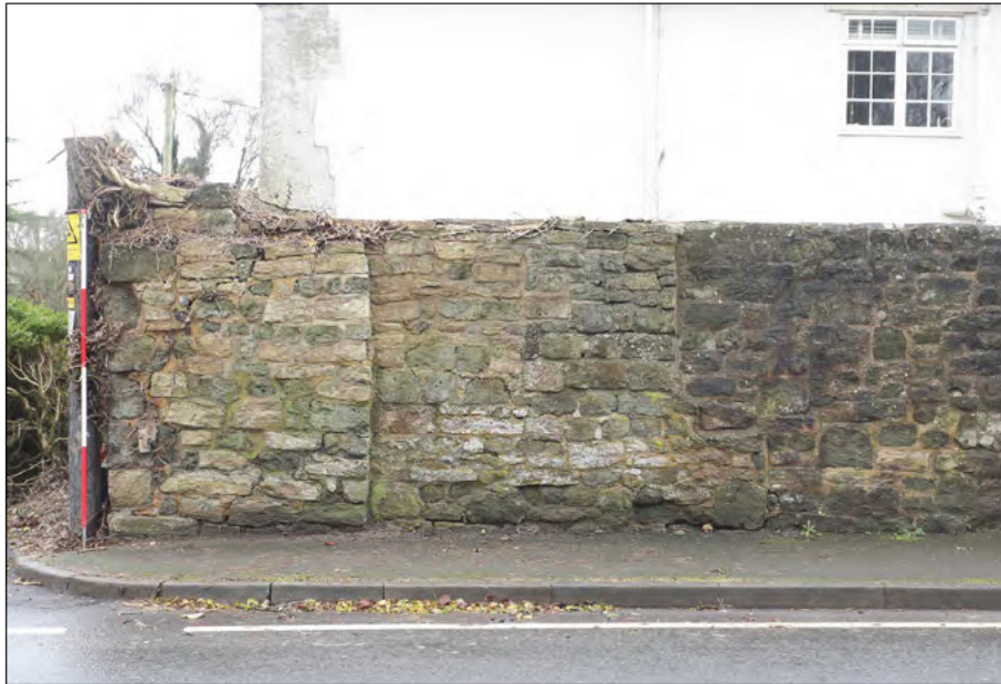
Photograph 9: The sections that form the east end of the West Street boundary wall
