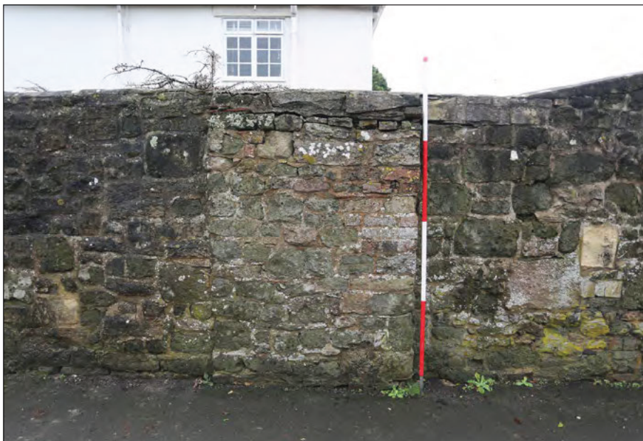
Photograph 8: A blocked door indicated by two straight joints and changes in the coursing and patina of the stone
