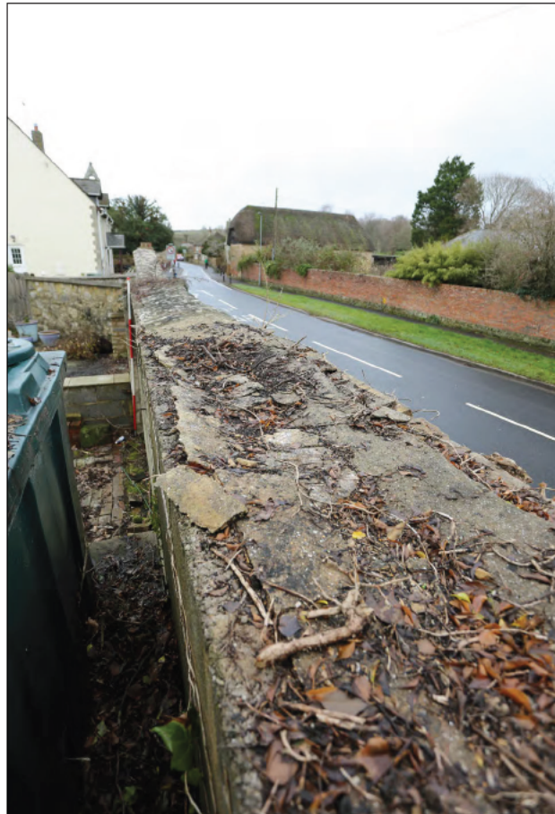
Photograph 4: The irregular top of the West Street boundary wall
