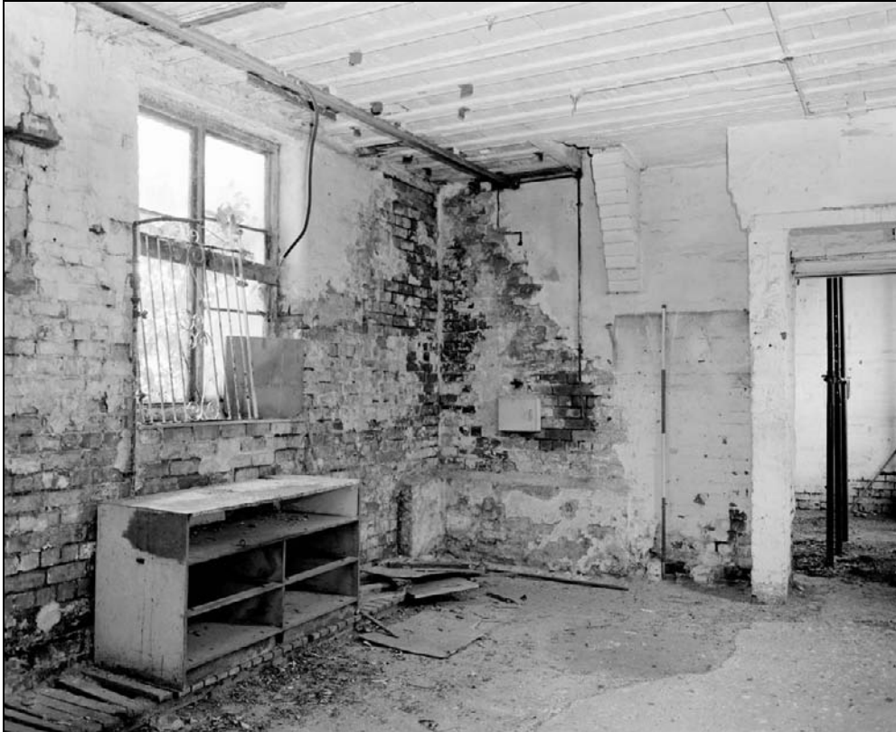
Plate 266: General view of southwest corner of G16 showing type 9 window and scars from removed forge (film 18.10)
