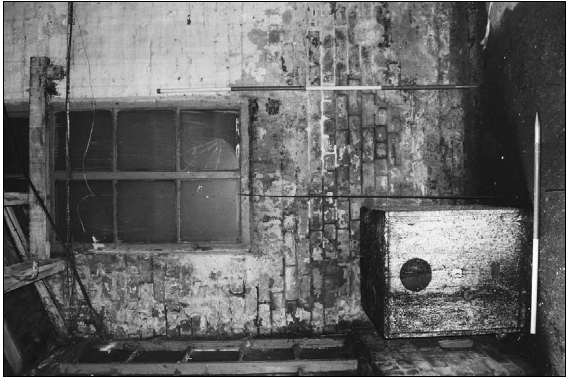
Plate 114: Detail of truncated and blocked window, west wall of G3, west range extension (film 21.7)
