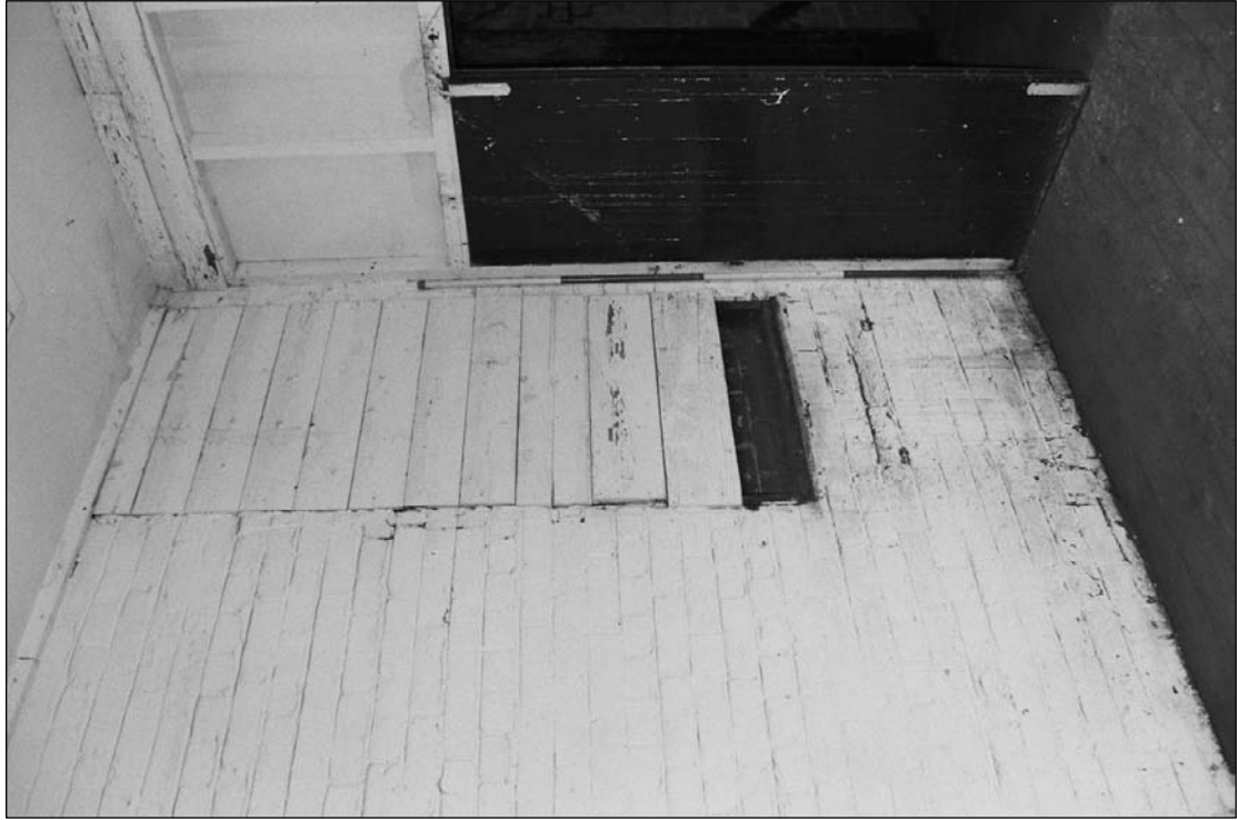
Plate 280: Detail of blocked and boarded opening within south wall of F10, south range (film 26.32)
