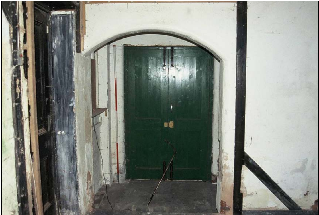
Plate 103: View of archway leading to loading door beneath staircase, room G2, west range (film C/S 2.19)
