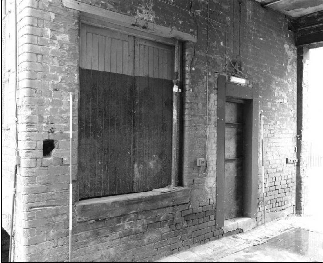
Plate 75: View of the south side of the cart passage, west range, showing loading door and pedestrian doorway within former window (film 20.9)
