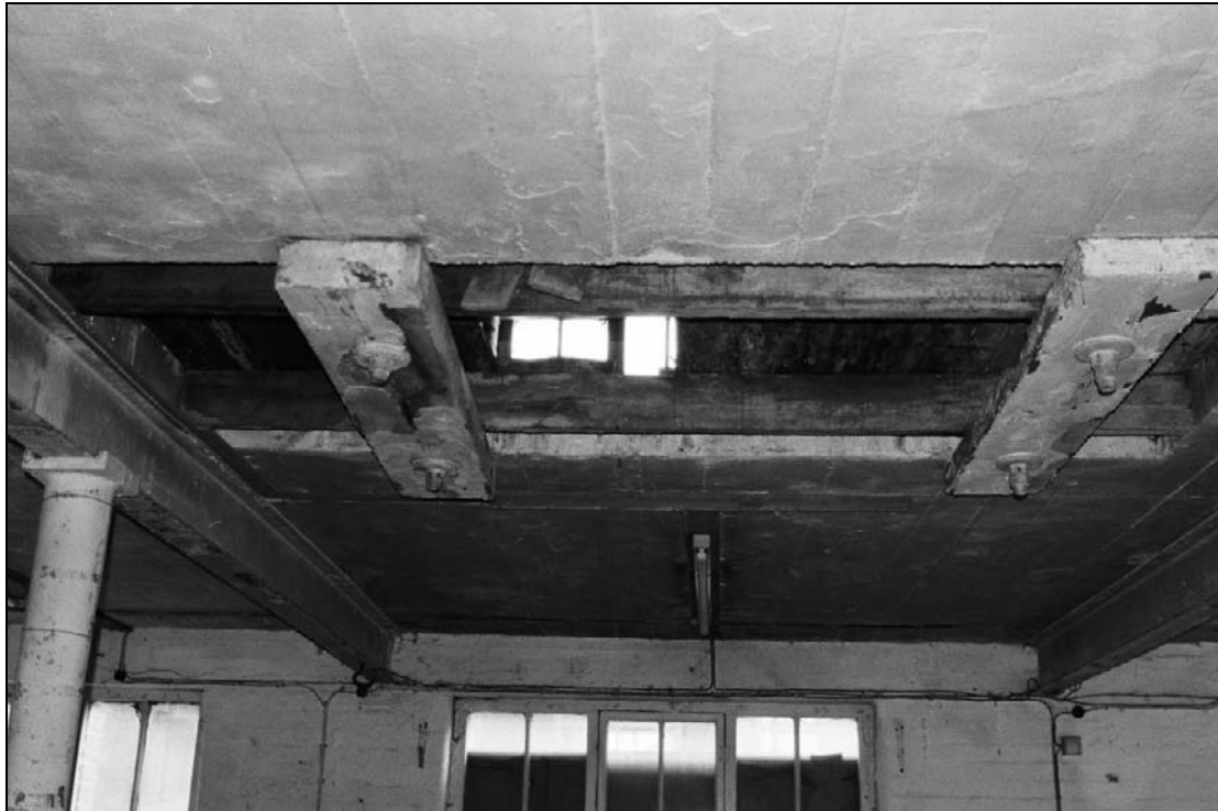
Plate 389: Detail of hatch/opening in ceiling of F4, leading to S5, north range (film 24.18)
