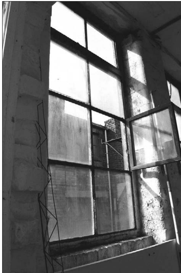
Plate 336: Detail of type 4 window, west wall of F5, showing open casement (film 26.6)
