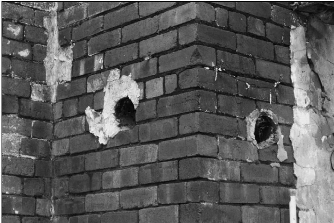
Plate 437: Detail of upper section of chimney stack, northeast corner of G11, furnace house – showing inserted pipes (film 23.7)
