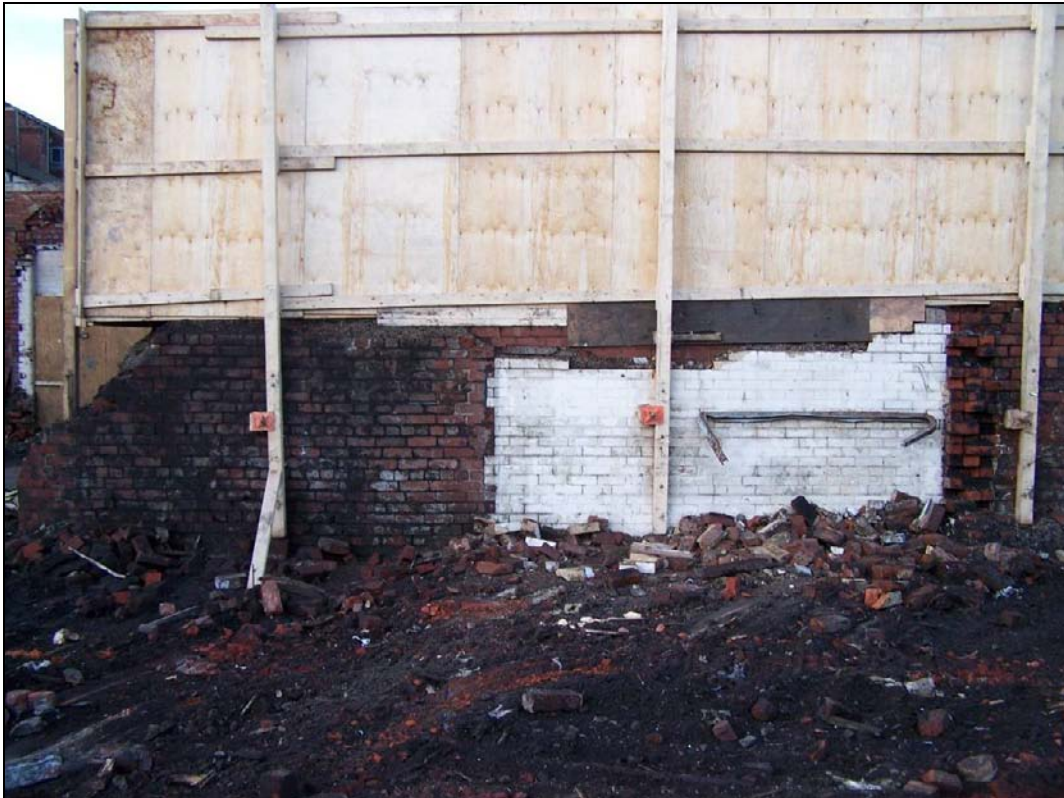
Plate 424: View of north wall of G9, west building of furnace house range, showing vertical joints to east and west (film D.30)
