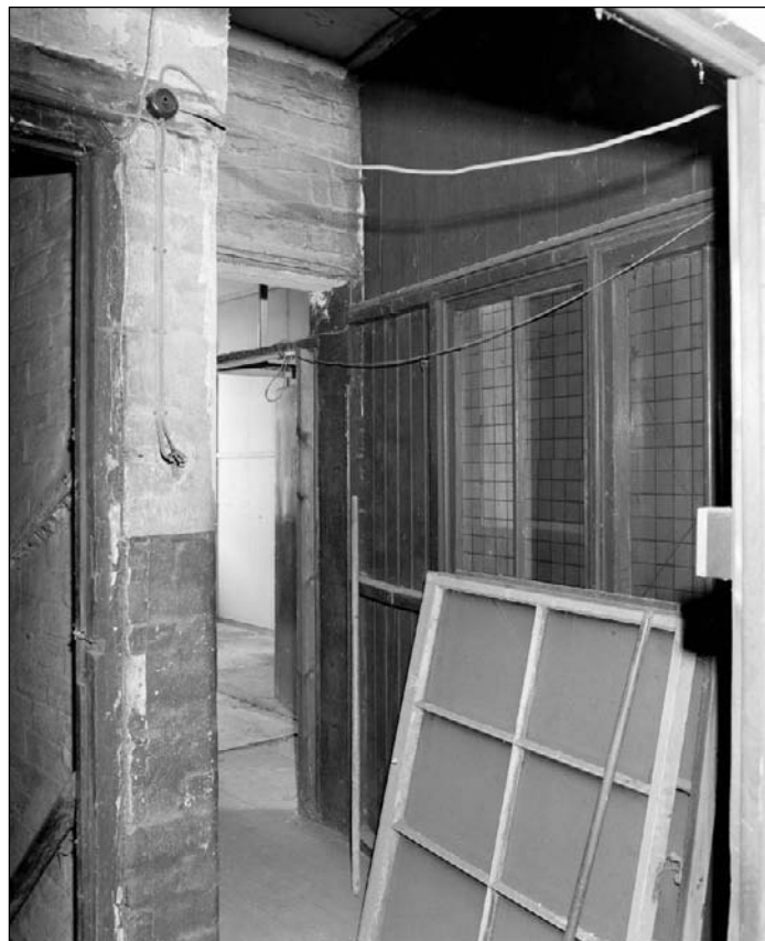
Plate 272: View of south side of timber and glazed partition at west end of F10, south range (west end) leading to F11 (film 29.6)
