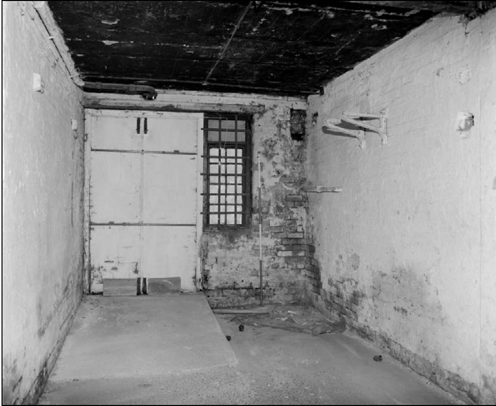
Plate 364: General view of northeast corner of G5, north range, showing widened doorway and inserted ramp (film 15.4)
