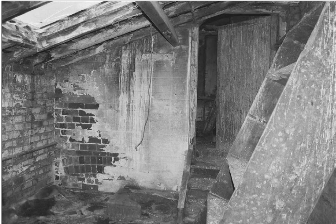
Plate 209: General view of S4 showing doorway from S3 – note blocked window of F3 below (film 44.21)
