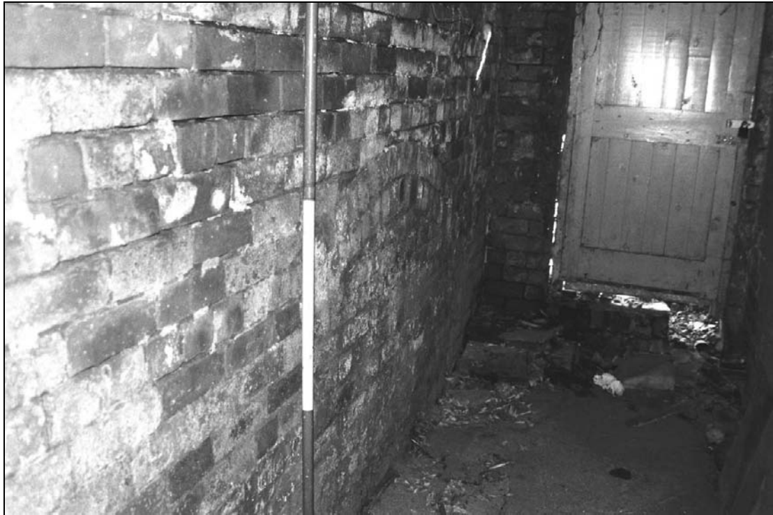
Plate 241: Detail of section of phase 1 wall with archway, east wall of B7, south range (film 27.13)
