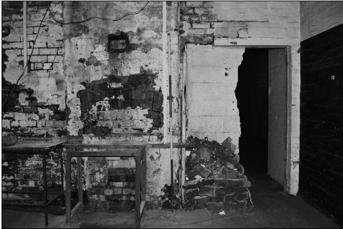
Plate 126: Detail of blocked fireplace and blocked doorway, east wall of G21, west range (film 3.19)
