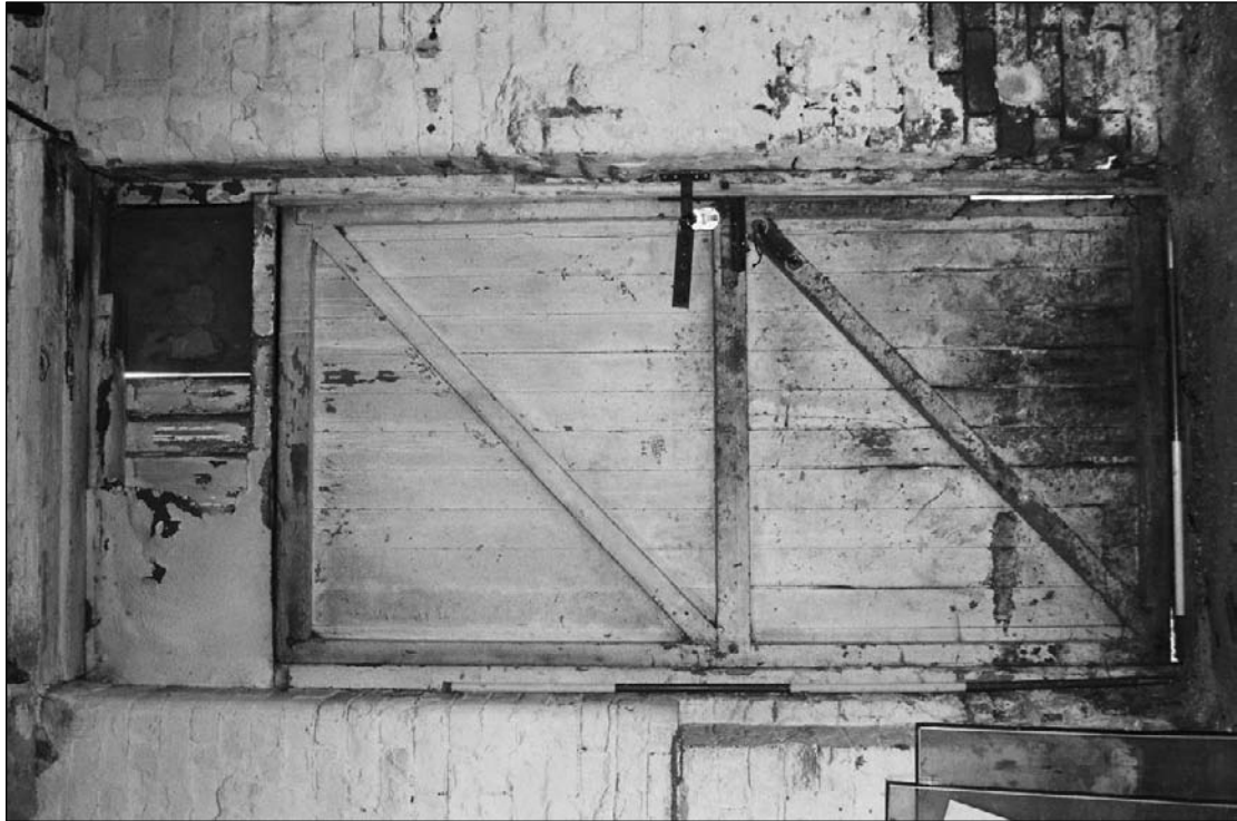
Plate 267: Detail of door within former window opening, north wall of G16, south range (film 23.35)
