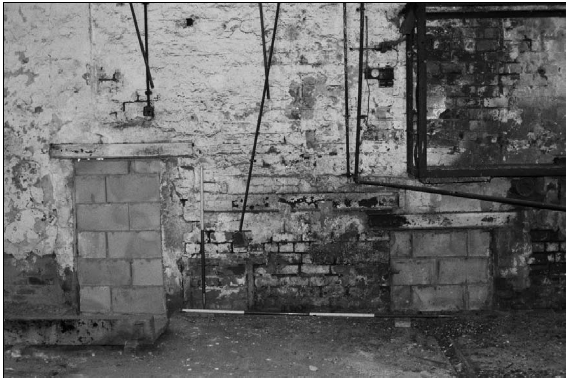
Plate 410: Detail of inserted doorways, blocked with blockwork, west wall of G15, machine shop (film 23.31)
