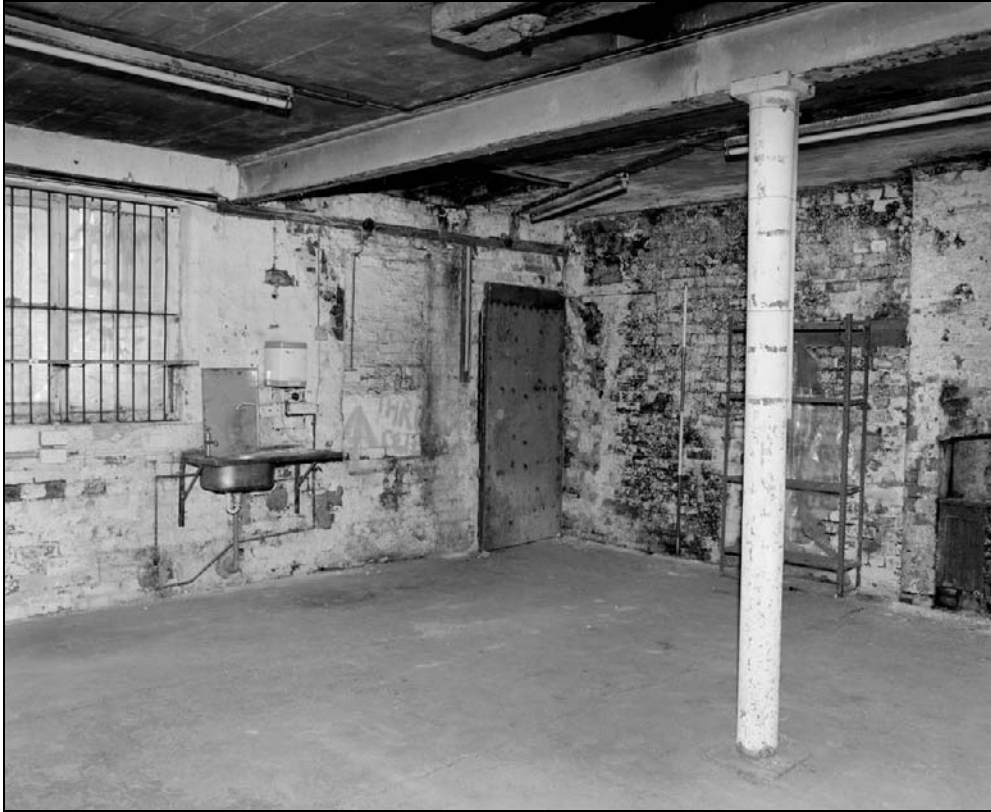
Plate 378: General view of F4, north range – note blocked window and stair scar (film 33.4)
