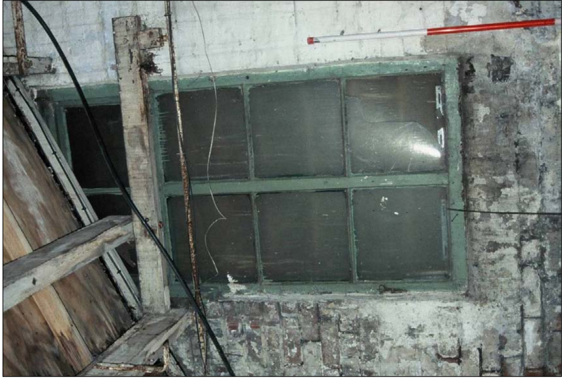
Plate 115: Detail of truncated and blocked window, west wall of G3, west range extension (film C/S 2.22)
