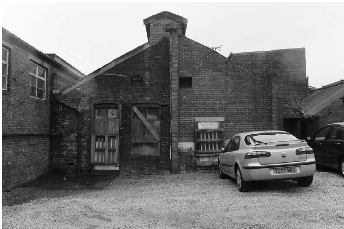
Plate 54: View of east elevation of machine shop showing altered window to door, inserted door and partially re-built northeast corner (film 1.4)
