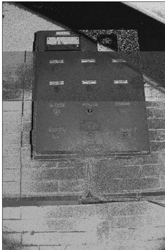
Plate 421: Detail of electrical panel associated with inserted incinerator in G10, furnace house range, west building (film 22.23)
