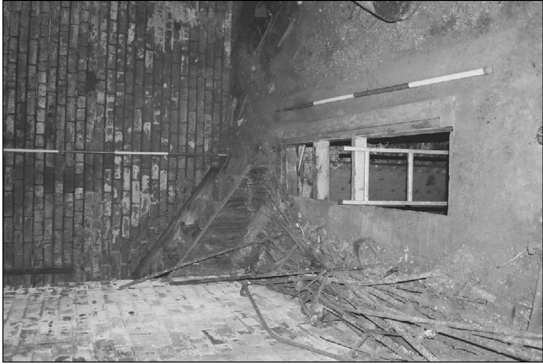
Plate 405: Detail of hatch in floor, leading to F4 below, room S5 (film 44.32)
