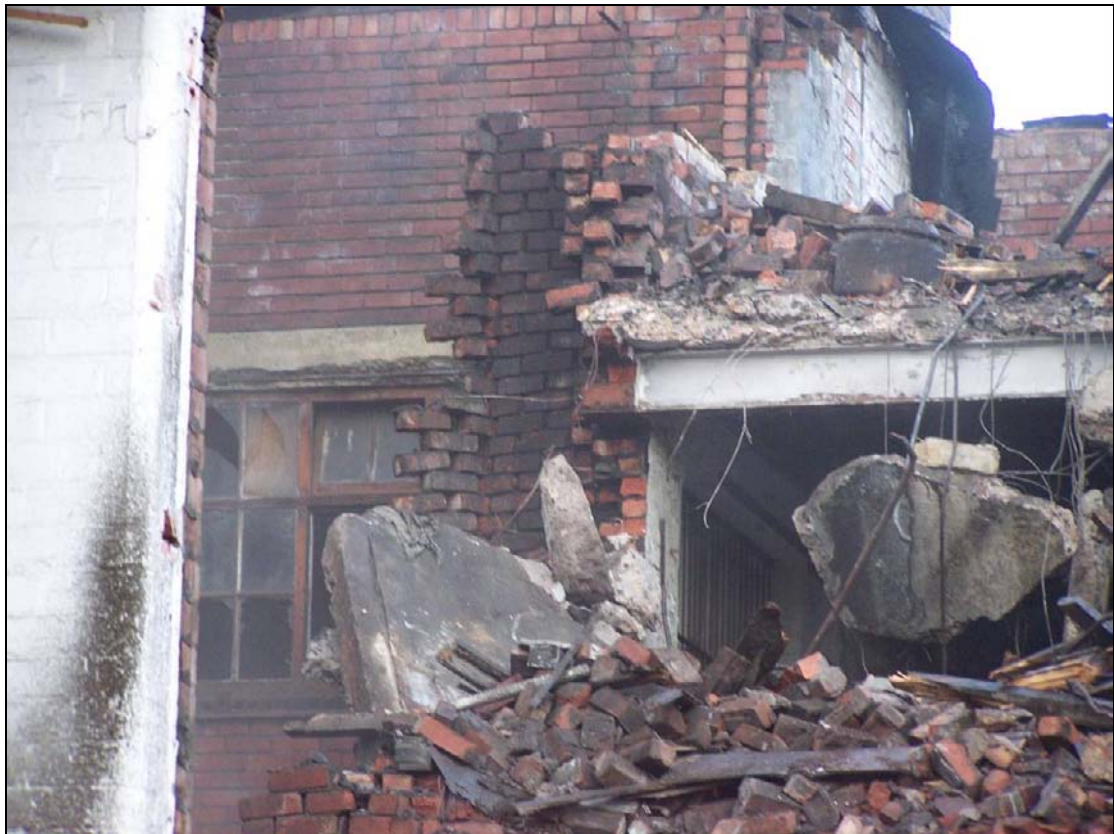
Plate 406: Detail of section through external chimney stack of north range (film D.27)
