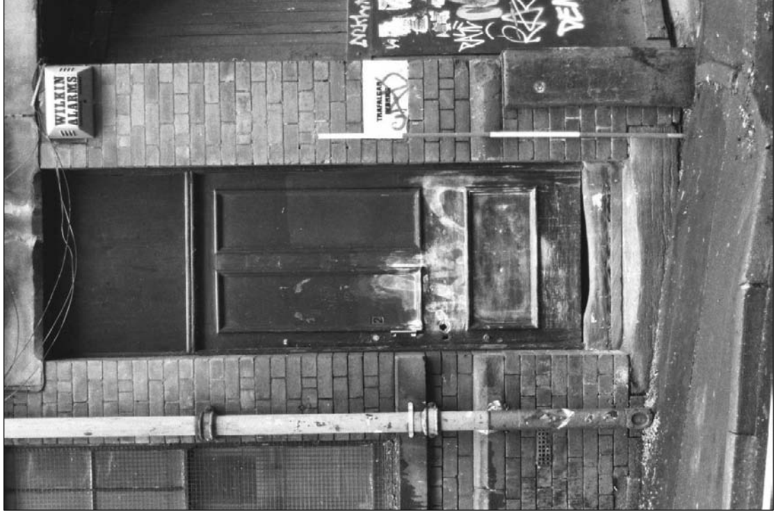
Plate 9: Detail of door leading to G1, west elevation of west range (film 1.31)
