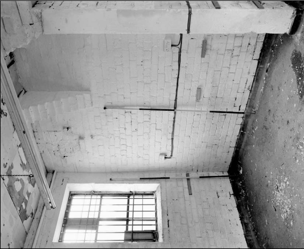
Plate 255: General view of southwest corner of G18 showing stepped brick supports for chimney breast and fireplace on floor above (film 17.9)
