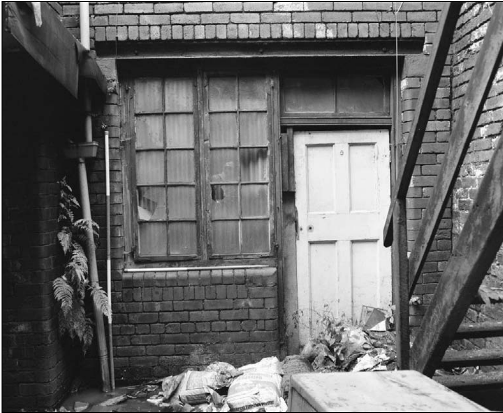
Plate 349: Detail of doorway and type 20 window, east elevation of north range (film 43.1)
