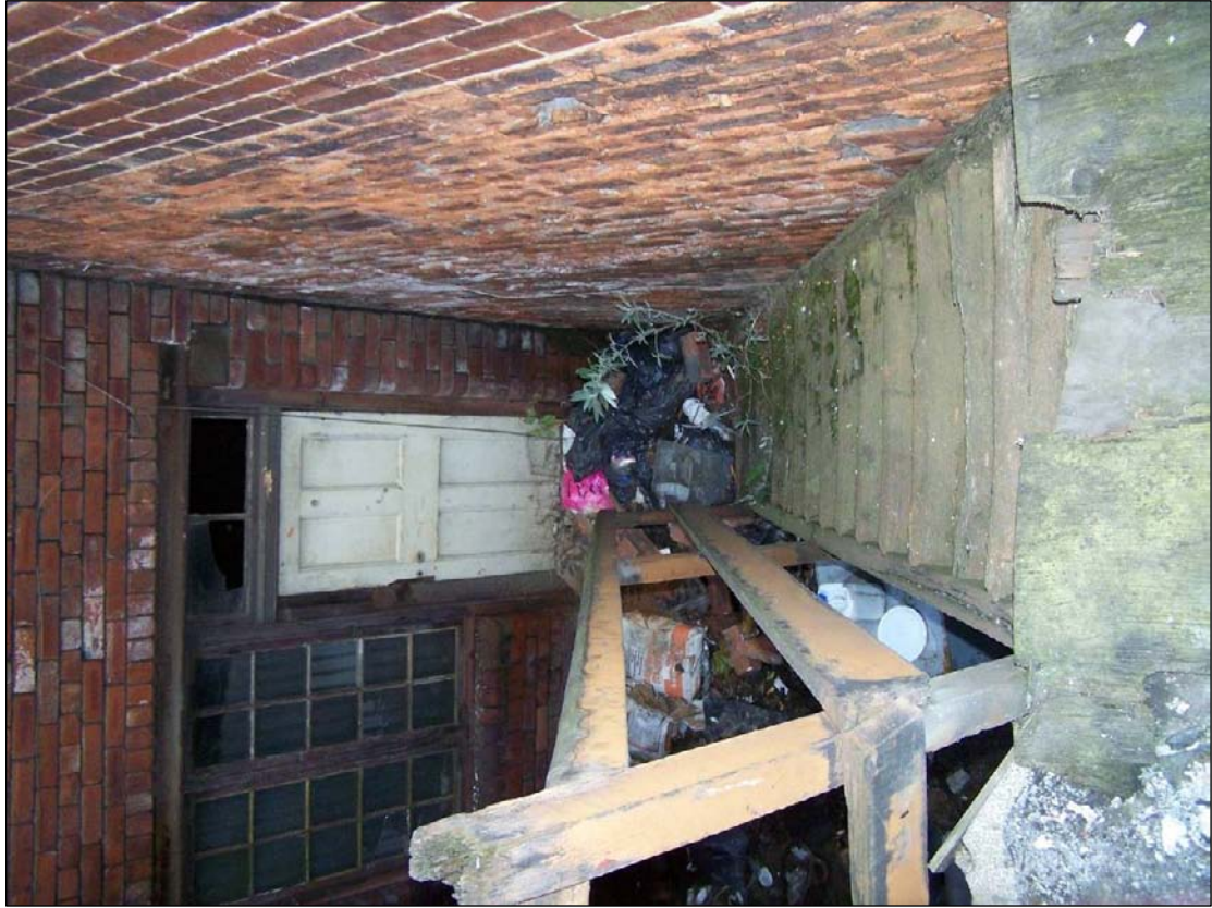
Plate 338: Detail of inserted secondary external staircase leading from F5, east range to central yard (film D.24)
