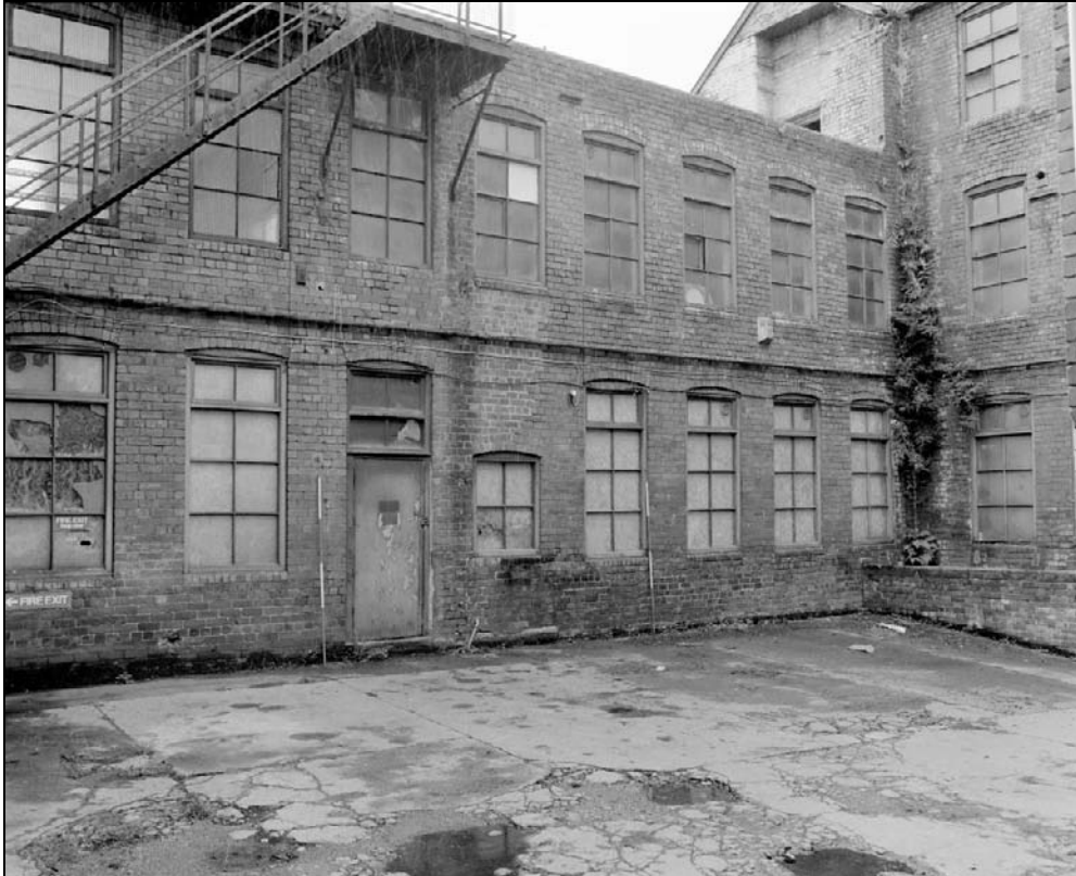
Plate 220: General view of north elevation of the south range (west end) – note removed 2 nd floor (film 9.10)
