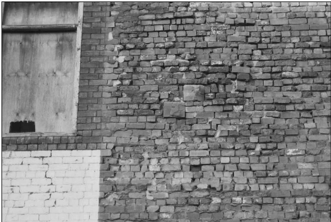
Plate 25: Detail of change in brickwork finish and concrete stairends, south elevation of west range (film 46.22)
