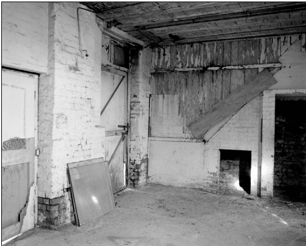
Plate 264: General view of G16 – note inserted door within former window and partitioned inserted staircase with storage space beneath (film 18.6)
