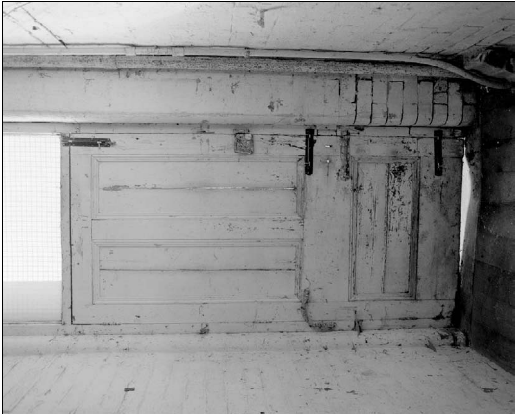
Plate 120: Detail of main door leading from Trafalgar Street into G23, west range (film 15.8)
