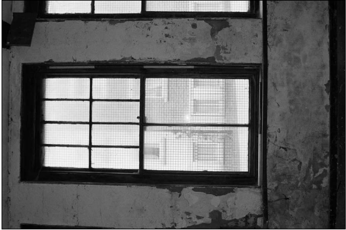
Plate 106: Detail of type 2 window, west wall of room G2, west range (film 22.29)
