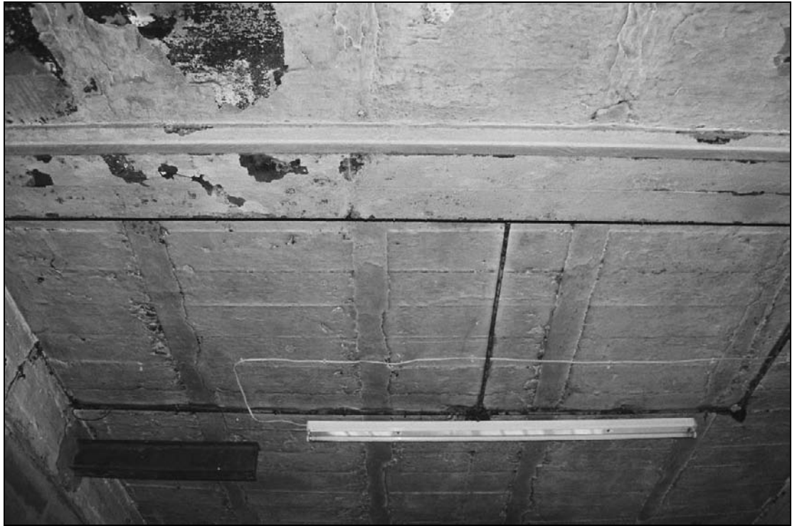
Plate 366: Detail of ceiling of G5 showing steel I-section beam indicating position of removed wall and shuttered concrete ceiling (film 21.11)
