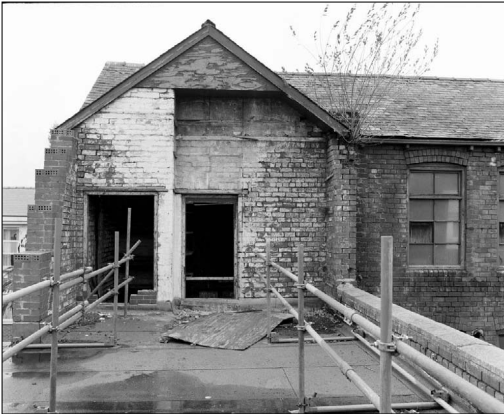
Plate 180: Detail of doorways to second floor of west range, from removed second floor of south range (film 12.9)
