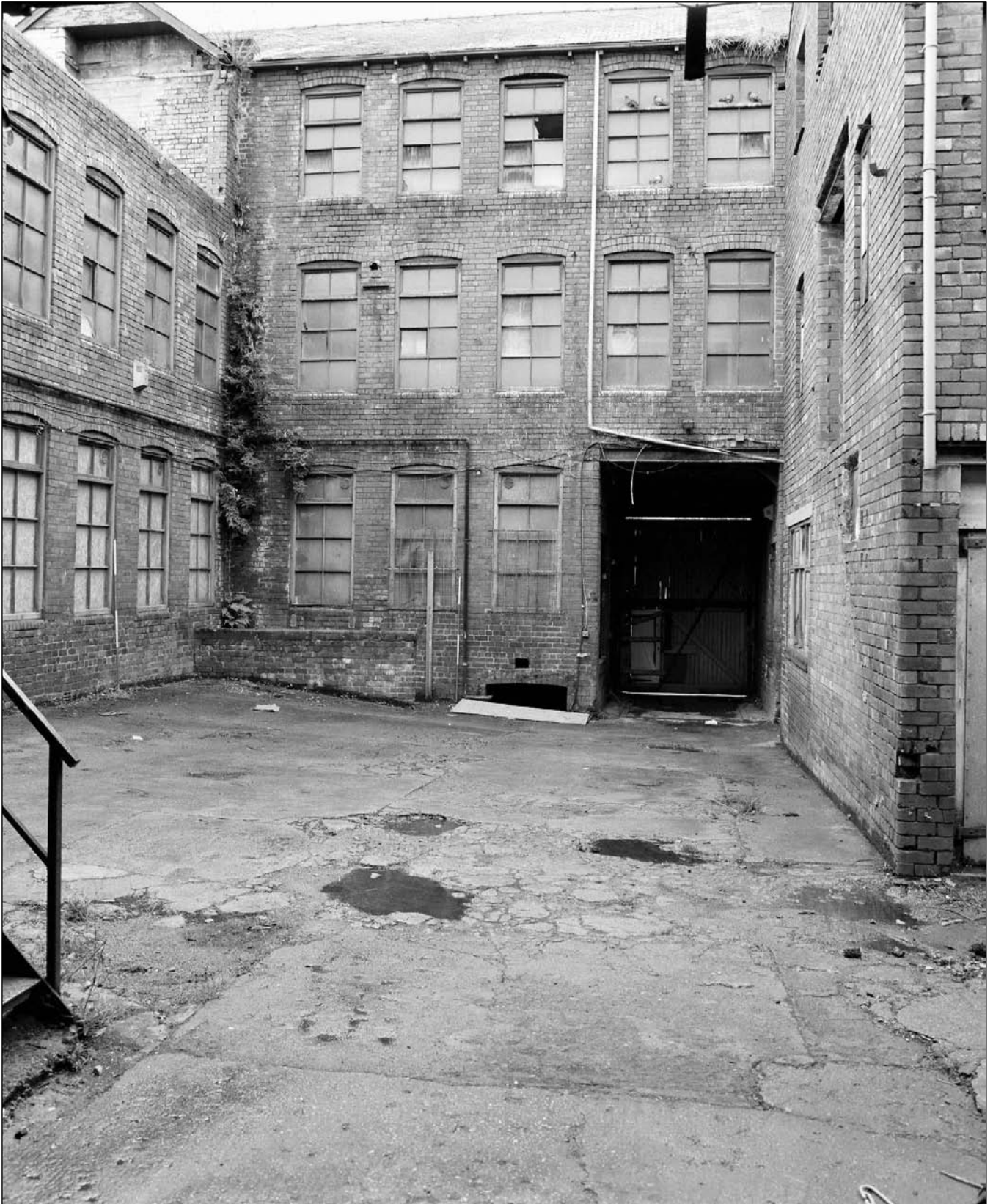
Plate 66: General view of the east elevation (south end) of the west range (film 10.5)
