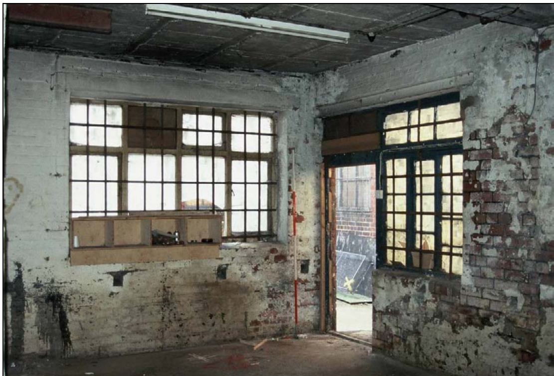
Plate 359: General view of southwest corner of G5, north range – note type 17 and 19 windows (film C/S 2.23)
