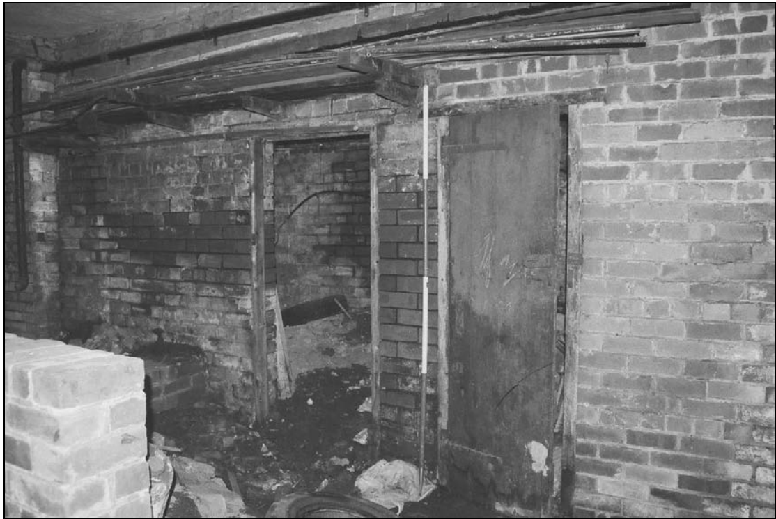
Plate 93: Detail of doors leading to B1 and B2, north wall of B3, west range (film 2.7)
