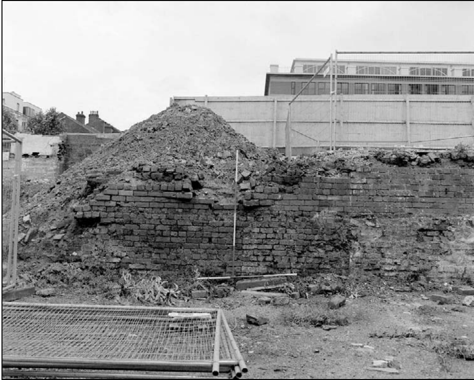
Plate 44: Detail of lower section of south elevation of south range (east end) (film 49.2)
