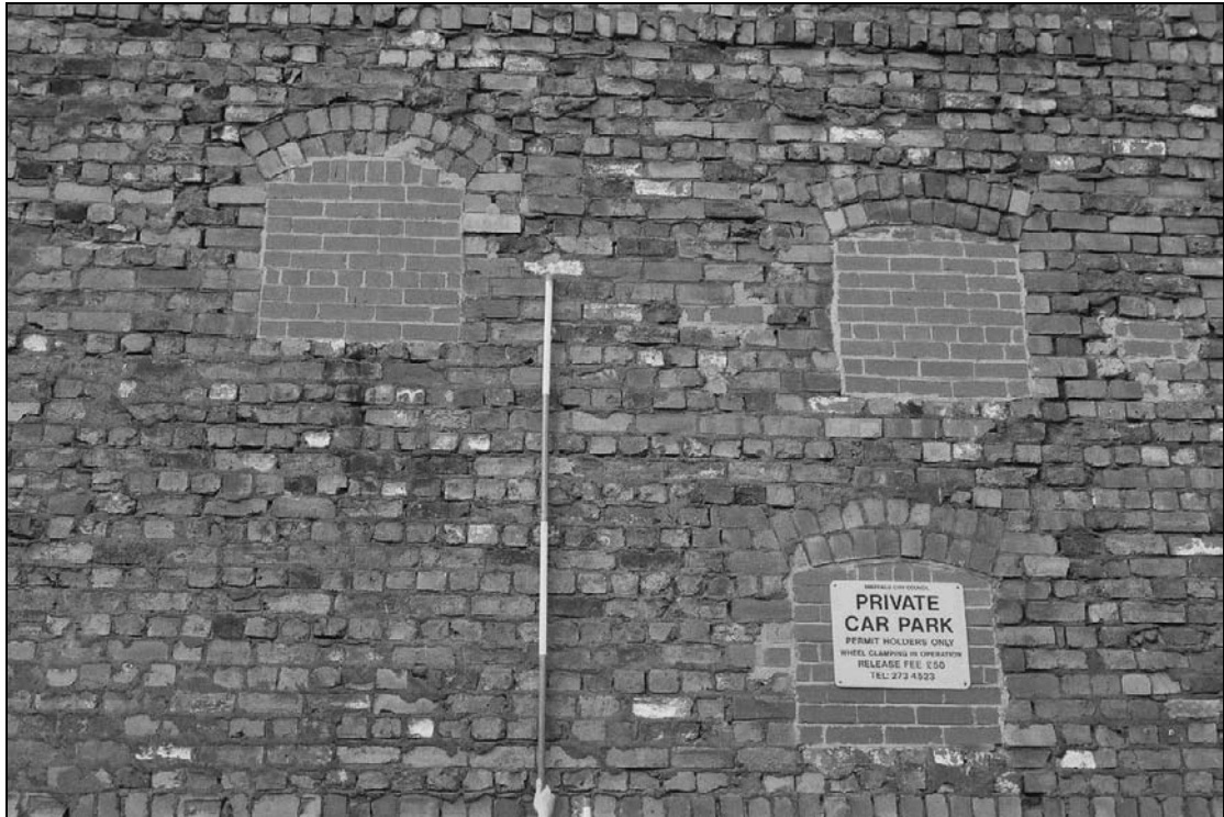
Plate 29: Detail of blocked primary openings, south elevation of south range (west end) (film 46.26)
