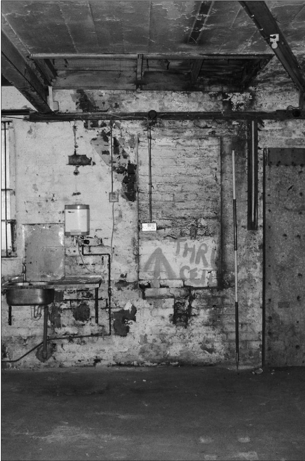
Plate 388: Detail of blocked window, stair scar and hatch in ceiling, west wall of F4, north range (film 24.32)
