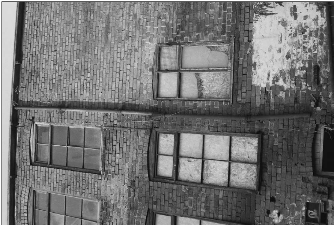
Plate 42: Detail of type 4 window and inserted window, south elevation of south range (film 46.19)
