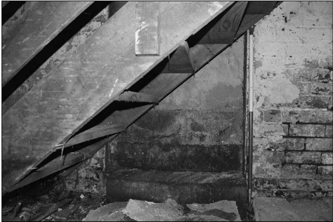
Plate 118: View of blocked doorway truncated by inserted stairs, in west wall of G3, originally leading to G2, west range (film 21.5)
