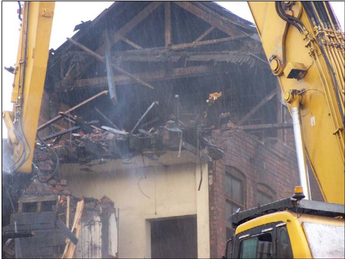
Plate 217: Detail of roof structure of king-post with diagonal braces, west range (film D.15)
