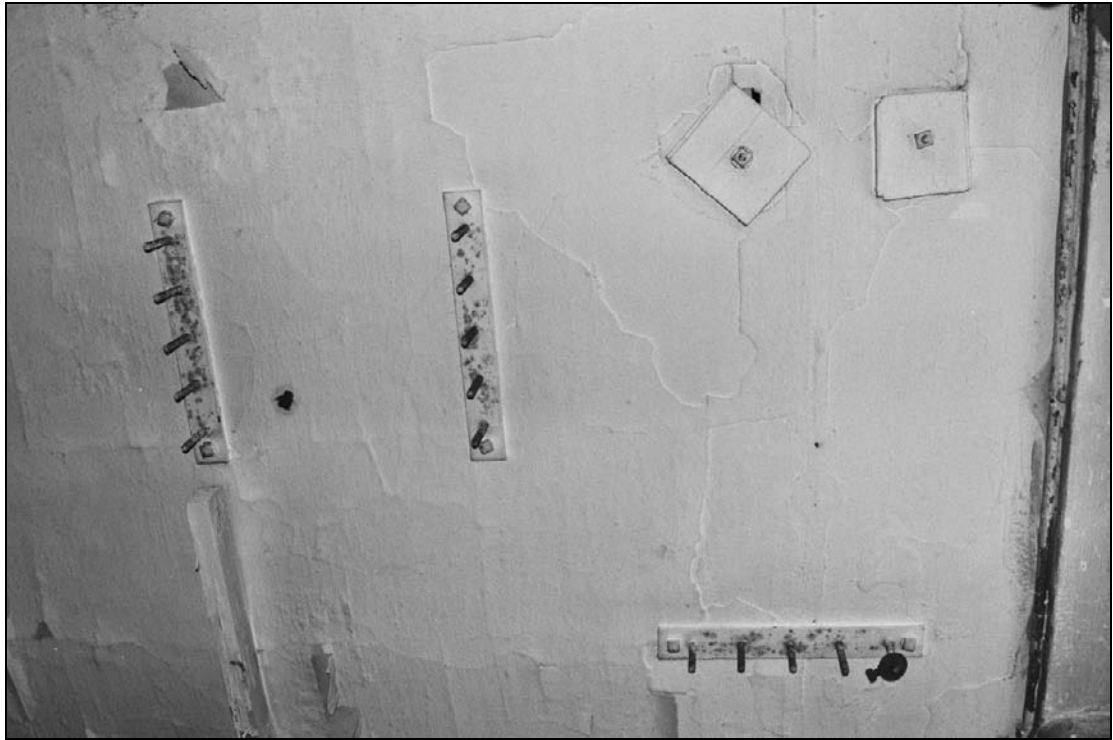
Plate 324: Detail of electrical fixings on the ceiling of G8, east range (film 21.21)
