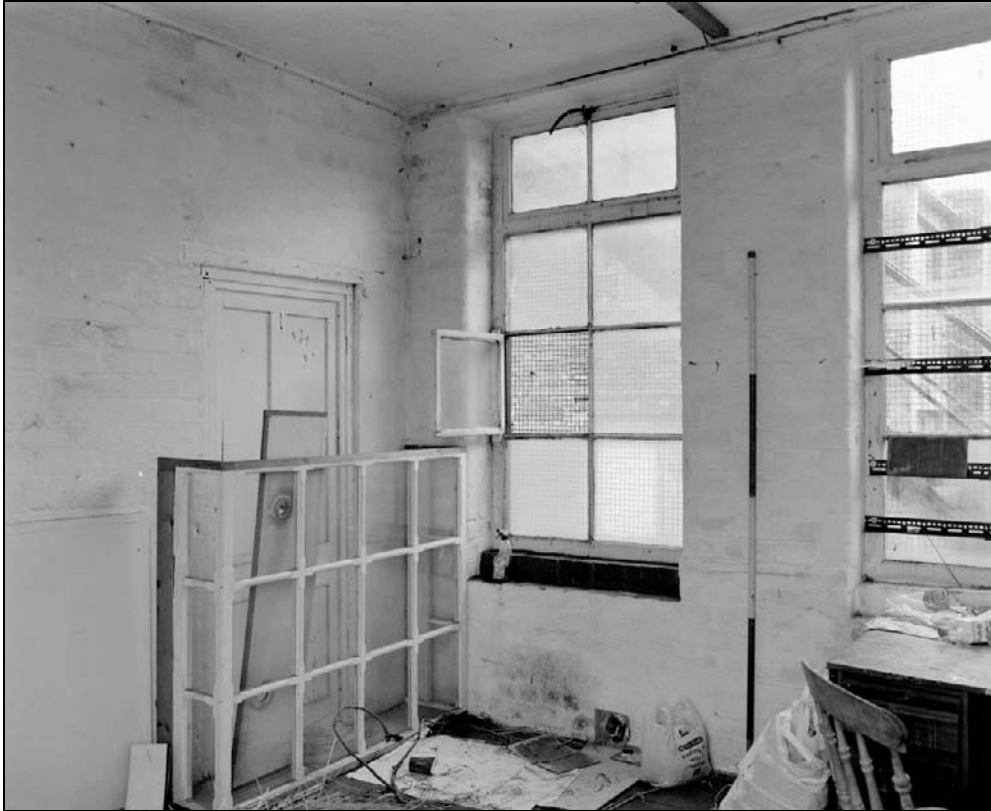
Plate 281: View of west end of F9, south range, showing doorway and type 4 window (film 34.3)
