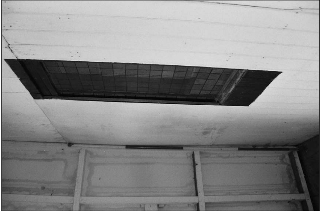
Plate 274: Detail of north side of timber and glazed partition, west end of F10 south range (film 25.6)
