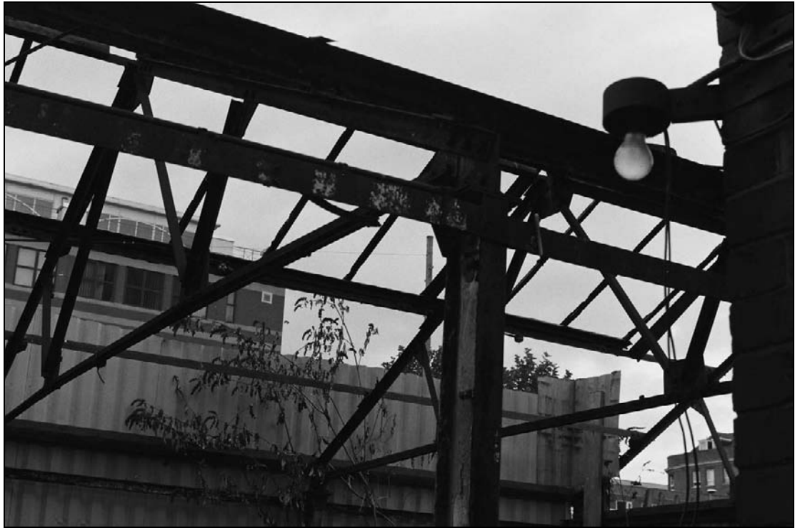
Plate 443: General view of bolted angle iron roof structure of G12, east building of furnace house (film 23.15)
