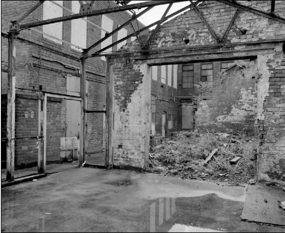
Plate 440: General view of G12, east building of furnace house range showing west wall (film 20.1)
