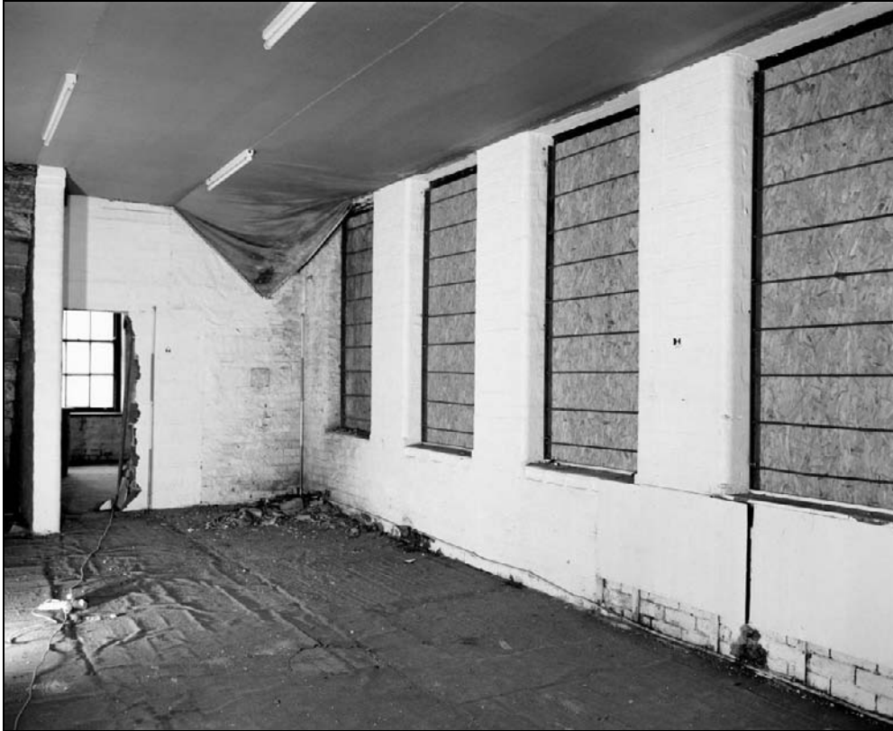
Plate 243: General view of room G20, south range – note partially blocked doorway leading to G21, west range (film 16.5)
