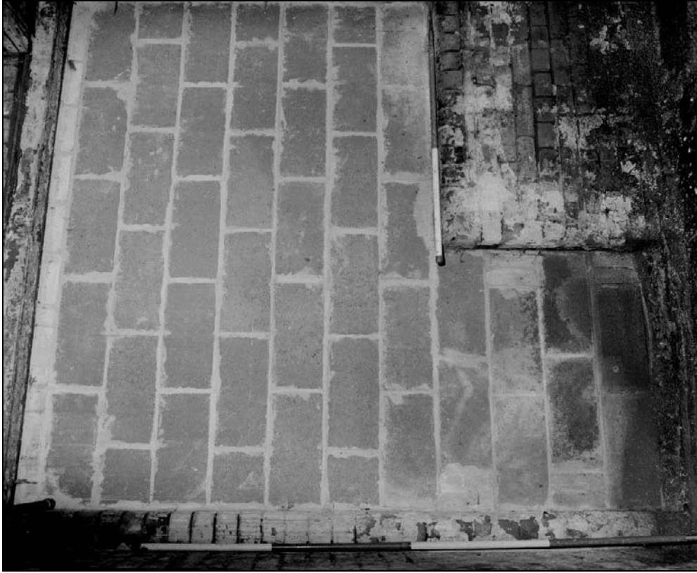
Plate 113: View of blocked entrance and window to G5, north range, east wall of G3 west range extension (film 14.2)
