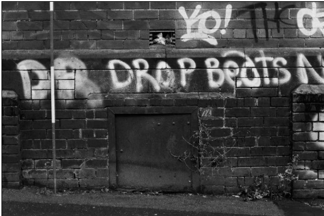
Plate 13: Detail of partially blocked and altered lightwell, west elevation of west range (film 1.19)
