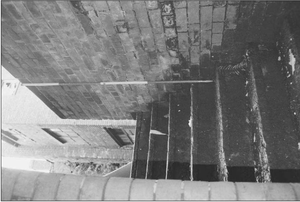
Plate 83: Detail of external stairs leading from basement (B3) to central yard (film 2.8)
