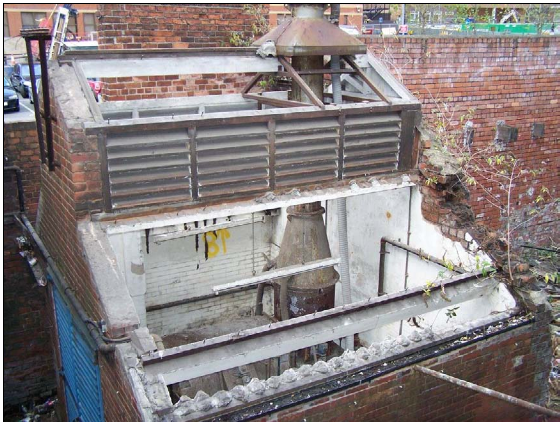
Plate 423: General view of G10 and G9, furnace house range, west building after removal of roof (film D.29)
