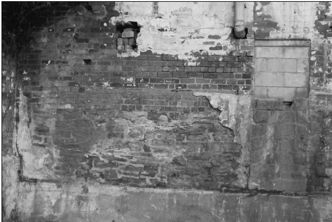
Plate 49: Detail of brick and stone walling of west elevation of machine shop (film 46.2)
