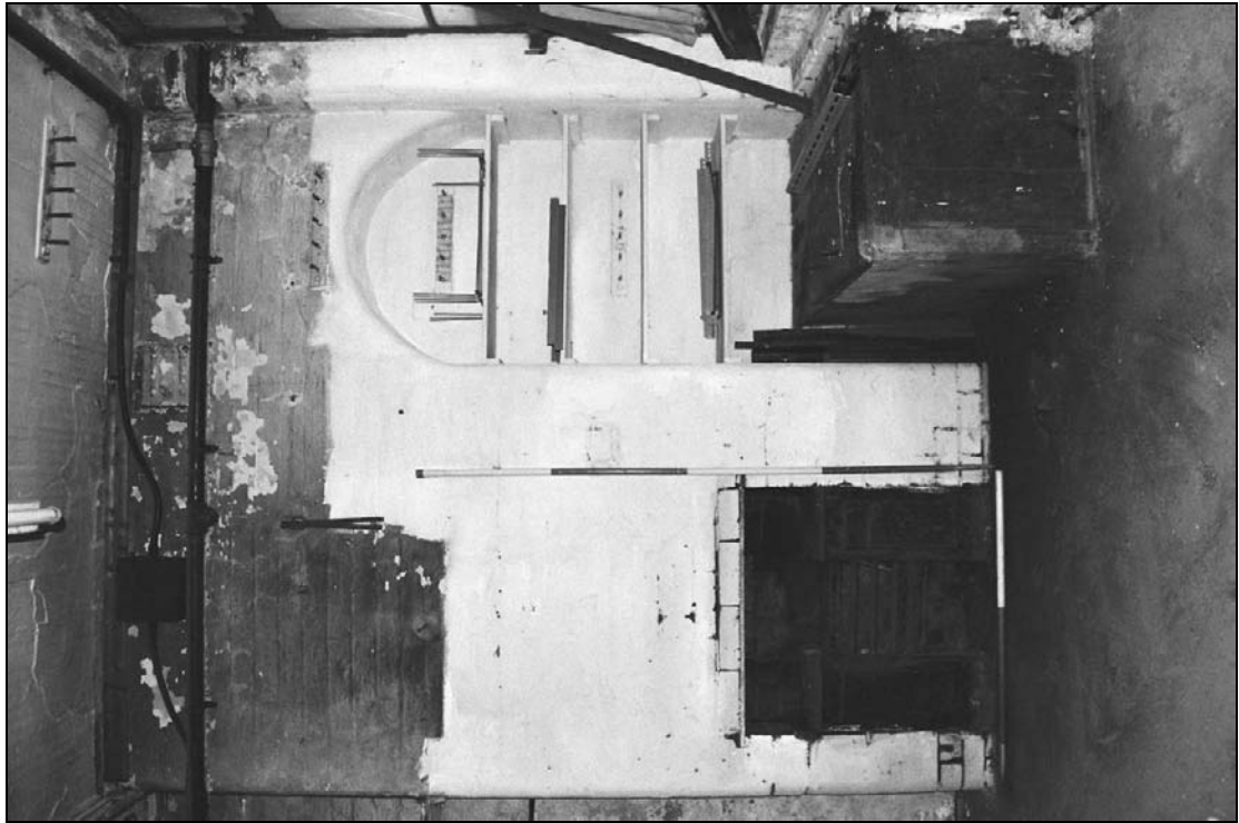
Plate 322: Detailed view of fireplace and adjacent arched alcove, G8 – note timber box over external staircase leading to basement (B7)(film 21.25)
