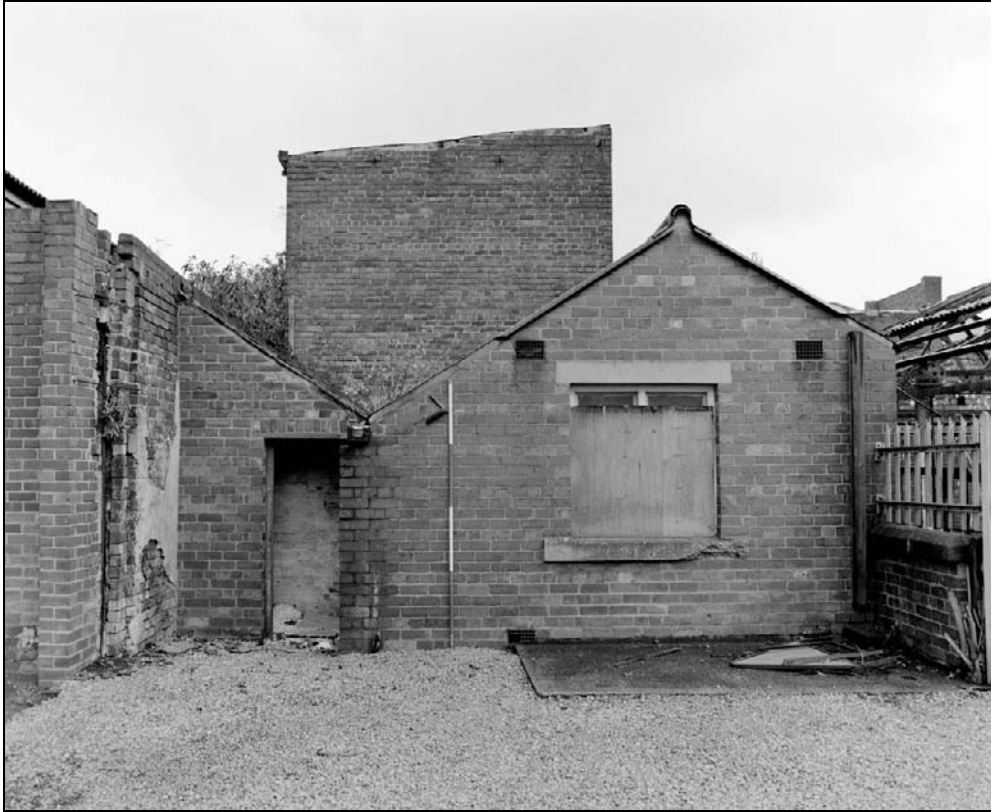
Plate 55: View of east elevation of wash house range, with south range beyond (film 5.10)
