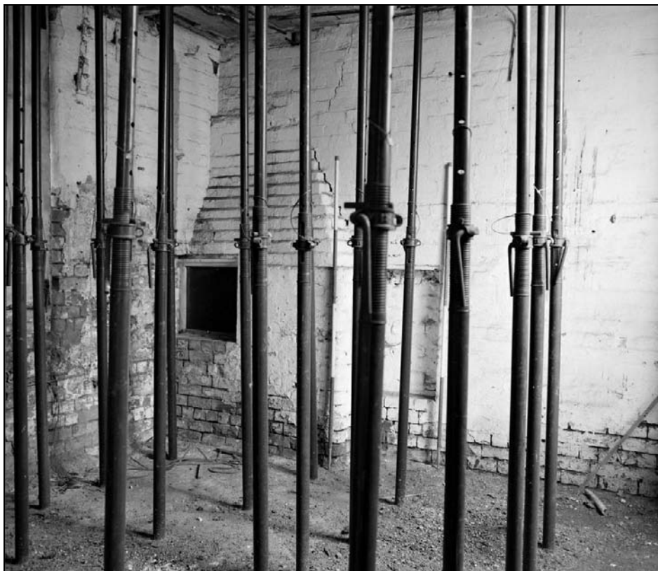
Plate 258: General view of room G17, south range – note remains of hand forge (film 18.1)
