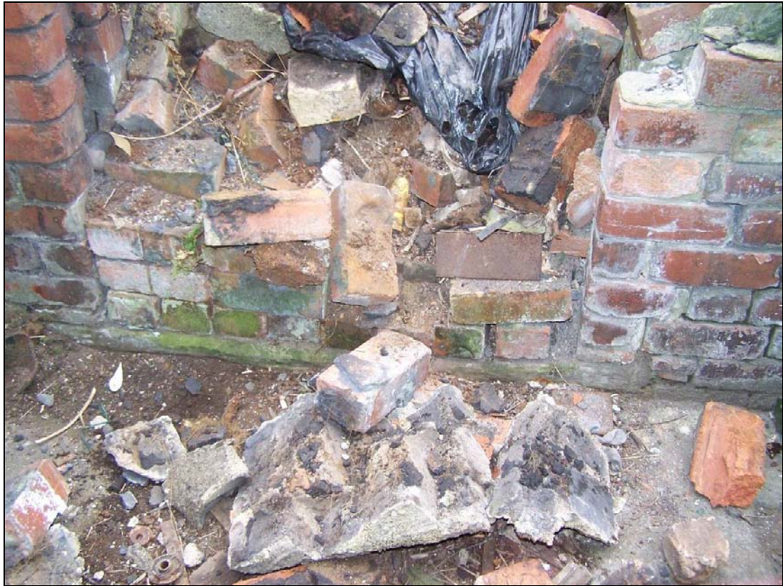
Plate 430: Detail of blocked door opening, south elevation of furnace house, G11, west end (film D.31)
