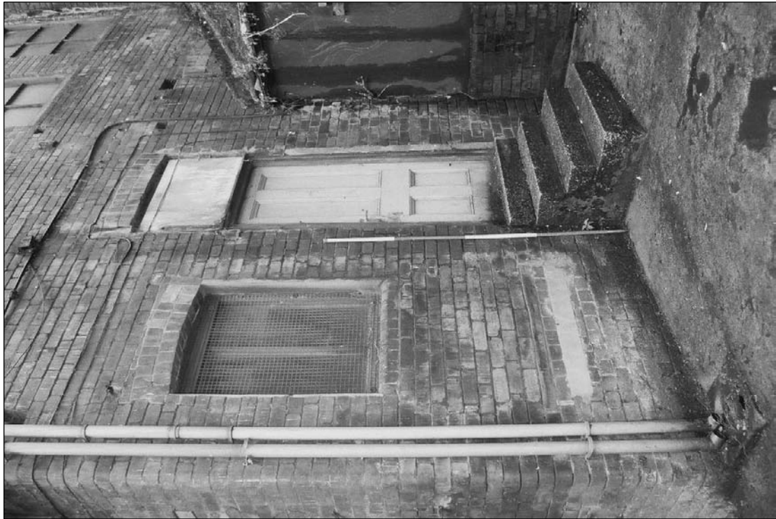
Plate 79: View of east elevation of west range (north end), showing doorway within former window and window within former doorway (film 2.31)
