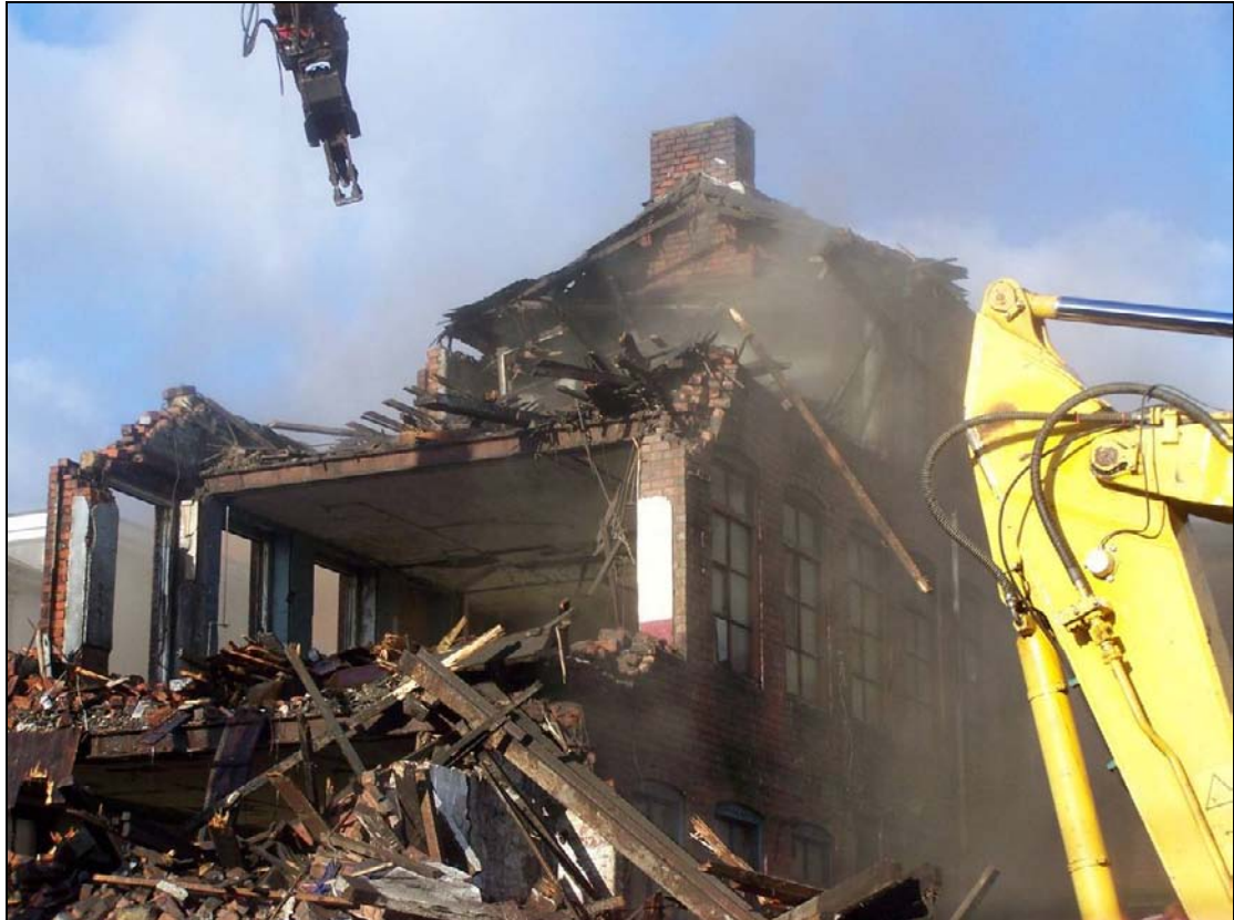
Plate 216: View of west range showing transverse steel I-section beams within which the timber joists were set (film D.14)
