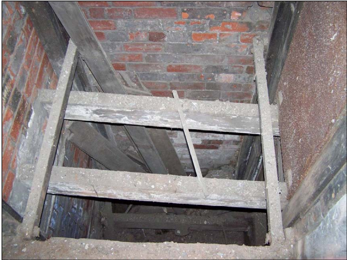
Plate 149: View of base of lift shaft with inserted timber platform and basement (B3) below (film D.7)
