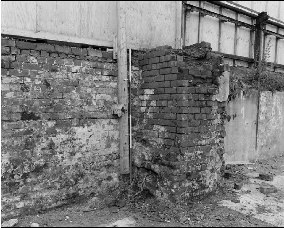
Plate 436: Detail of lower section of chimney stack, northeast corner of furnace house – note blocked arched opening (film 51.6)
