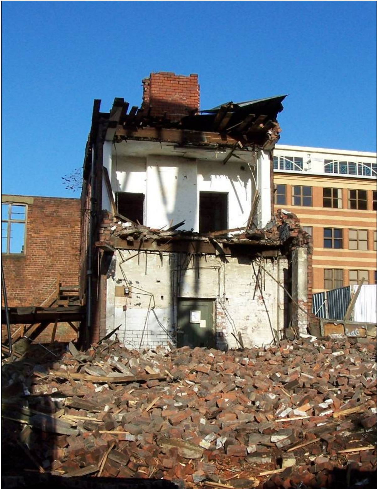
Plate 339: General view of east range during demolition showing floor and ceiling construction (film D.25)
