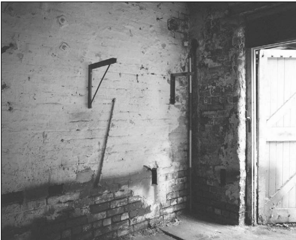
Plate 369: Detail of northeast corner of G6 showing former position of hand forge – note flue in east wall (film 43.5)
