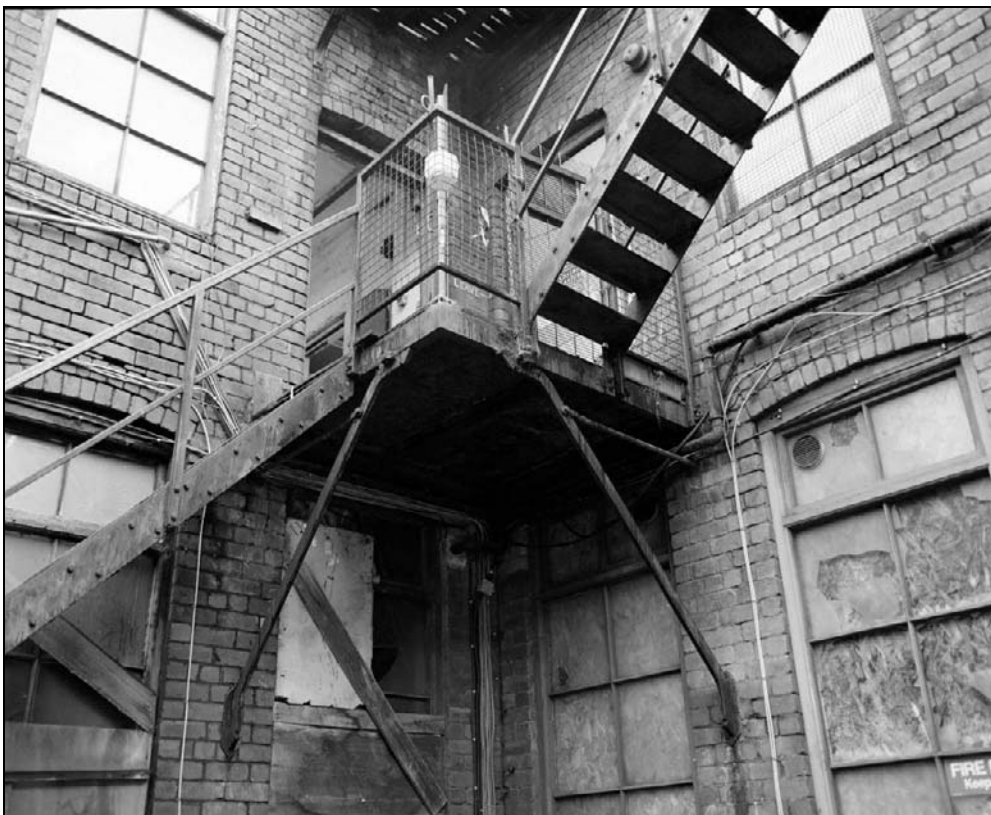
Plate 313: Detail of external staircase and cast iron brackets, west elevation, south end of east range (film 43.10)
