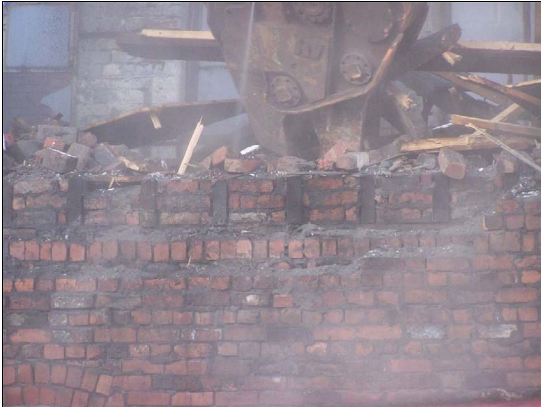
Plate 310: Detail of timber floor joists set into south wall of south range (film D.20)
