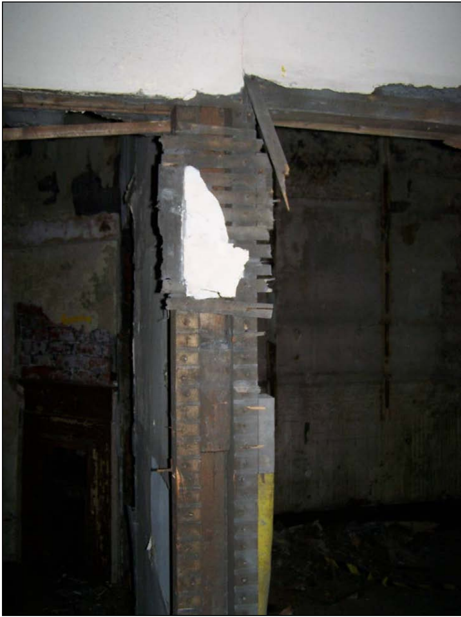
Plate 168: Detail of partition construction with lath and plaster covering, north wall of F1 (film D.10)
