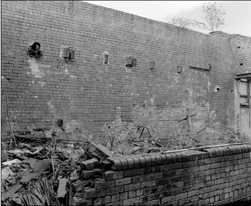
Plate 426: General view of central building/furnace house – showing truncated roof trusses in north wall and chimney stack in northeast corner (film 10.10)
