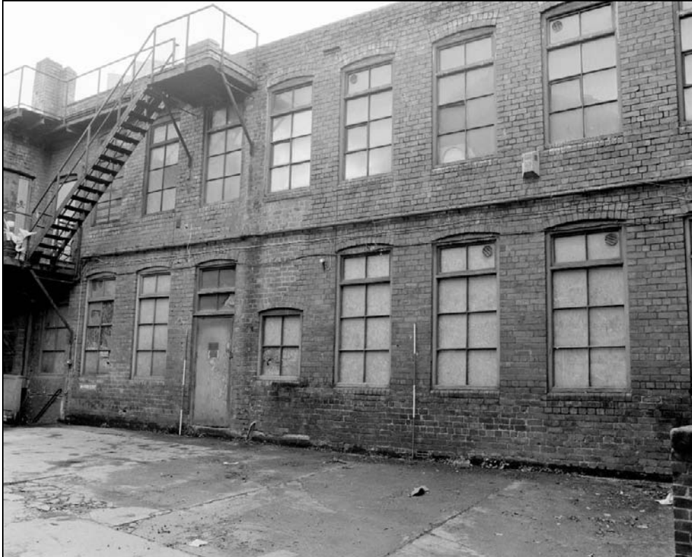
Plate 219: General view of north elevation of the south range (west end) (film 9.3)
