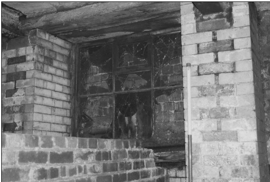
Plate 87: Detail of blocked lightwell, B3, west range (film 2.2)
