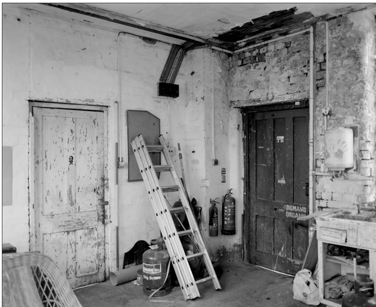
Plate 328: General view of southwest corner of F6, east range, showing doorways leading to F9, south range and the external staircase from the central yard – note brick flue (film 35.10)
