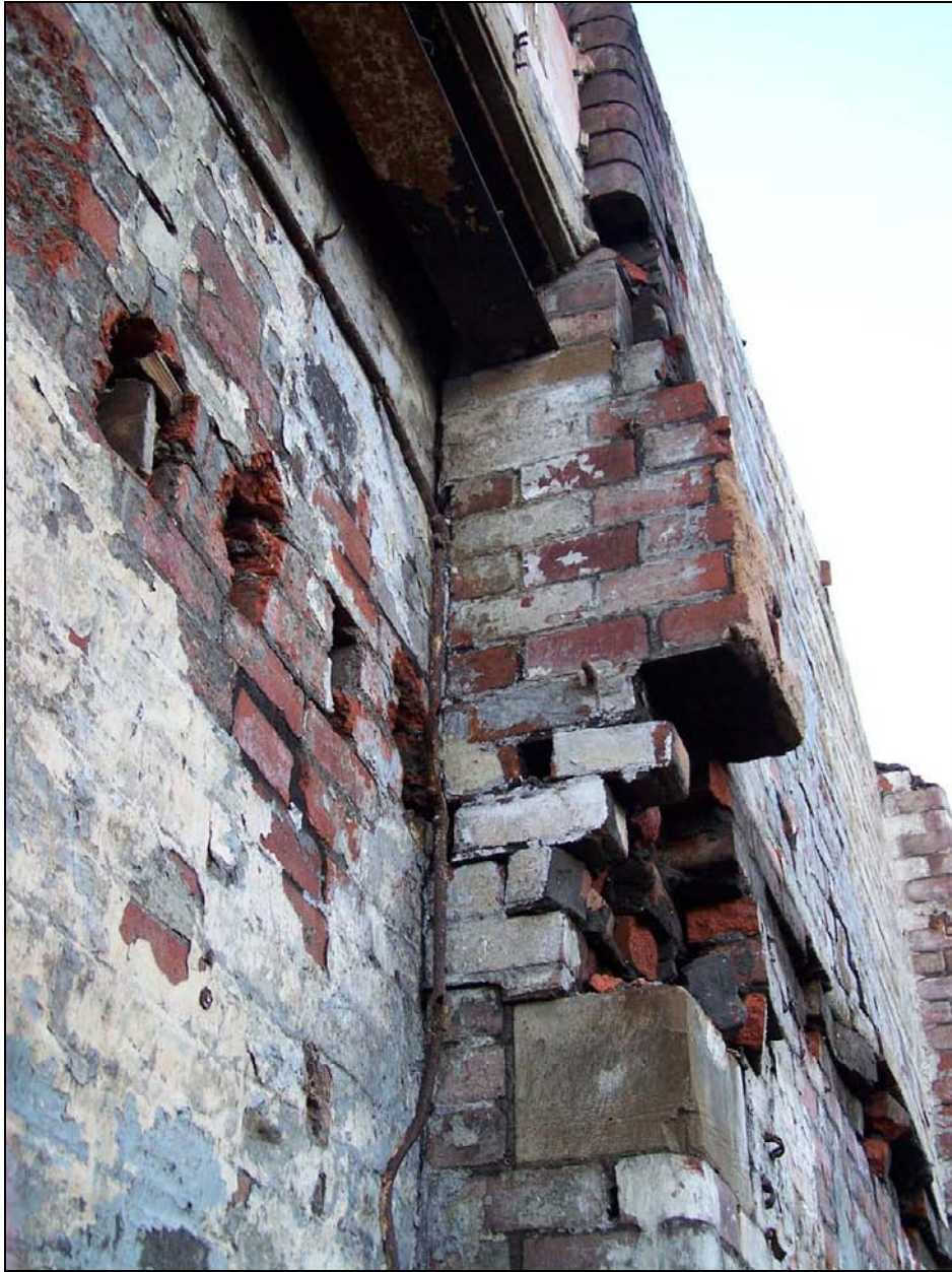
Plate 391: Detail of bull nosed brick jamb, north wall of former F4 – also note modern brickwork below (film D. 26)
