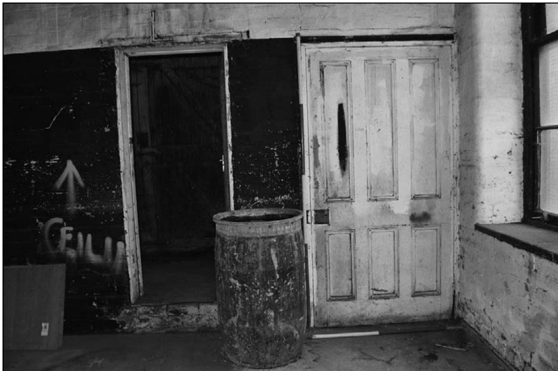
Plate 127: Detail of stair doorway and adjacent timber panelled lift door, south wall of G21, west range (film 3.14)
