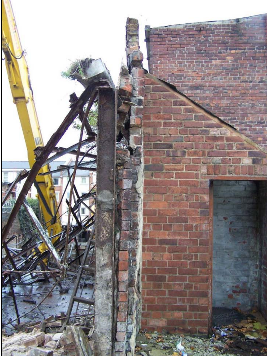
Plate 416: View showing detail of steel structure of machine shop and relationship with earlier privy block to the north (right) (film D.28)
