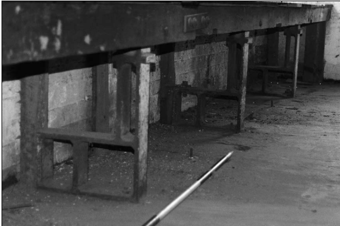
Plate 386: Detail of line shafting supports of workbench along east wall of F4, north range (film 24.25)
