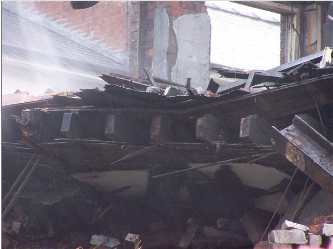
Plate 215: Detail of timber floor joists, boarding and lath and plaster construction, west range (film D.13)
