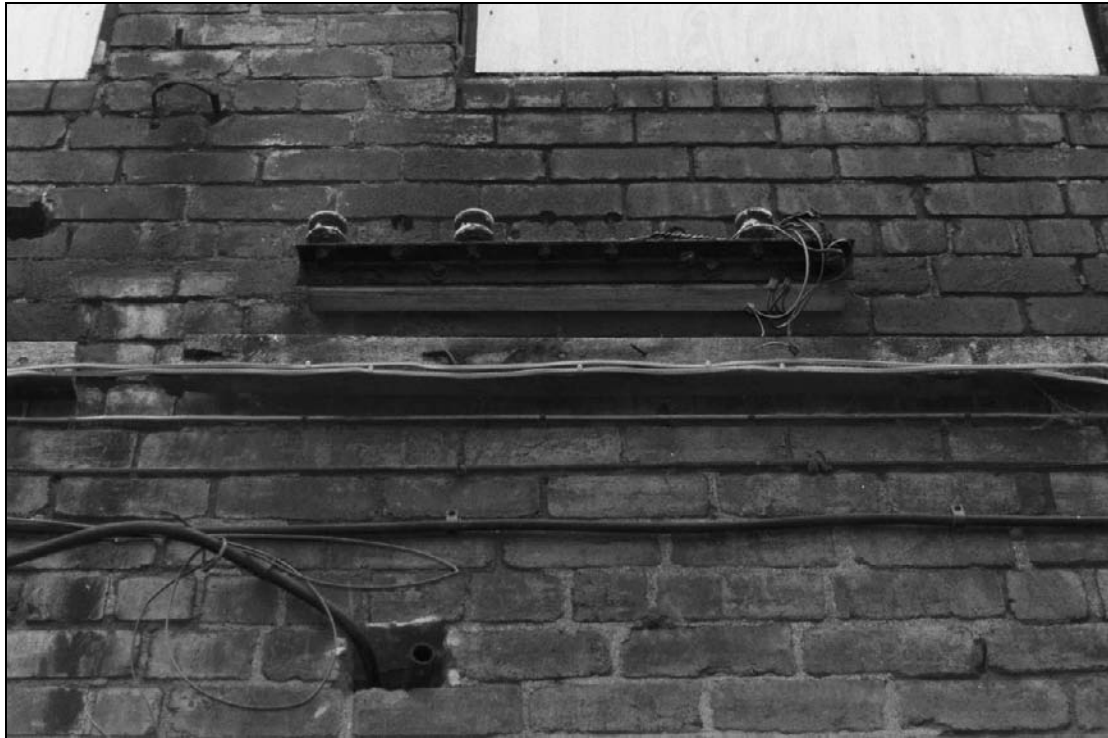
Plate 228: Detail of electrical transformers positioned on the north elevation of the south range (east end) (film 23.1)
