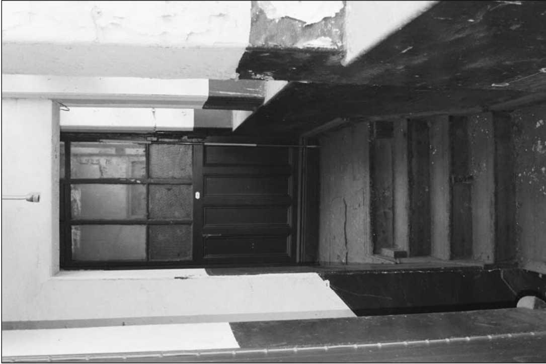
Plate 152: View of north end of F18 showing paneled partition and top of staircase (film 25.21)
