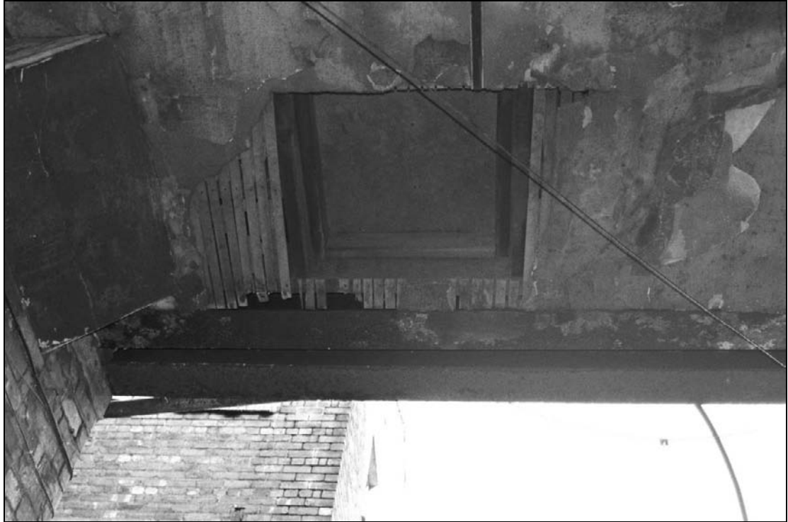
Plate 78: Detail of inserted overhead hatch within ceiling of cart passage, west range (film 27.7)
