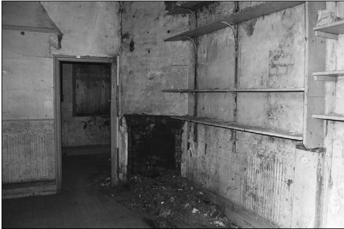
Plate 174: General view of F3 showing doorway to F2 and shelving along north wall (film 24.10)
