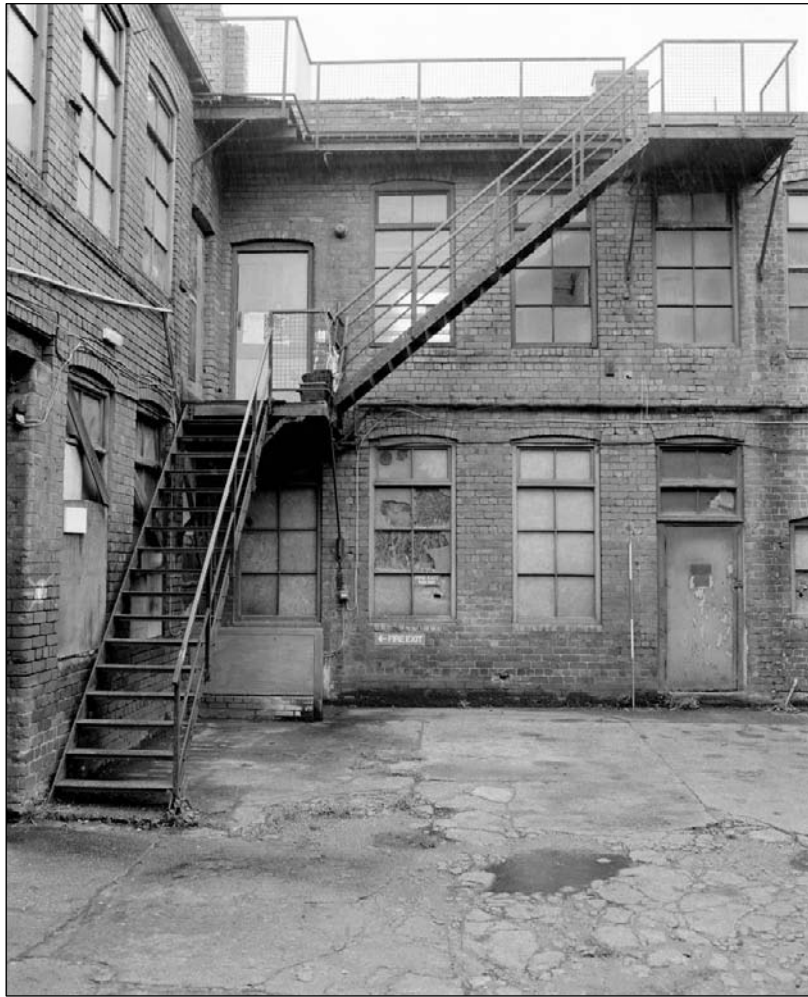
Plate 223: View of north elevation of south range (west end) showing join with east range – note external staircase (film 10.1)
