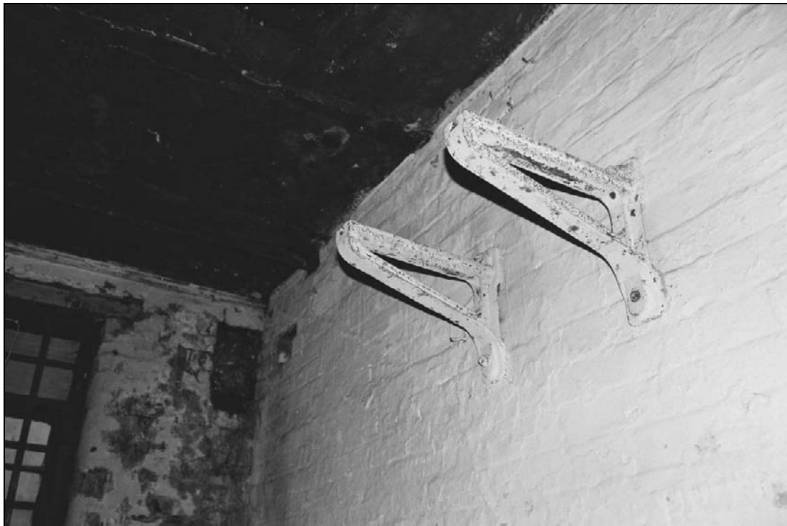
Plate 365: Detail of cast iron brackets, south wall of G5, north range (film 21.15)
