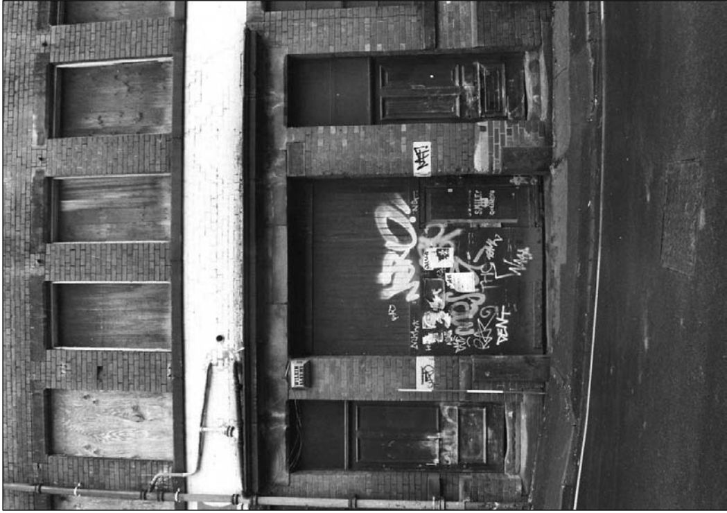
Plate 7: Detail of cart passage and flanking pedestrian doors, west elevation of west range (film 1.28)
