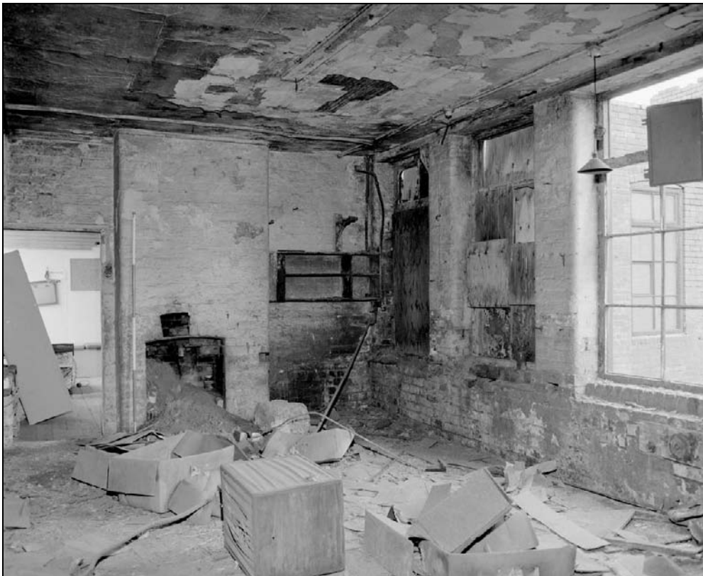
Plate 291: General view of F7, south range (east end) – note fireplace and shelving (film 35.2)
