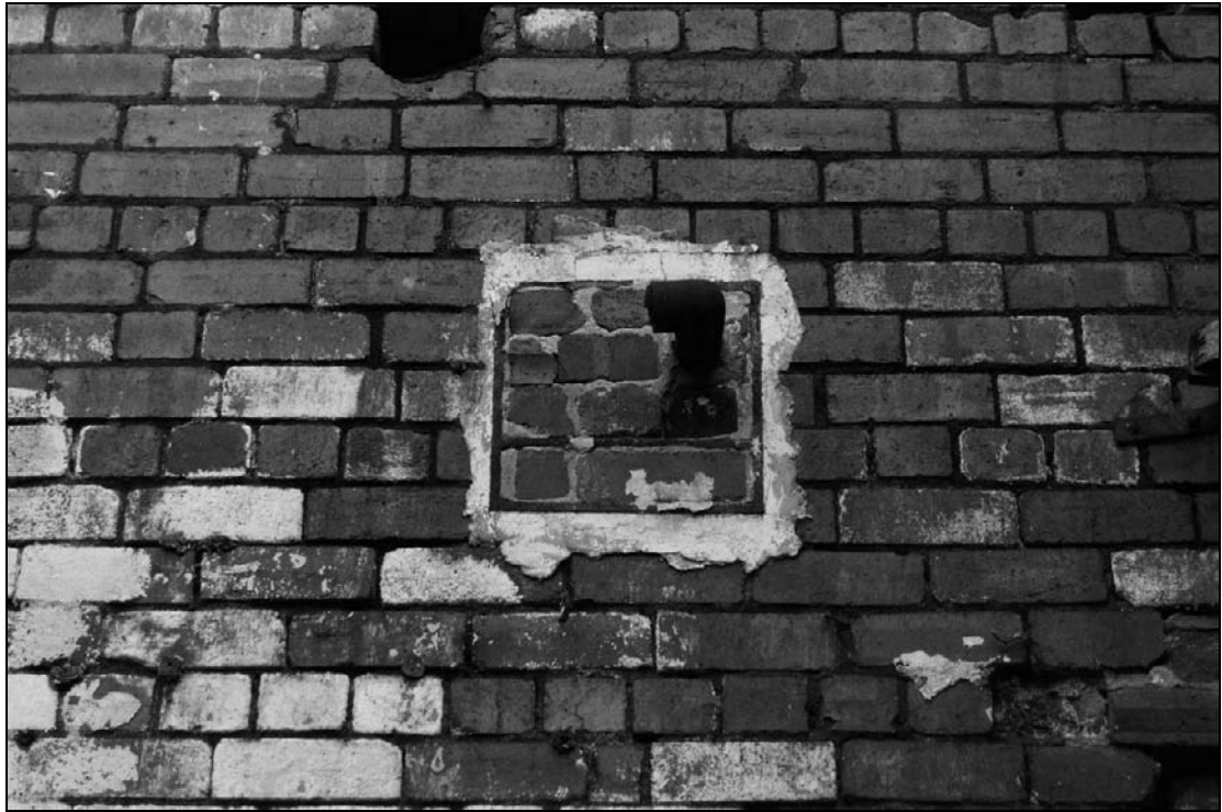
Plate 428: Detail of blocked wall box, west wall of G11, furnace house (film 23.9)
