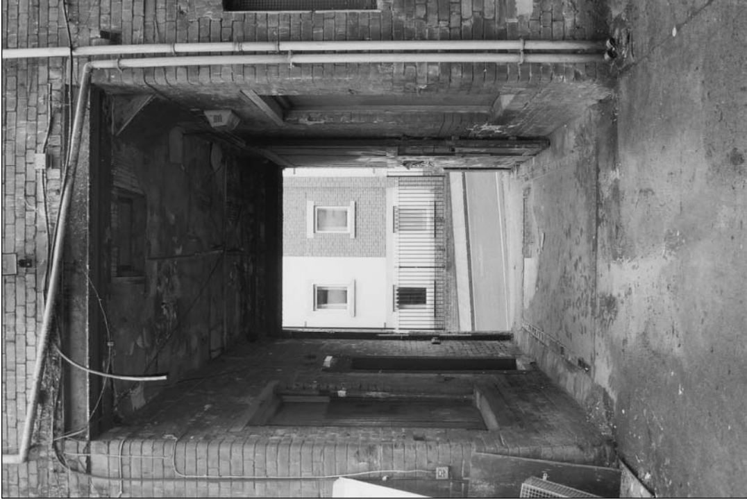
Plate 74: Detail of cart passage with gate open, east elevation of west range (film 2.34)
