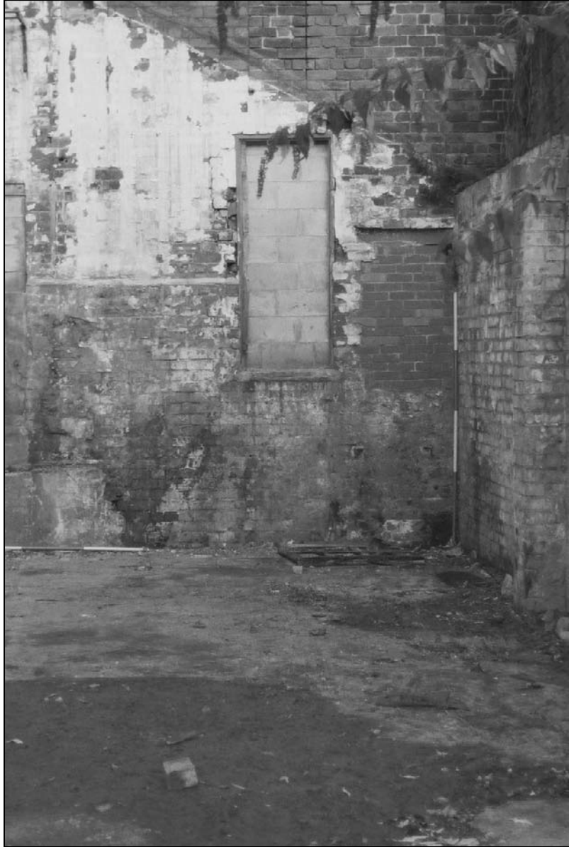
Plate 50: Detail of blocked door and adjacent blocking, west elevation of machine shop (film 46.5)
