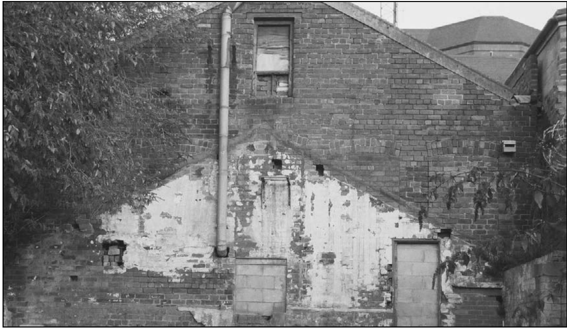
Plate 51: Detail of blocked primary windows and later roof scar, west elevation of machine shop (film 46.7)
