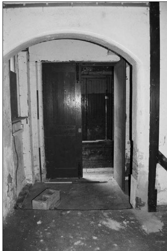
Plate 104: View of archway with loading door beyond leading to cart passage, room G2, west range (film 22.35)
