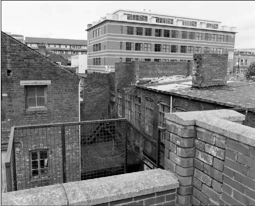
Plate 315: View of west elevation of east range showing removed second floor and projecting truncated chimney breast with blocked fireplace (film 12.7)
