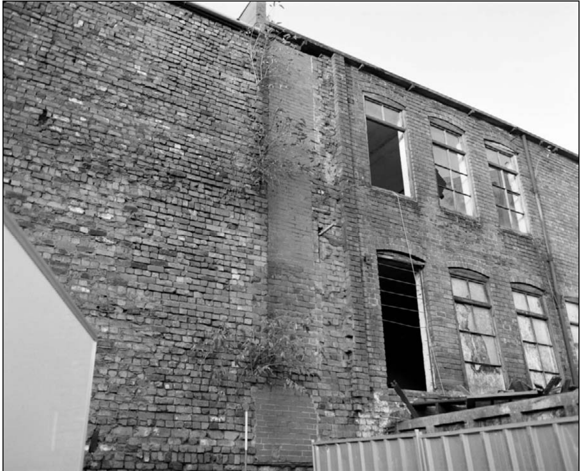
Plate 31: View of possible blocked power transmission shaft and projecting bricks denoting the eastern extent of the formerly adjacent Trafalgar Grinding Wheel and extensions, south elevation of the south range (film 48.1)
