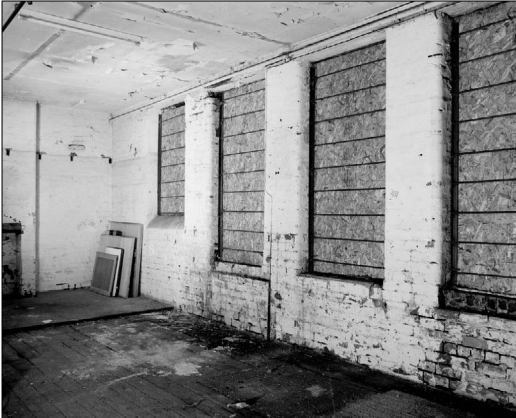
Plate 248: General view of G19, south range – note inserted window and raised floor level with sockets in east wall from former partitioned room with suspended ceiling (film 16.7)
