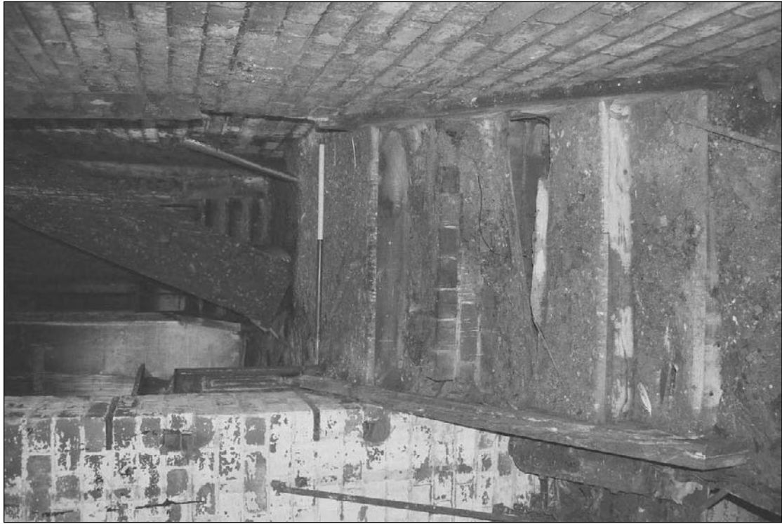
Plate 404: Detail of timber stairs leading to/from S4, northwest corner of S5 (film 44.23)
