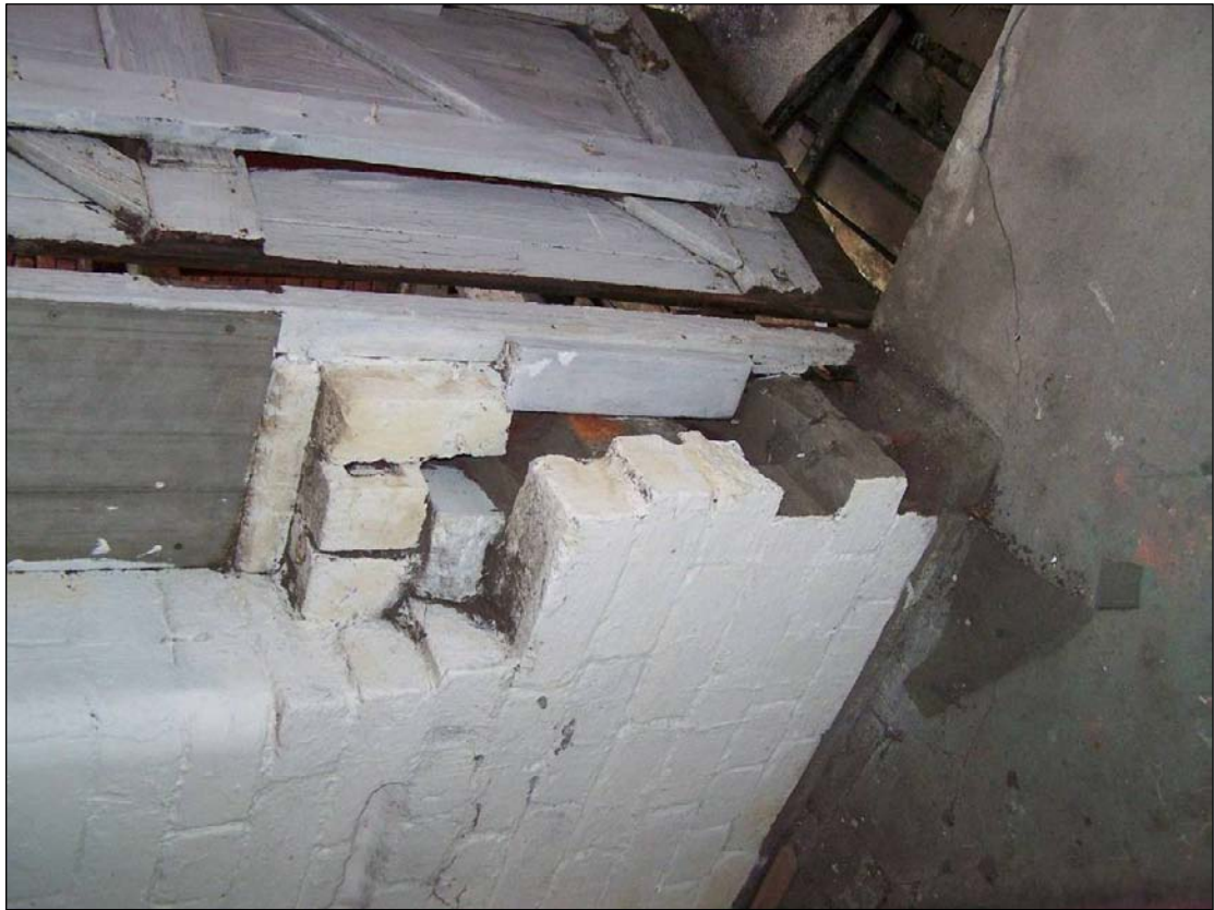
Plate 337: Detail of inserted doorway within former type 4 window, leading to secondary external staircase, F5, east range (film D.23)
