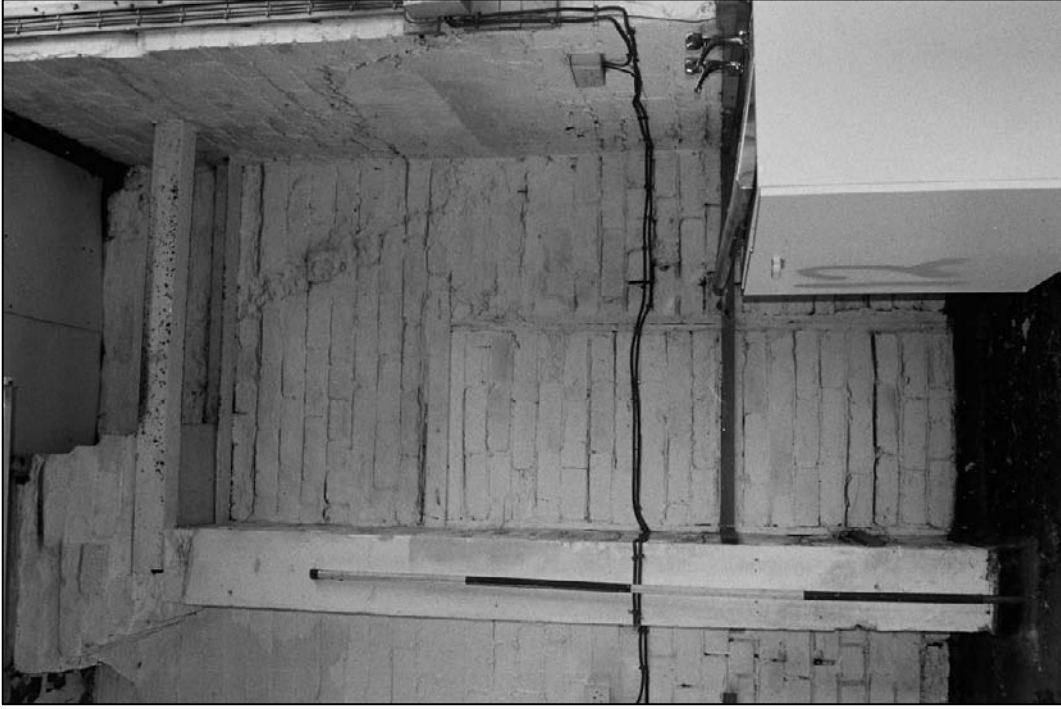
Plate 256: View of northwest corner of G18 showing scars from removed hand forge and inserted doorway (film 22.15)
