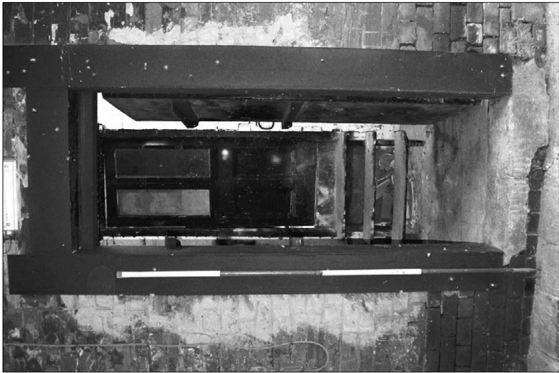
Plate 77: Detail of inserted door within former window, south side of cart passage, west range (film 27.9)
