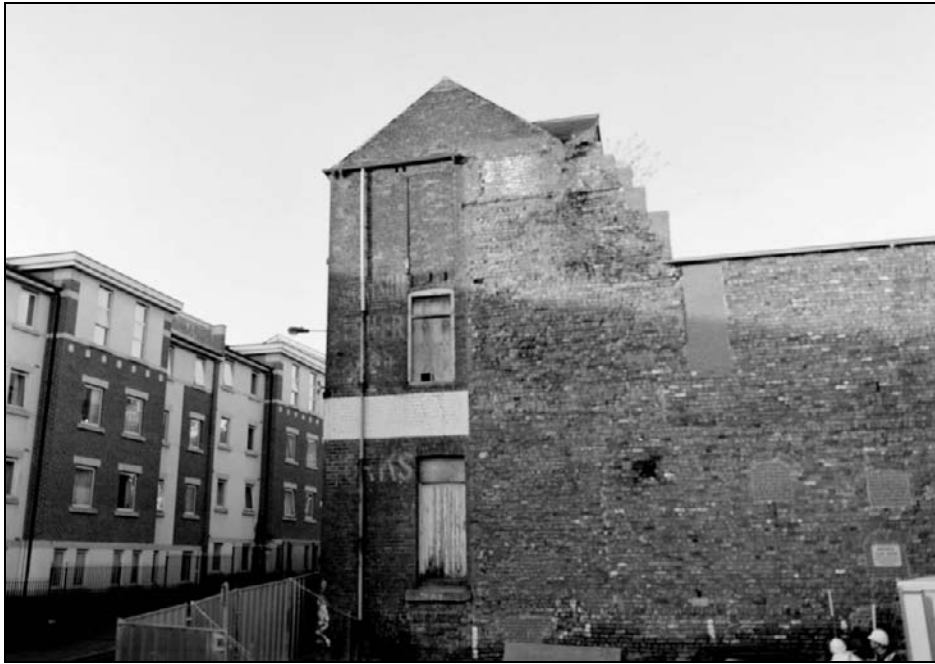
Plate 19: View of south elevation of the west range and west end of the south range (film 47.3)
