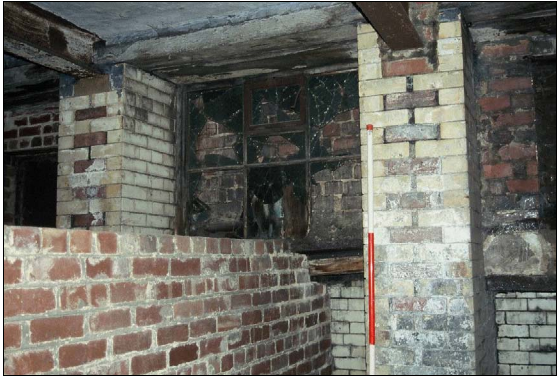
Plate 88: Detail of blocked lightwell, B3, west range – note also light reflecting brick work (film C/S 2.27)
