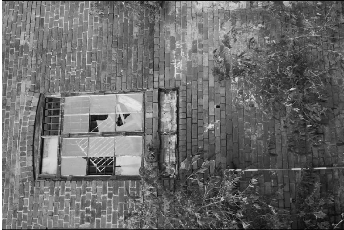
Plate 43: Detail of type 9 window with raised sill, south elevation of south range (east end) (film 46.12)
