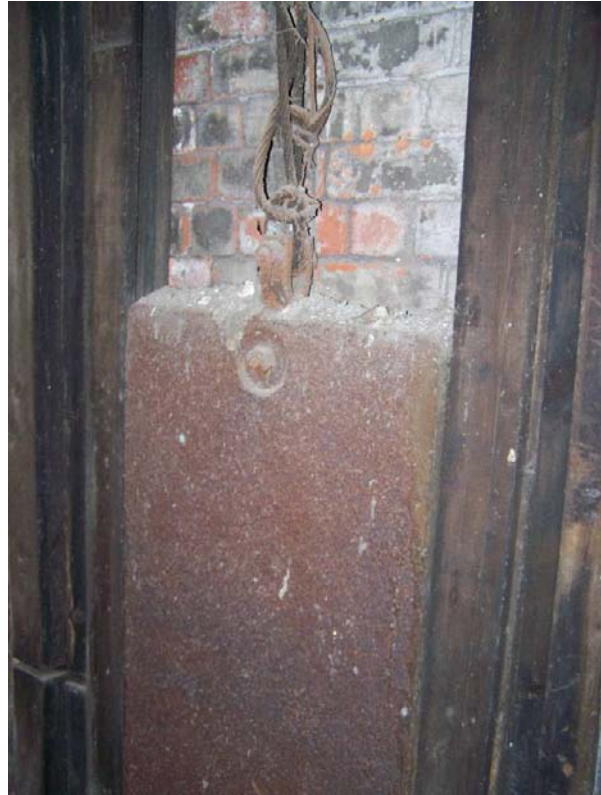
Plate 150: Detail of lift counterweight (film D.8)
