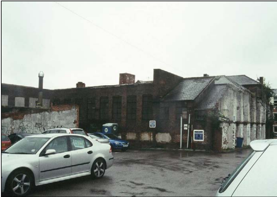
Plate 63: General view of the east and north elevation of the east range (film C/S 2.31)
