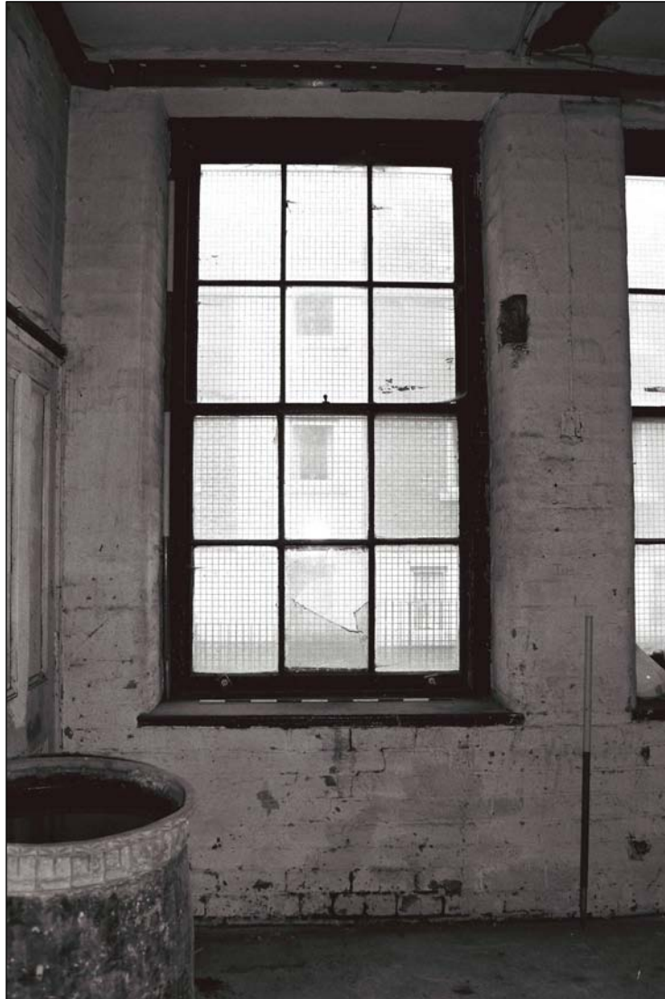
Plate 125: Detail of type 1 window, west wall of room G21, west range (film 3.12)
