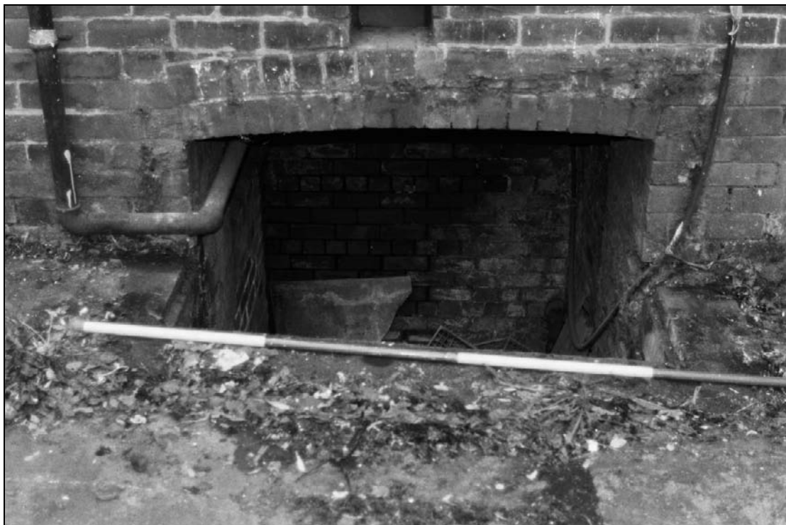
Plate 70: Detail of lightwell into B2, east elevation of west range (south end) (film 27.11)
