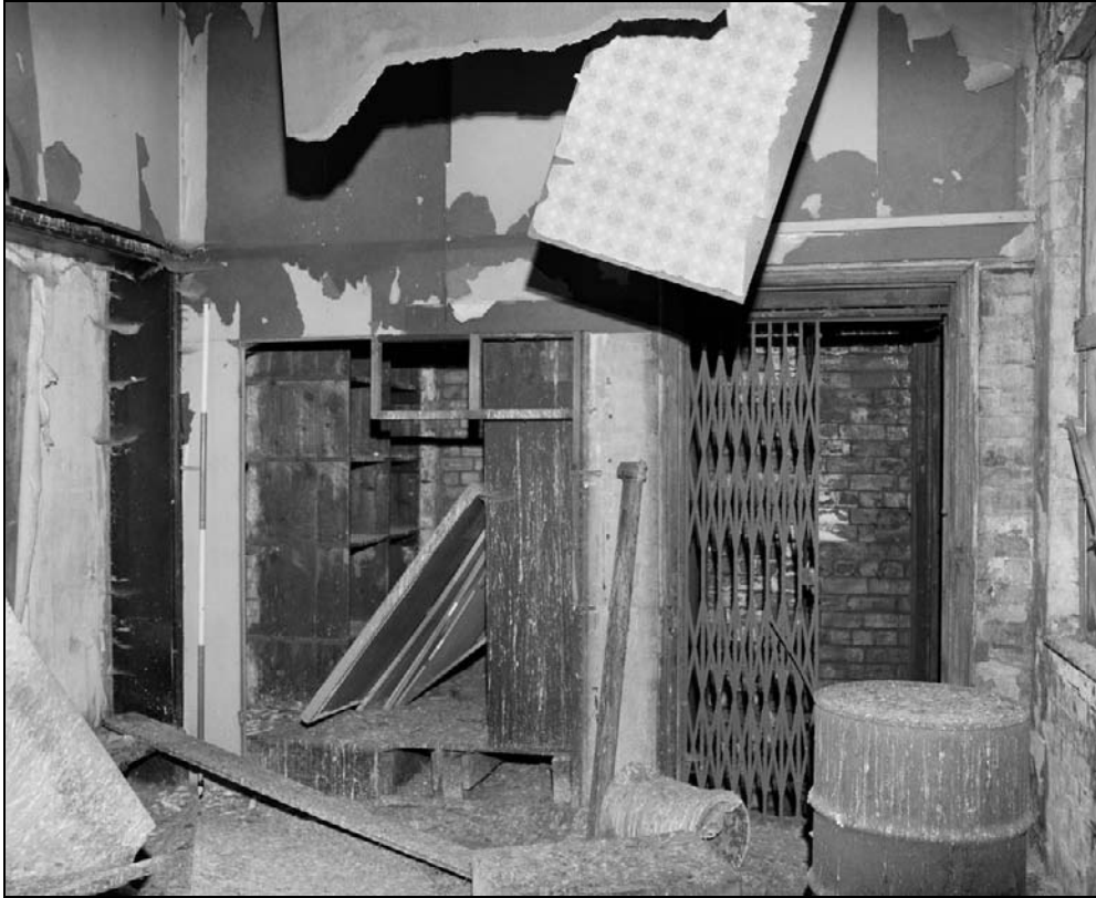
Plate 187: View of lift shaft and storage area at south end of S1 (film 37.6)
