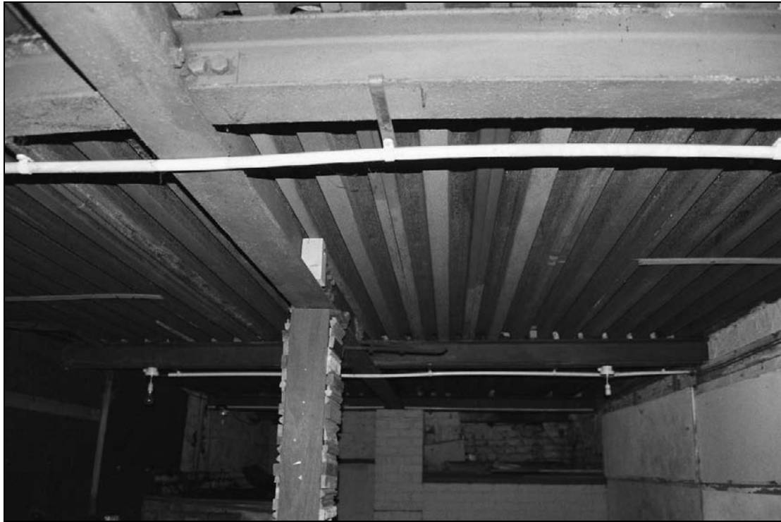
Plate 235: Detail view of inserted ceiling (air raid shelter) of B5 (south range) (film 3.28)
