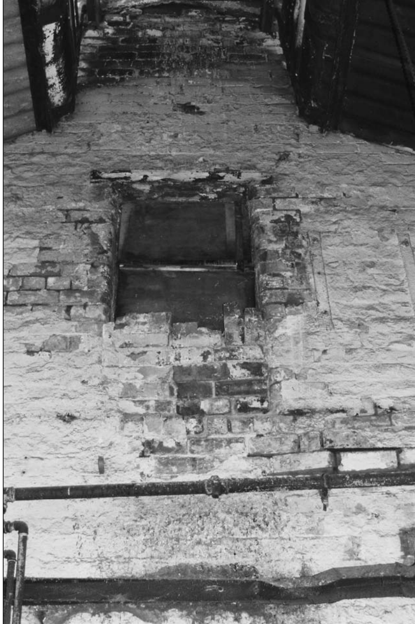
Plate 411: Detail of boarded primary window in gable of west wall, G15, machine shop (film 23.29)
