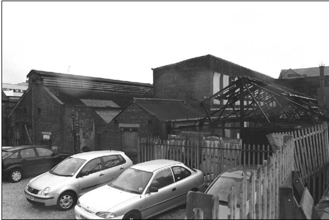
Plate 57: General view of the east elevation of the machine shop, wash house and furnace house ranges, with the south range beyond (film 1.7)
