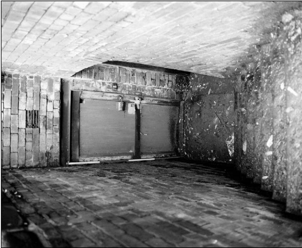
Plate 82: Detail of external yard leading to basement, west range, from central yard (south range ahead, west range to right) (film 6.2)
