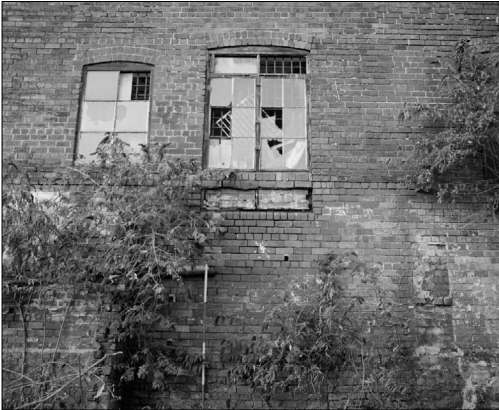
Plate 40: Detail of type 8 and 9 windows, south elevation of south range (east end) (film 48.6)
