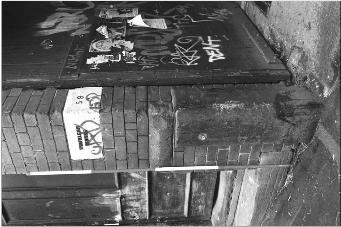
Plate 10: Detail of corner iron plate, cart passage, west elevation of west range (film 1.24)
