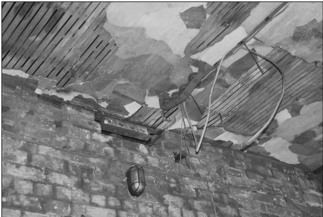
Plate 319: Detail of lath and plaster ceiling of east range cart passage and attached electrical transformers (film 2.18)
