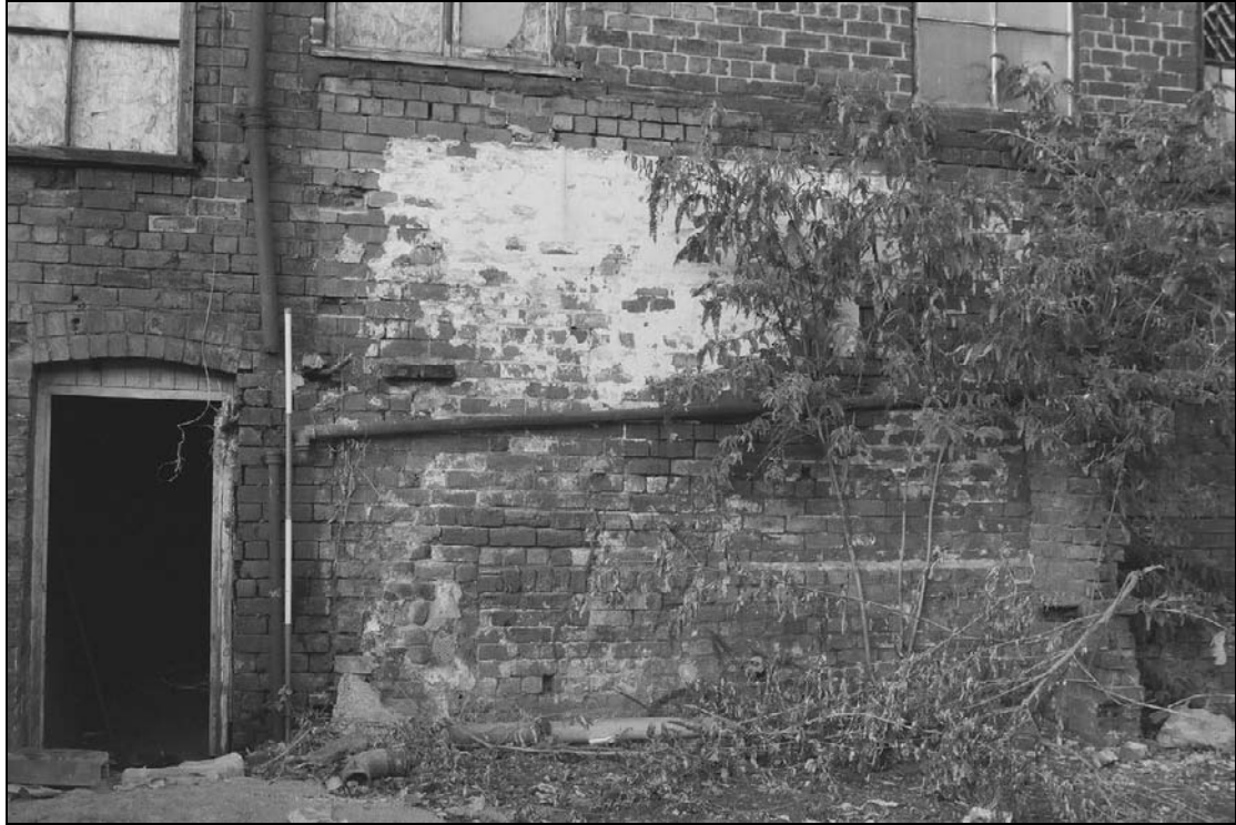
Plate 36: Detail of changes in brickwork, including blockings, paint remains and abut walls of former structures, south elevation of south range (east end) (film 46.15)
