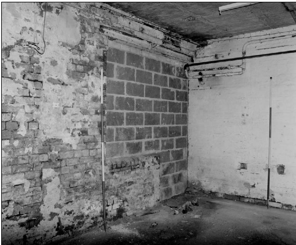
Plate 361: Detail of blocked doorway and type 19/20 window, west wall of G5 (film 15.1)
