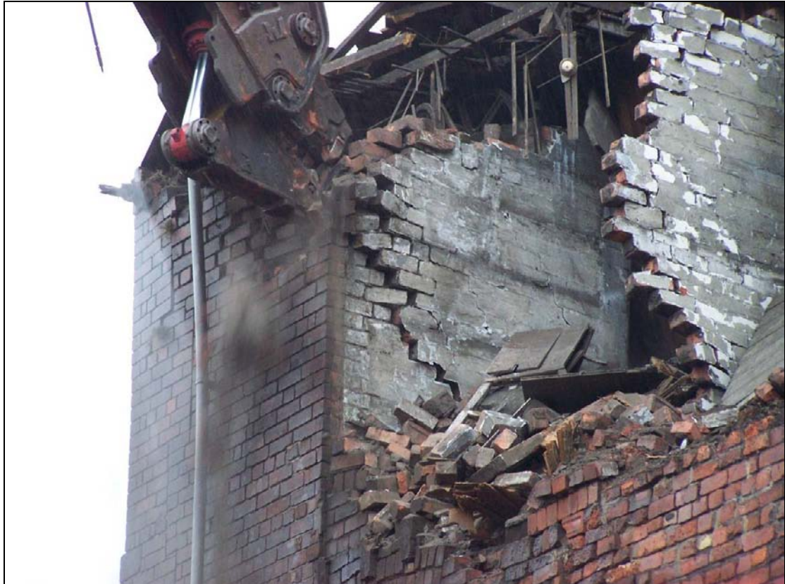
Plate 214: Detail view of original east wall of lift shaft, west range (film D.12)
