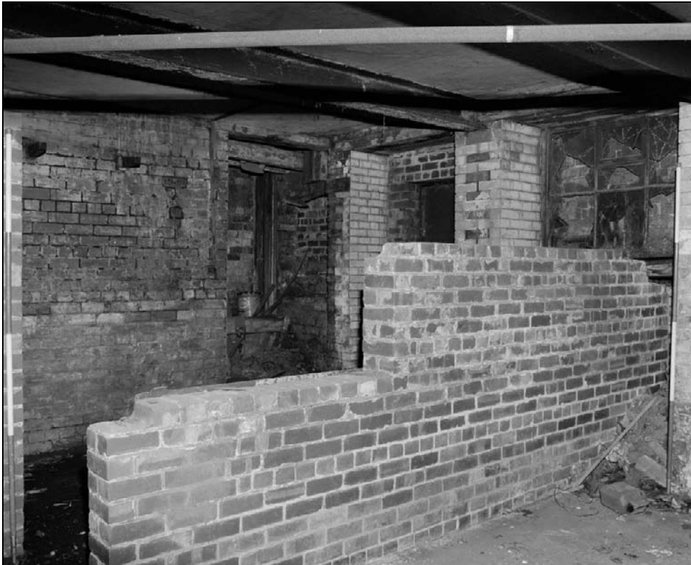
Plate 84: General view of room B3, west range – note inserted brick partitions and light reflecting brick piers (film 6.9)
