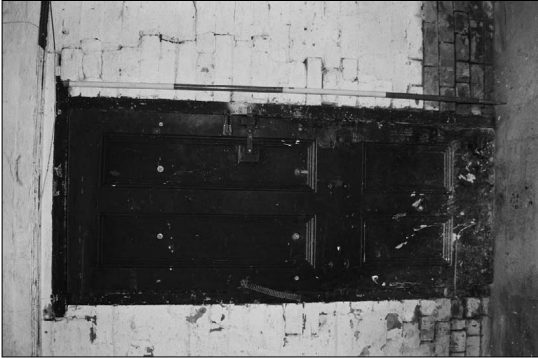
Plate 121: Detail of inserted doorway within former window leading from cart passage, G23 west range (film 3.6)
