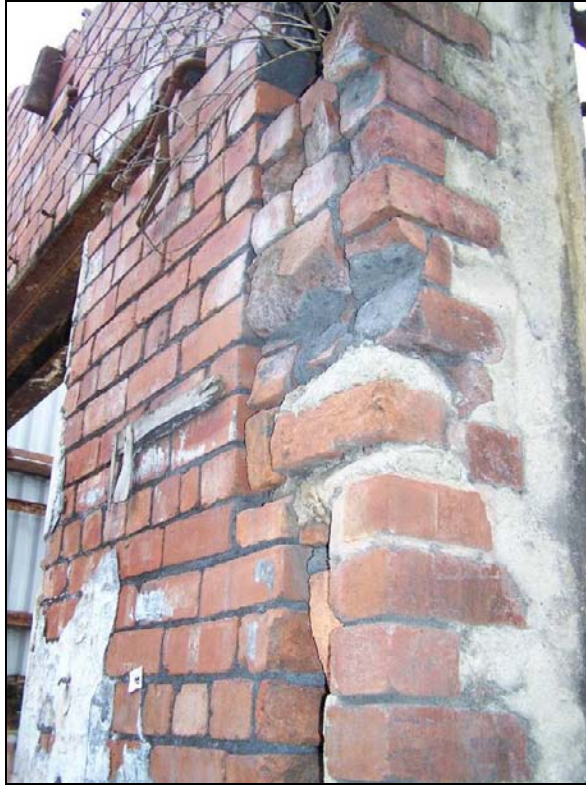
Plate 432: Detail of southeast corner of south elevation of furnace house showing remains of spring of segmental brick arched head of former doorway (film D.33)
