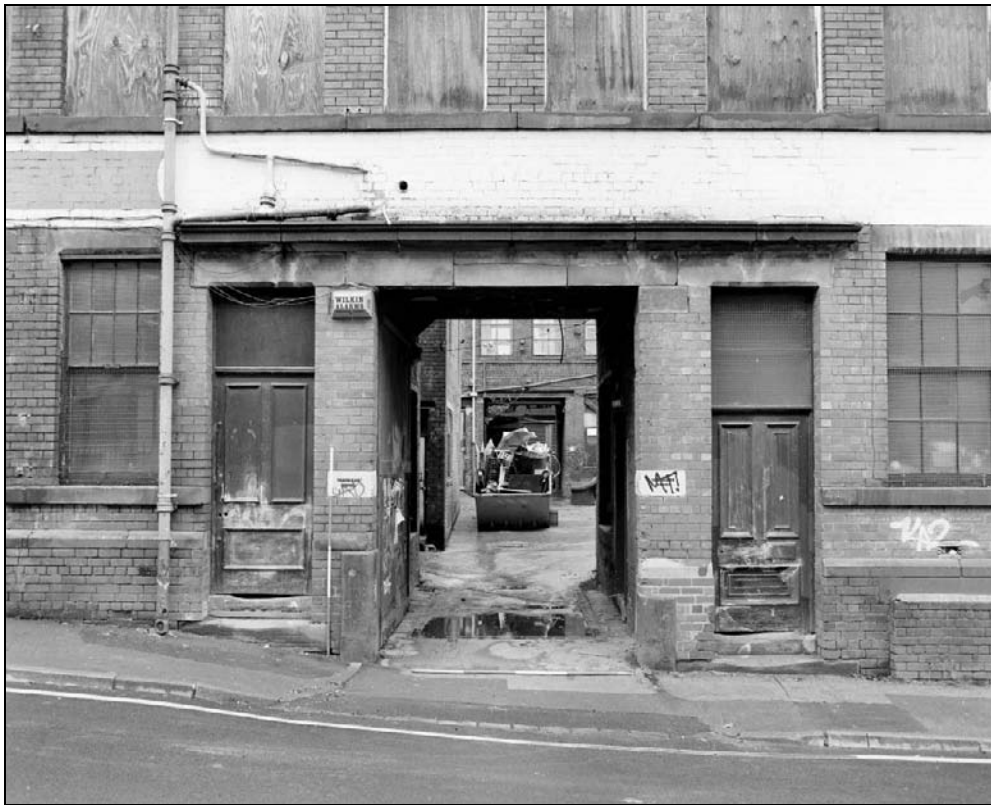
Plate 4: Detail of cart passage and flanking pedestrian doors, west elevation of west range (film 4.6)
