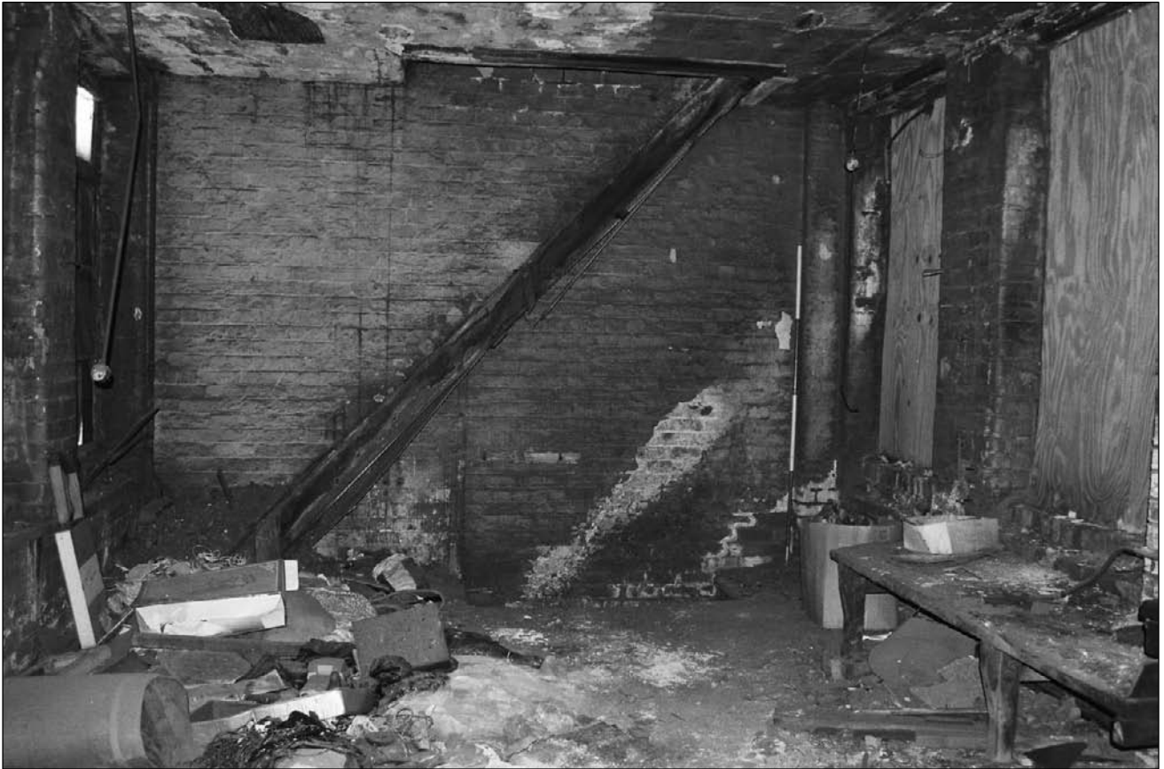
Plate 307: View of inserted staircase at east end of F8 – note brick flue in southeast corner of room (film 27.16)
