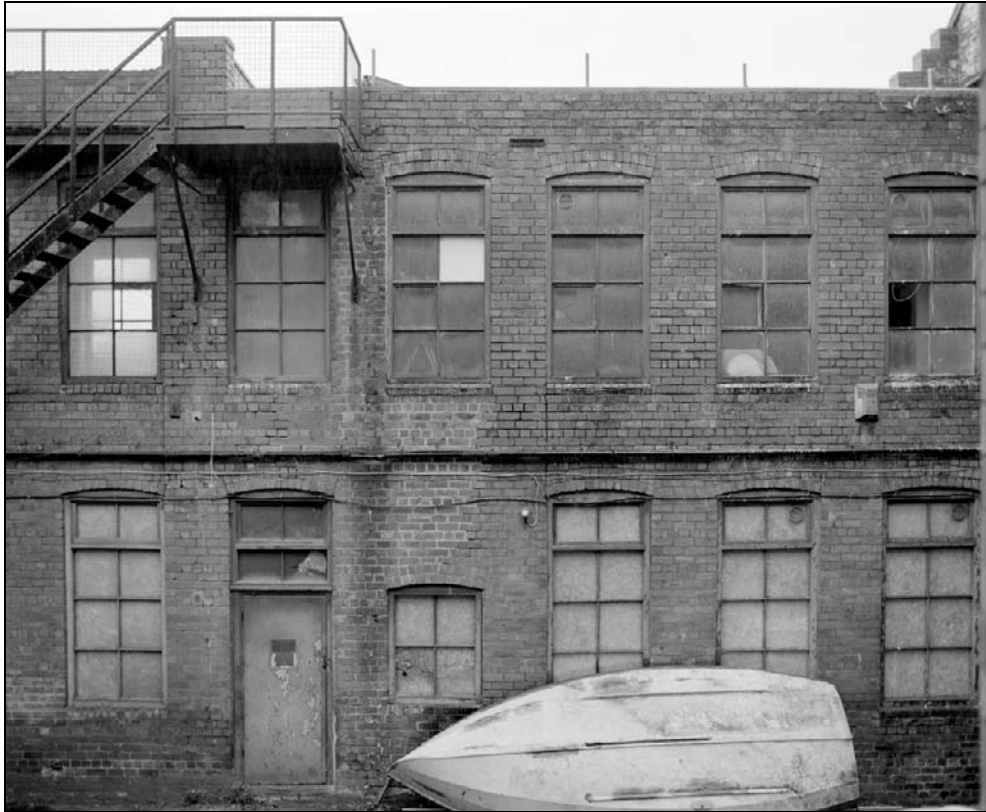
Plate 222: General view of north elevation of south range (west end) – note external staircase leading to 2 nd floor and inserted door within former window and inserted window in former door at ground floor (film 33.6)
