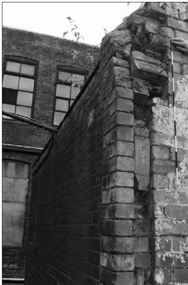
Plate 429: Detail of southwest corner of furnace house showing join with west building of the range and remains of spring of segmental brick arched head of former doorway in south elevation (film 23.3)
