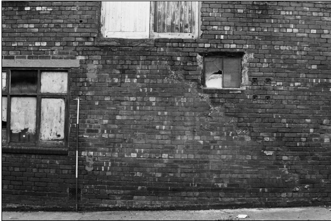
Plate 342: Detail of removed external staircase scar, south elevation of north range (film 28.24)
