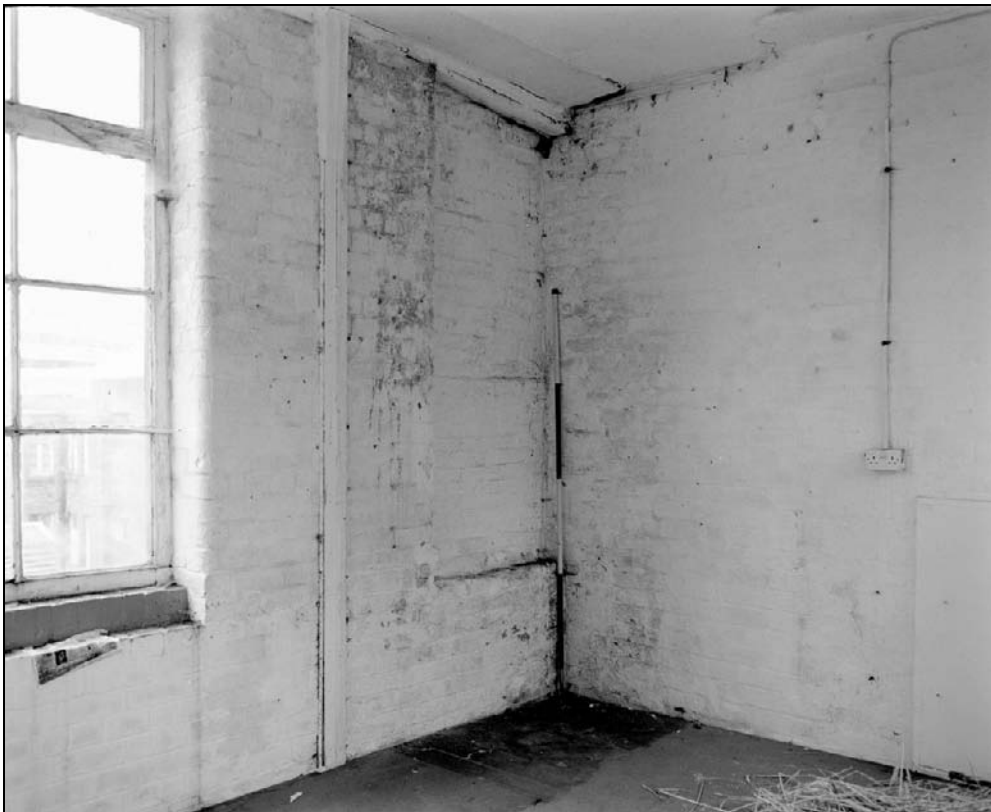
Plate 282: View of southwest corner of west end of F9 showing blocked opening (film 34.2)
