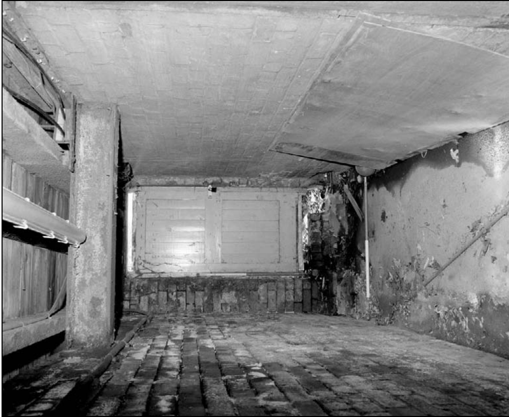
Plate 240: General view along B7 towards doorway leading to former rear yard of Trafalgar Grinding Wheel (film 8.8)
