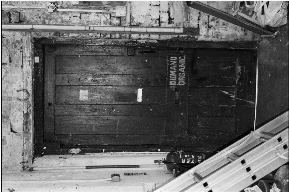
Plate 329: Detail of primary timber panelled door, west wall of F6, east range (film 26.10)
