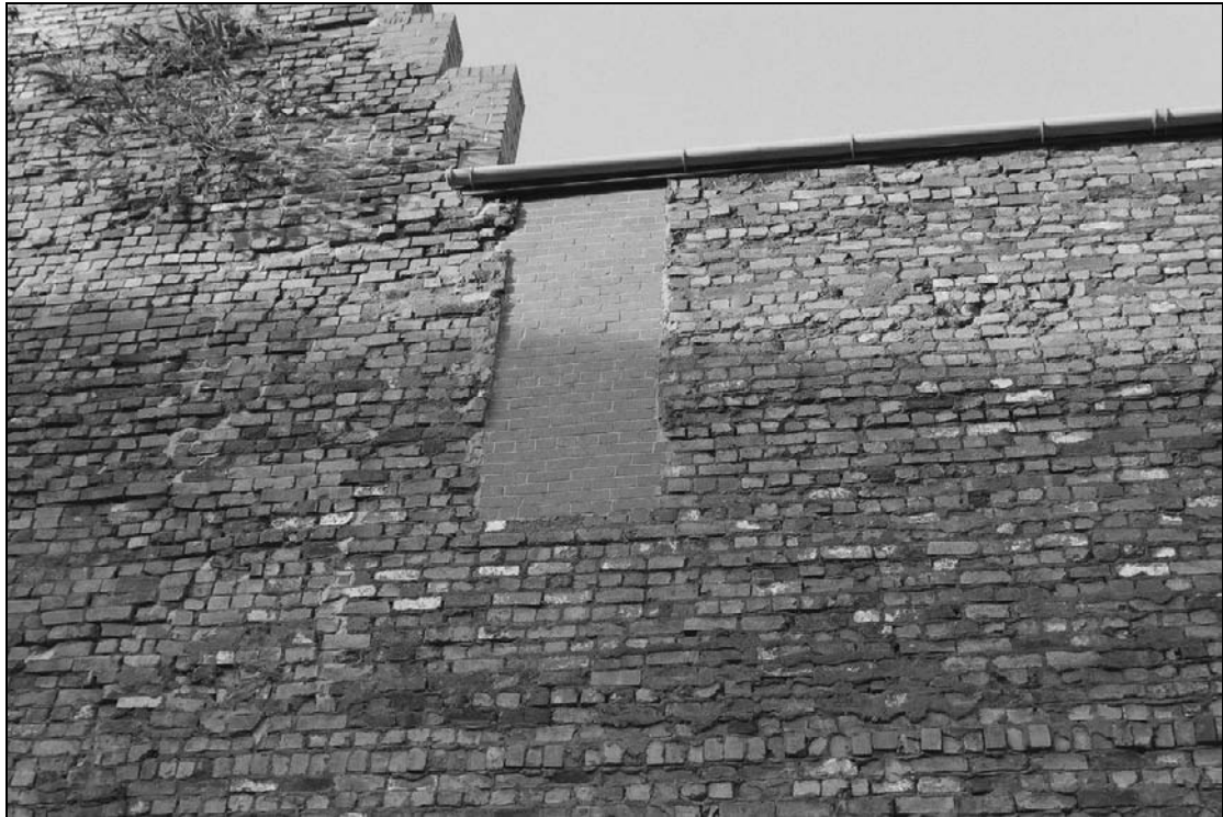
Plate 24: Detail of blocked opening, 1 st floor of south range, south elevation (film 46.25)
