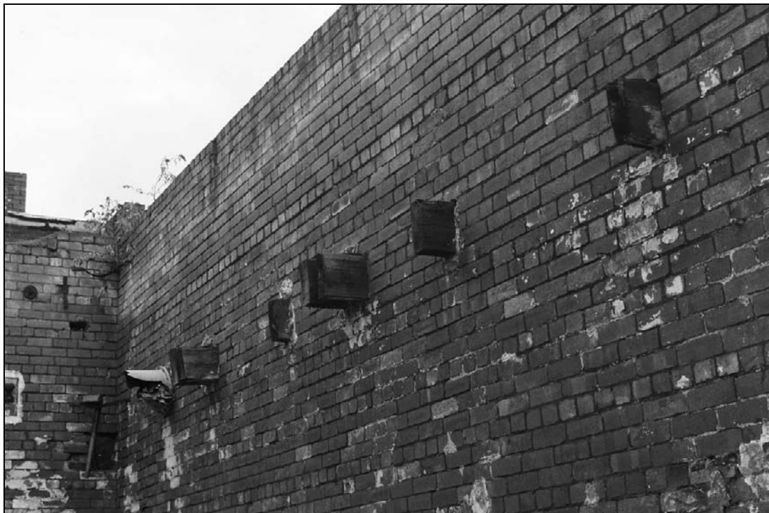
Plate 433: General view of truncated trusses, north wall of G11, furnace house (film 23.4)
