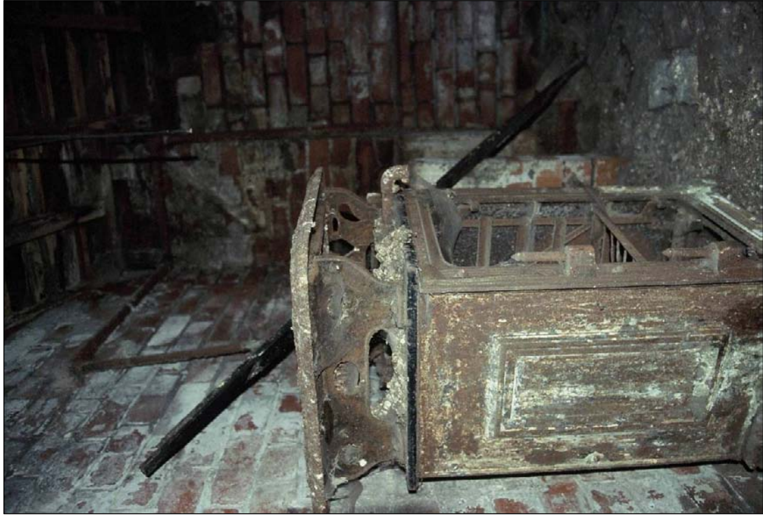
Plate 212: Detail of cast iron stove, S4 (film C/S 4.12)
