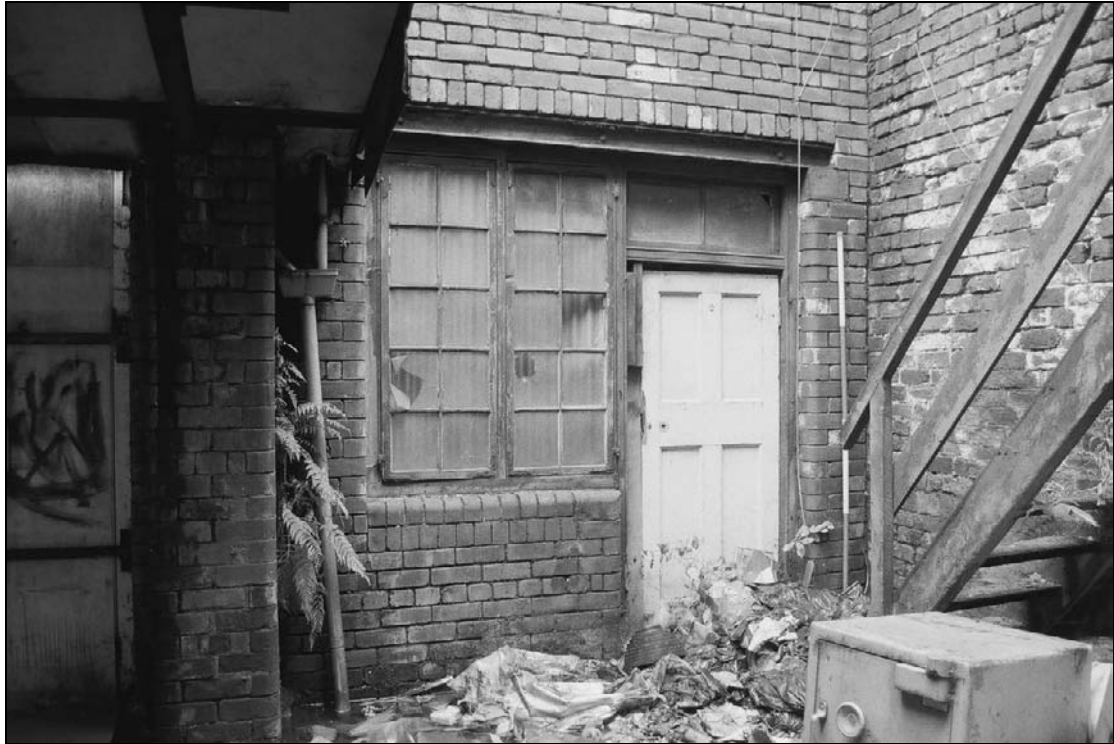
Plate 351: General view of entrance and window type 20 to G4, east elevation of north range (film 2.23)
