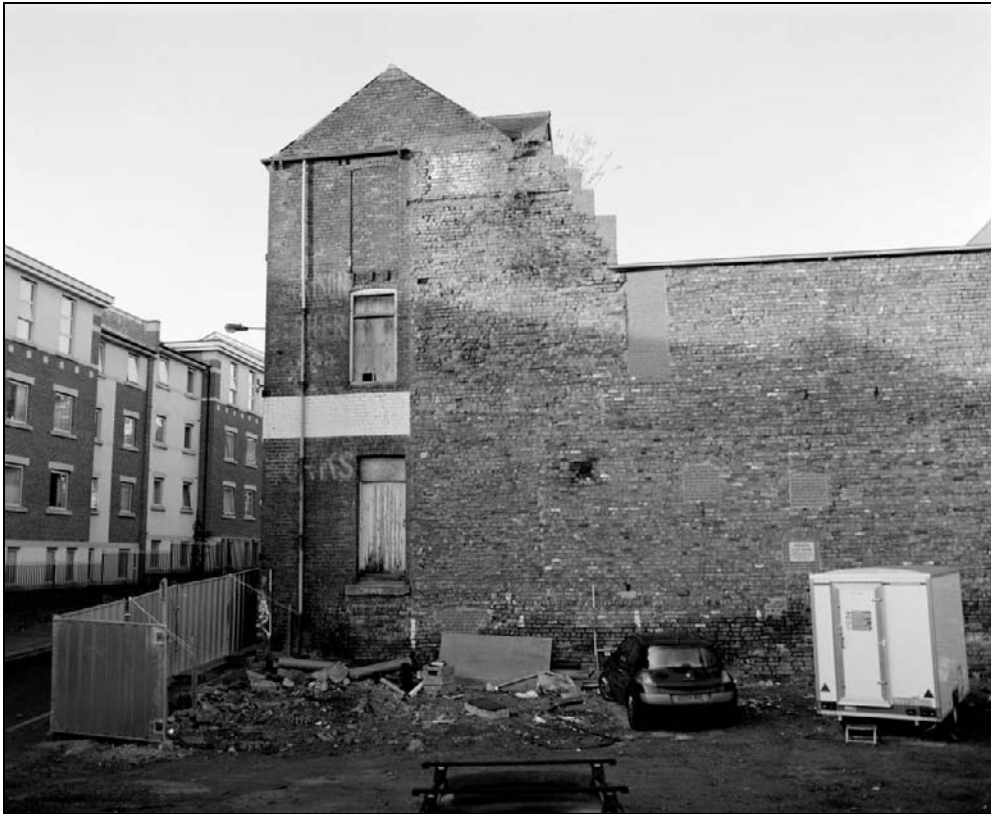
Plate 17: General view of south elevation of the west range and west end of the south range (film 47.1)
