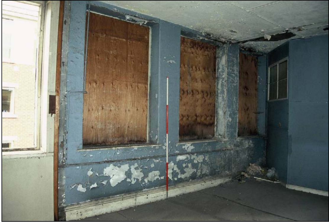
Plate 139: General view of F13 showing original skirting, inserted partitions and colour scheme (film C/S 2.3)
