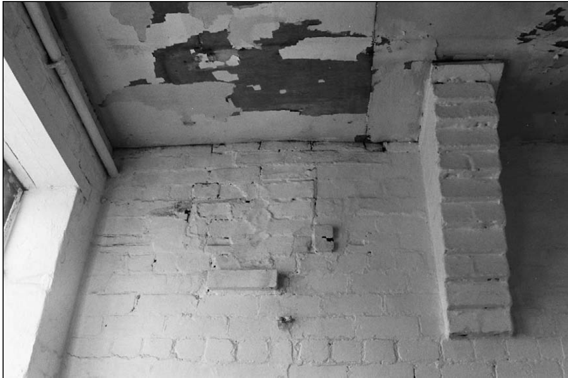
Plate 257: Detail of high blocking within west wall of G18, south range (east end) (film 22.17)
