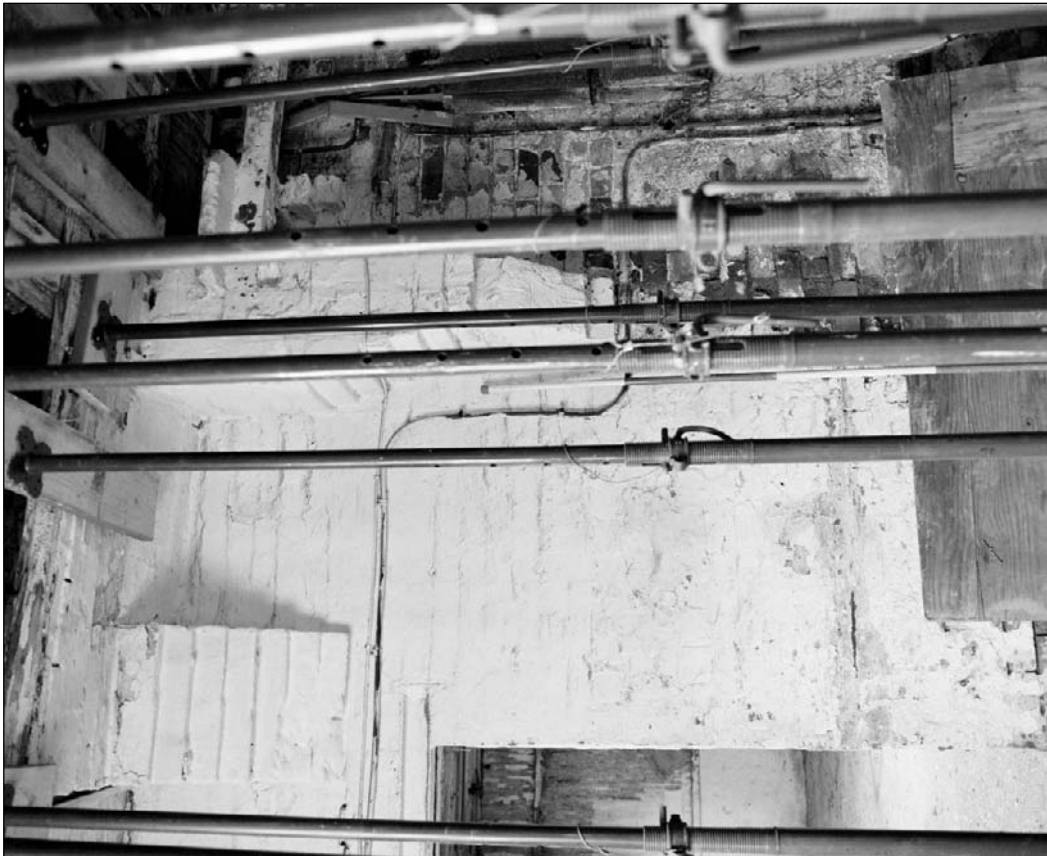
Plate 261: View of stepped brick supports for the chimney breast and fireplace on floor above, east wall of G17, south range (film 18.3)
