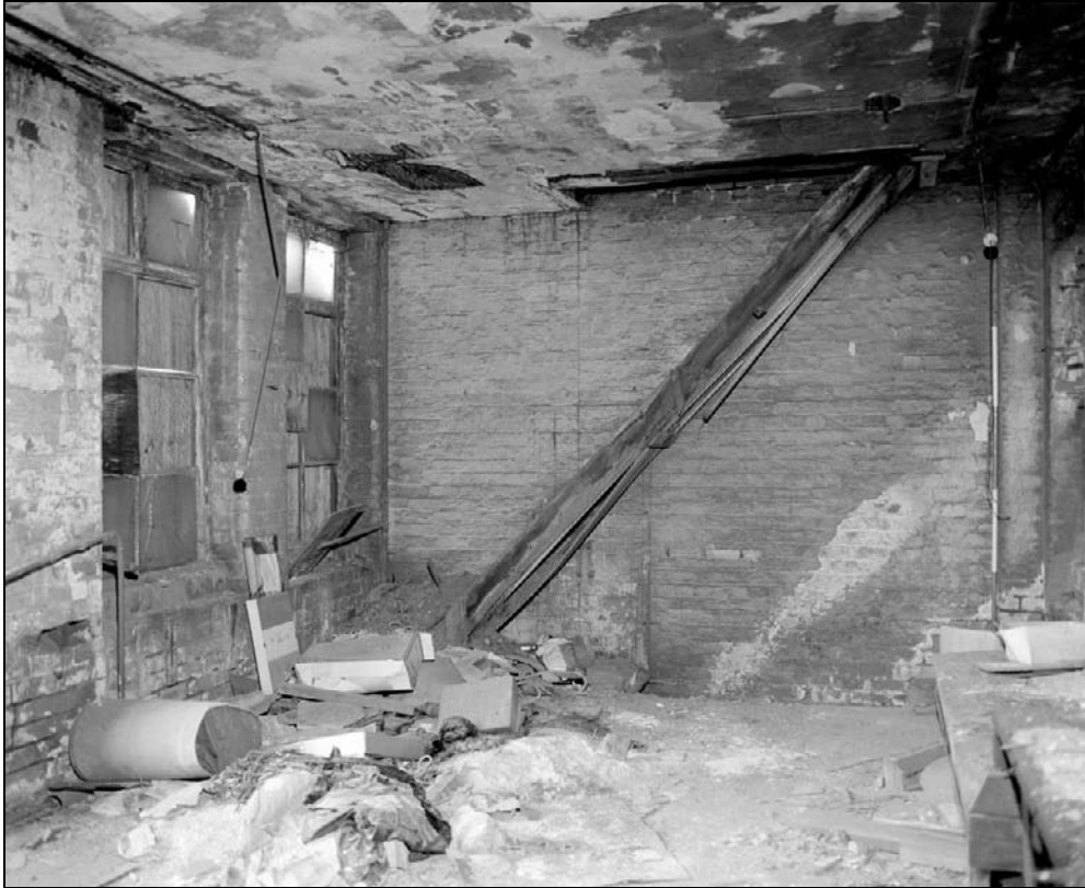
Plate 298: General view of F8, south range (east end) – note inserted staircase (film 35.4)
