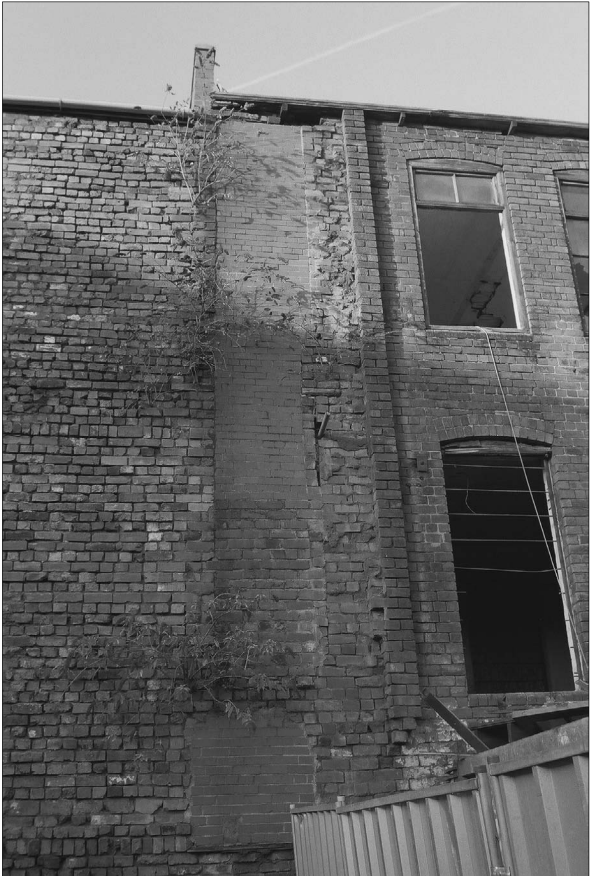
Plate 32: View of possible blocked power transmission shaft and projecting bricks denoting the eastern extent of the formerly adjacent Trafalgar Grinding Wheel and extensions, south elevation of the south range (film 46.20)
