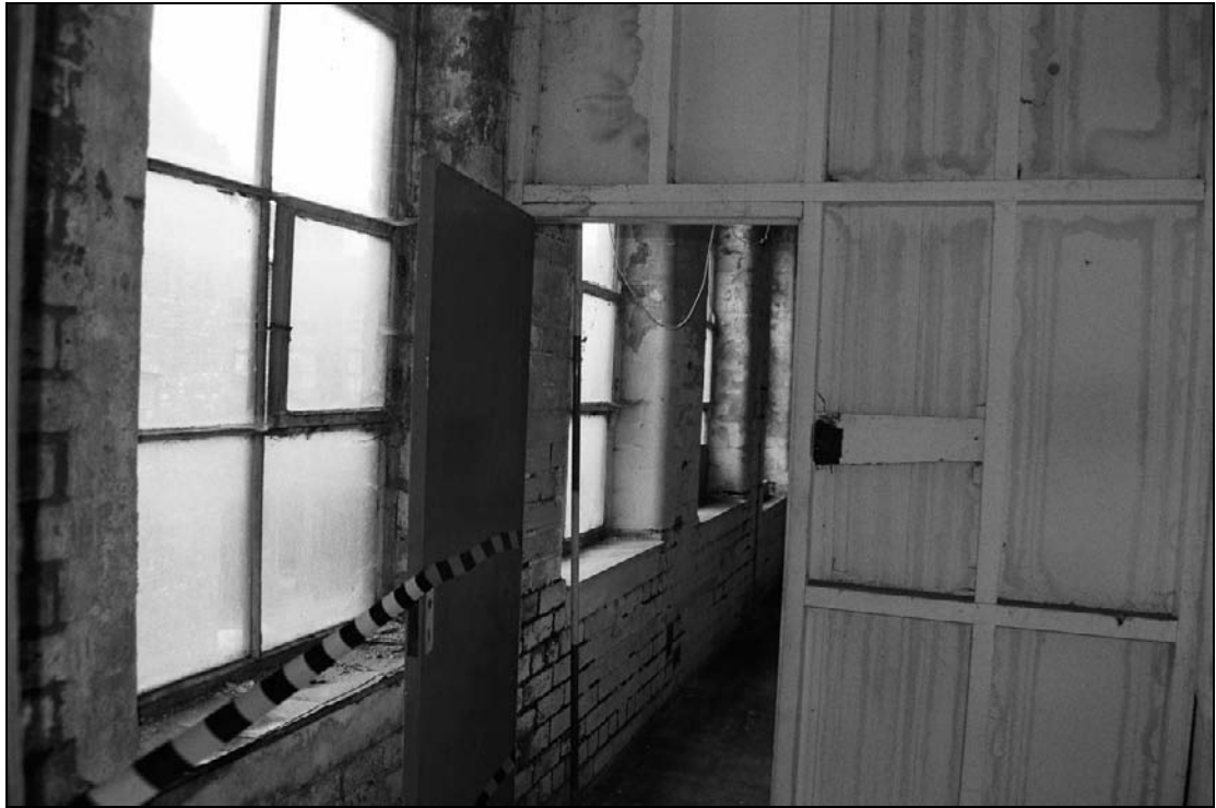
Plate 275: View of modern studwork partition at west end of F10, south range (film 25.8)
