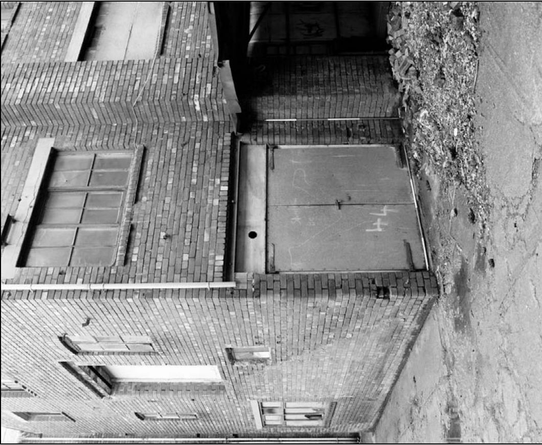
Plate 347: Detail of secondary inserted modern door and type 14 window, southeast corner of north range (film 10.4)
