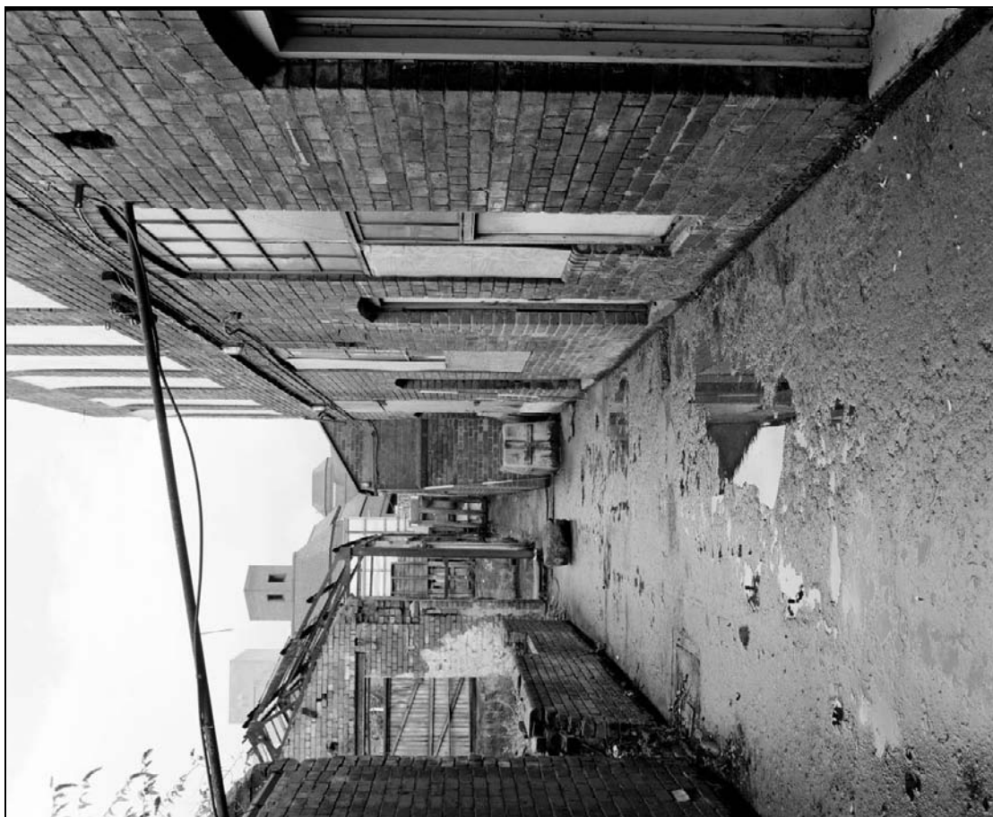
Plate 227: View of rear yard showing south range (east end) to the right, furnace house range to the left (film 10.7)
