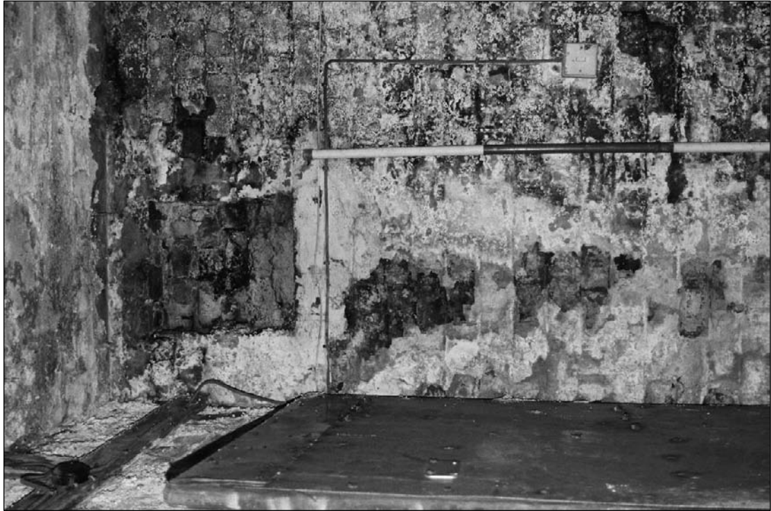
Plate 384: Detail of blocked wall box, north wall of F4, north range (film 24.34)
