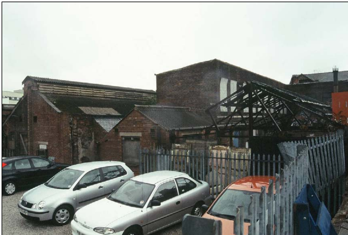
Plate 58: General view of the east elevation of the machine shop, wash house and furnace house ranges, with the south range beyond (film C/S 2.30)
