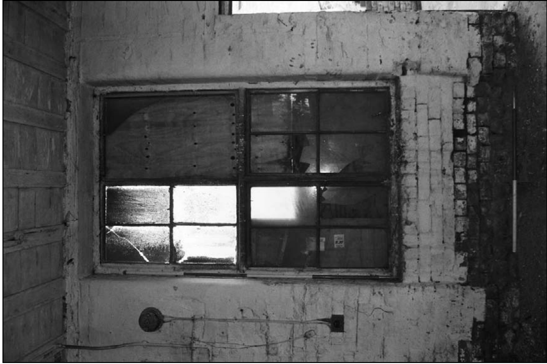
Plate 268: Internal detail of type 7 window, north wall of G16, south range (film 22.3)
