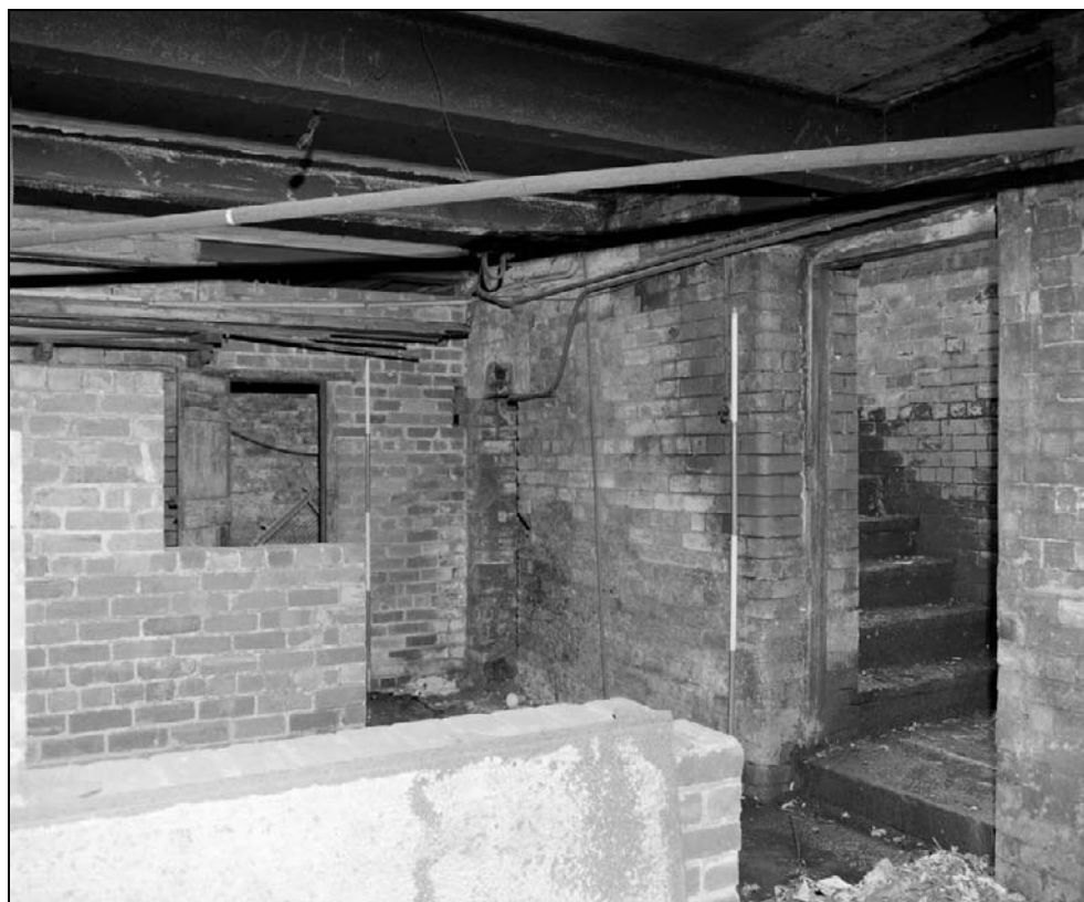
Plate 85: General view of room B3, west range – note steel I-section beams supporting the concrete floor above (film 7.2)
