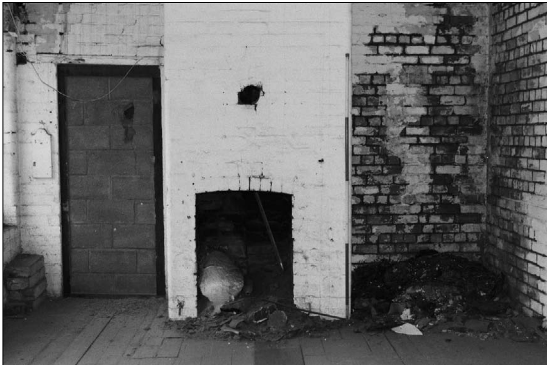
Plate 278: Detail of fireplace and blocked doorway, east wall of F10, south range (film 25.2)
