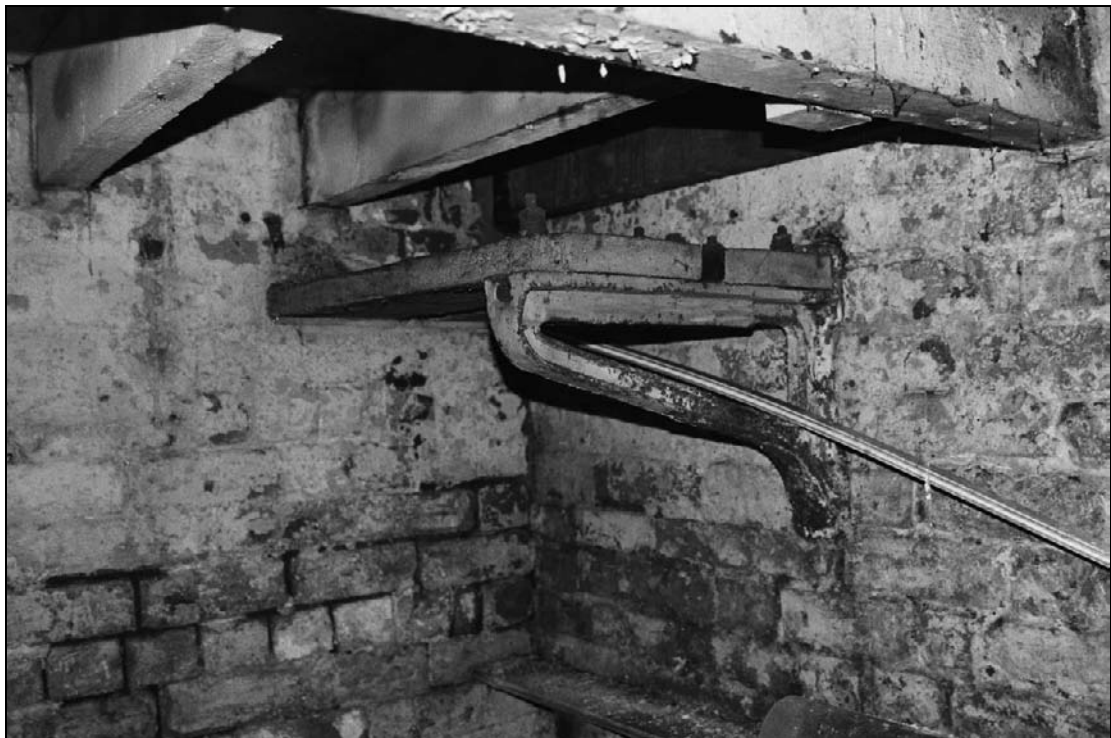
Plate 119: Detail of cast iron bracket, north wall of G3, west range extension (film 21.2)
