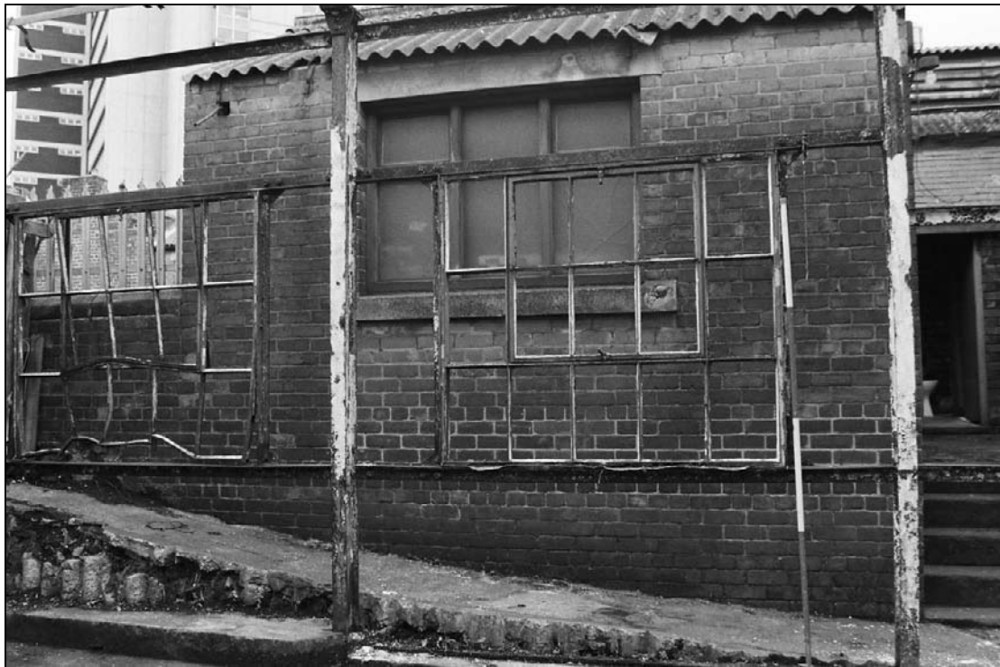
Plate 441: Detail of metal framed type 24 window and steel framed structure, south wall of G12, east building of furnace house range – note north elevation of G13, wash house beyond (film 23.13)
