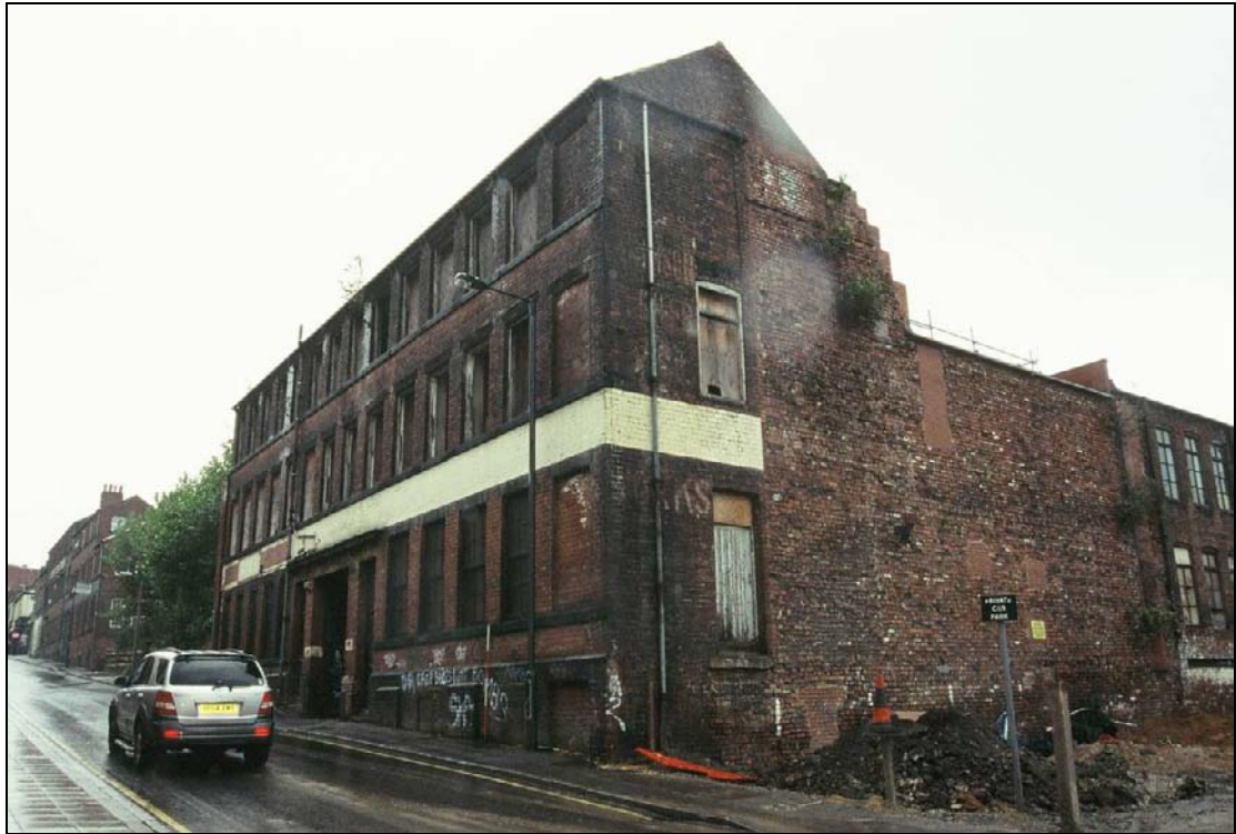
Plate 15: General view of the principal façade (west elevation) and south elevation of Trafalgar Works, fronting Trafalgar Street (film C/S 2.35)
