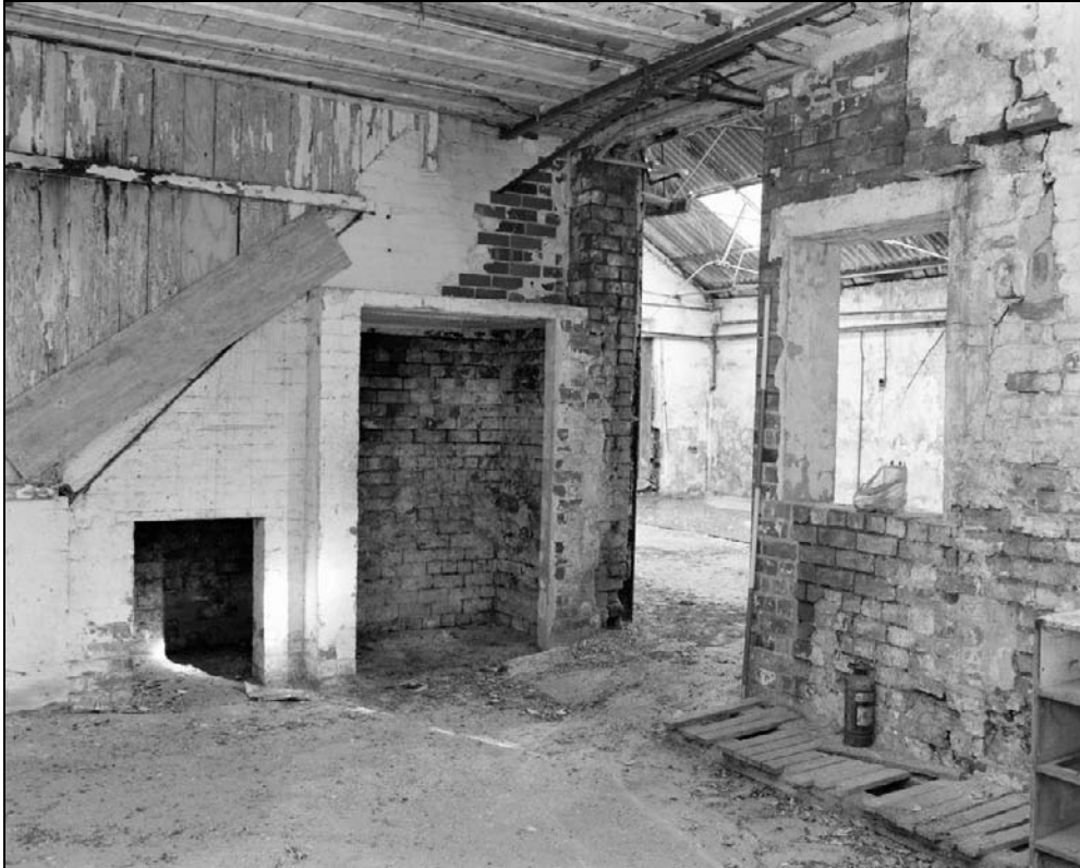
Plate 265: General view of southeast corner of G16, south range with G15, machine shop beyond – note inserted doorway in former window, inserted window and removed hand forge (film 18.8)
