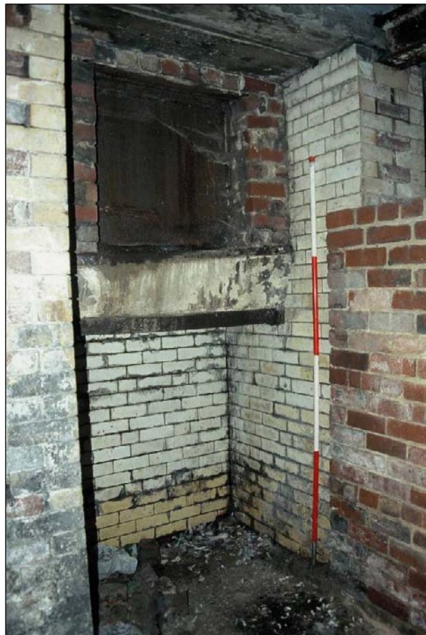
Plate 89: Detail of altered lightwell to coal chute, B3, west range (film C/S 2.26)
