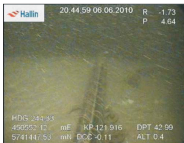
Plate 21: Chain under cable
