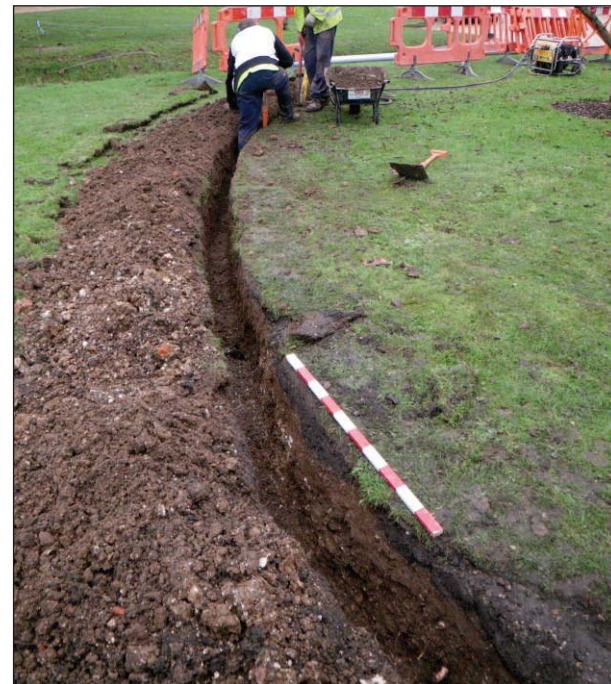
Plate 5: BT Data Cable viewed from north-east
