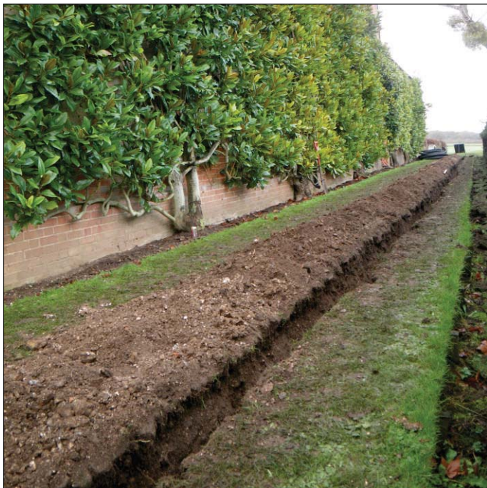
Plate 4: BT Data Cable viewed from south-east
