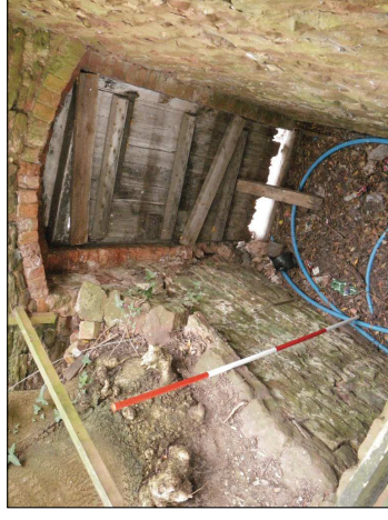
Plate 8: The internal side of the north-eastern gate depicted in Plate 7. Note the depth of made ground against the internal side of the precinct wall (note 2m scale).
