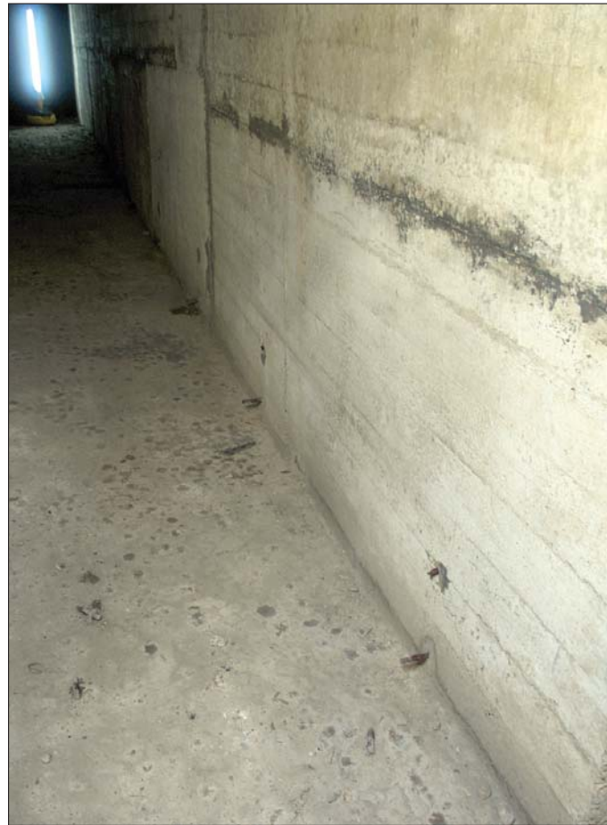
Plate 8: Studs along west wall of Tr 2b, former bench supports. Looking south-west.
