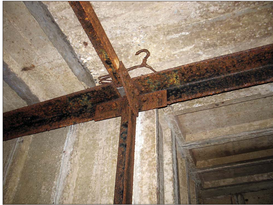
Plate 13: Coat hangers behind girder. Tr 1b. Looking north-east.
