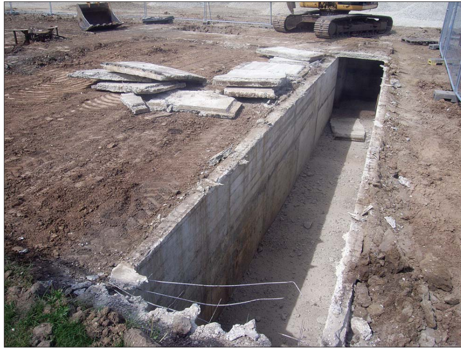
Plate 14: View along Tr2c showing exposed concrete and wire frame during demolition. Looking north.
