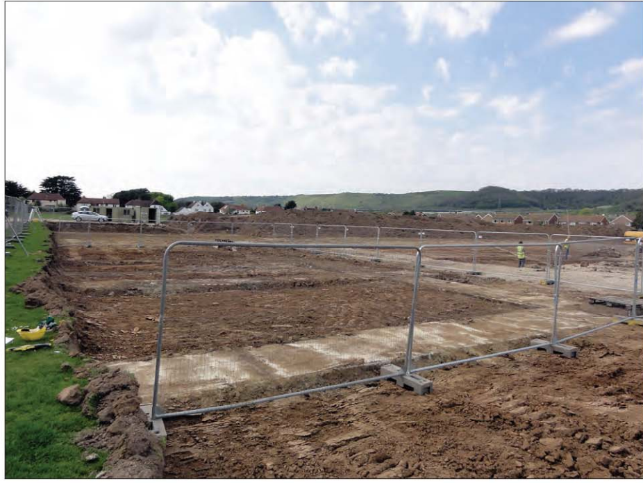
Plate 1: View across the exposed roof of the air raid shelter following top soil stripping. Looking West.
